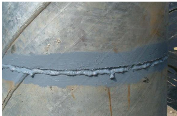
Unacceptable weld (overlap at the bottom of the weld, undercut/under fill at the top)
