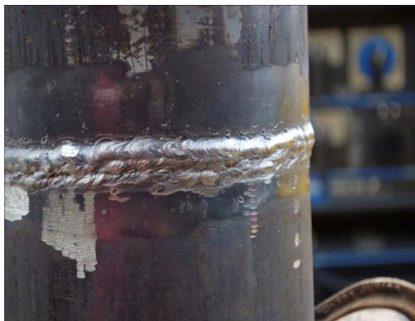
Unacceptable weld (overlap at the bottom of the weld, undercut/under fill at the top) Acceptable weld (arc strikes removed by grinding)
