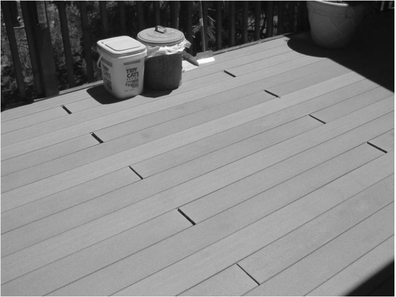
15.2 Shrinkage of WPC boards on a deck.
