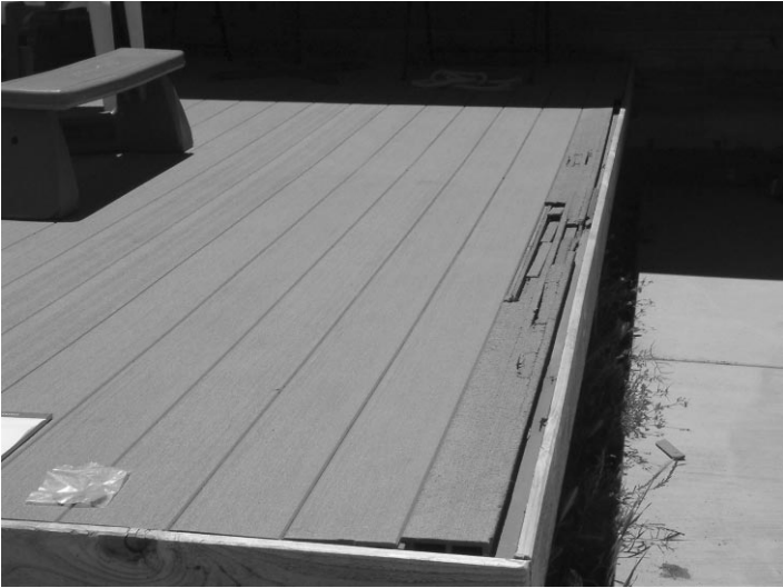
15.5 An advanced step of crumbling of a WPC deck board (Arizona).
