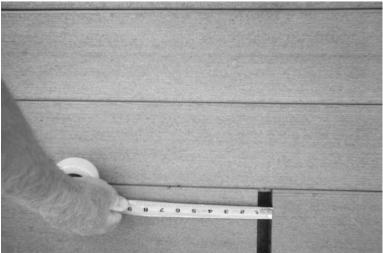
15.1 A 1-inch (25 mm) gap due to shrinkage of composite deck boards on a deck.
