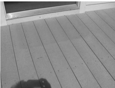
15.7 Fading of a composite deck. The ‘Welcome’ mat has just been removed.
