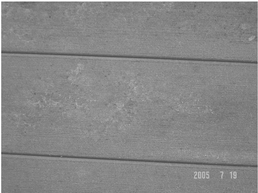
15.3 Mold on composite deck boards.
