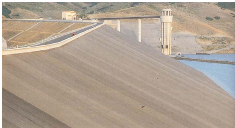
Fig. 84. The MONTE COTUGNO embankment dam on the Sinni River near Potenza, Italy [46]
