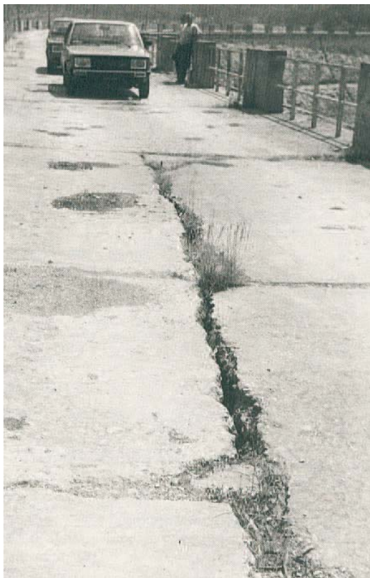
Fig. 110. Longitudinal cracks at the crest of the old DISUERI dry masonry dam after 50 years of service [35]
