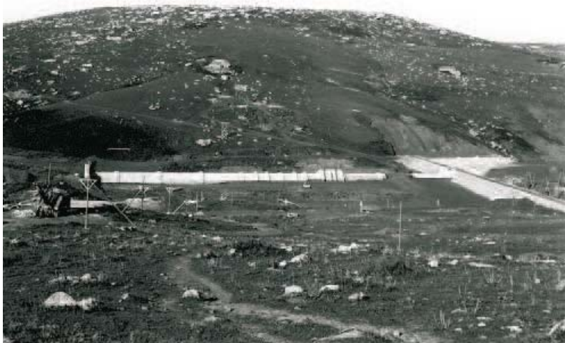
Fig. 116. The TRINITA' embankment dam under construction on the Delia River in Sicily in 1955. The outlet culvert crosses the dam foundation; one can note the reliefs at the extrados in order to improve contact of the concrete with the embankment core material [6] (photo by R. Jappelli, 1955)
