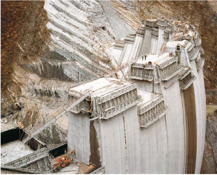
Fig. 112. The RIDRACOLI double curvature arch dam ( H = 100\text{ m} ) on the Bidente River in Romagna, under construction (L'Acquedotto della Romagna, 1991)
