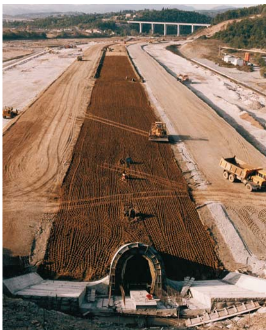
Fig. 89. The BILANCINO dam on the Sieve River near Florence: work in progress
