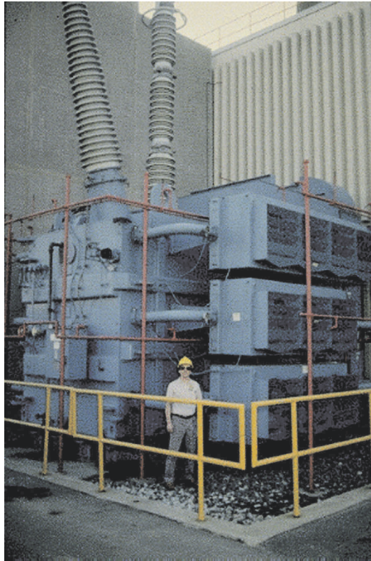
Figure 3.4 - This transformer in the Delaware River nuclear center plant in New Jersey was damaged by the magnetic storm of March 13 th 1989
