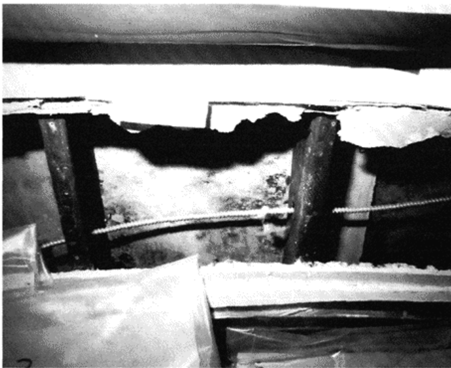
Fig. 4. Fungal growth on the internal surface of exterior gypsum board sheathing of an envelope wall. Gypsum board on the interior side of metal studs has been cut away revealing the growth within the wall cavity. Rainwater which wet the exterior sheathing could not evaporate to the outside because of a thick layer of rigid plastic insulation in the exterior part of the envelope.
