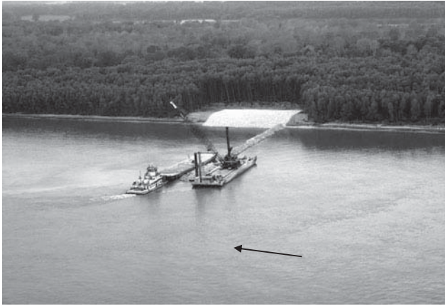
Fig. 5-8. Dike bank paving on the lower Mississippi River Source: USACE Vicksburg District
