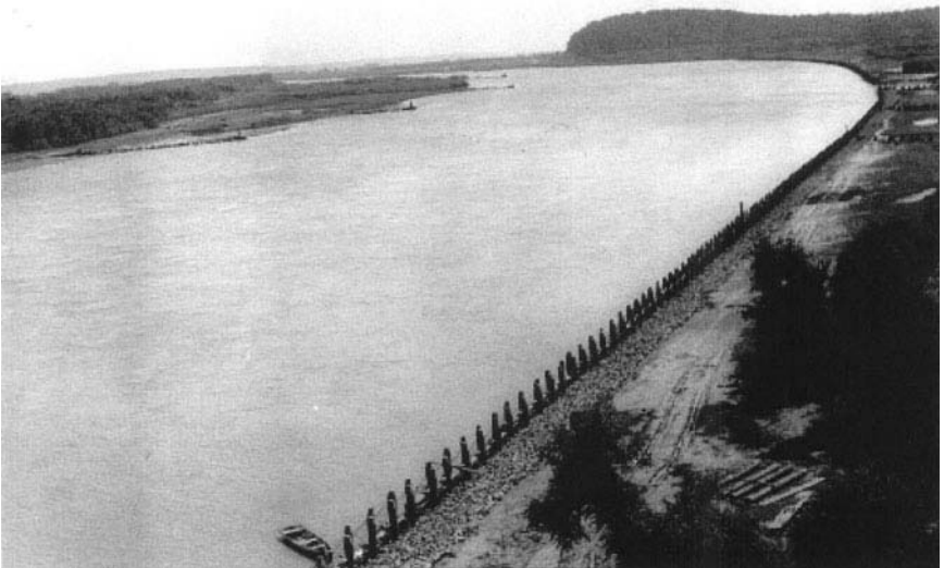
Fig. 5-22. Rock Bluff Bend, Missouri River, longitudinal stone-filled timber-pile dike added and timber-pile dikes on opposite point bar, September 1942
