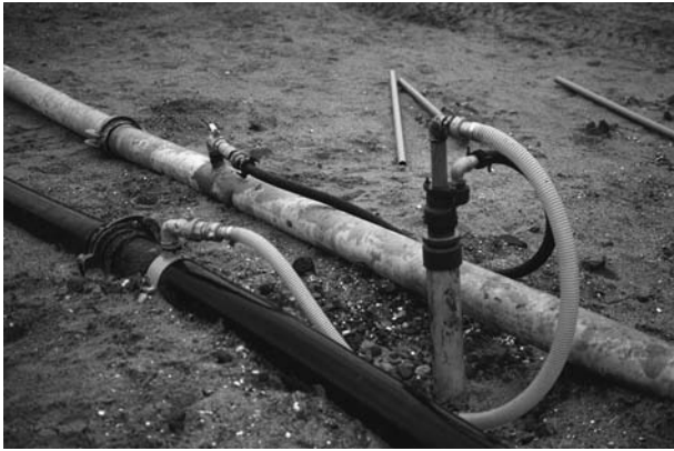
Figure 11.6 Ejector pipework. An ejector headworks is shown fitted to the well. The supply and return header pipes can be seen either side of the ejector well, linked to the ejector by flexible hoses. (Courtesy of WJ Groundwater Limited, Bushey, U.K.)
