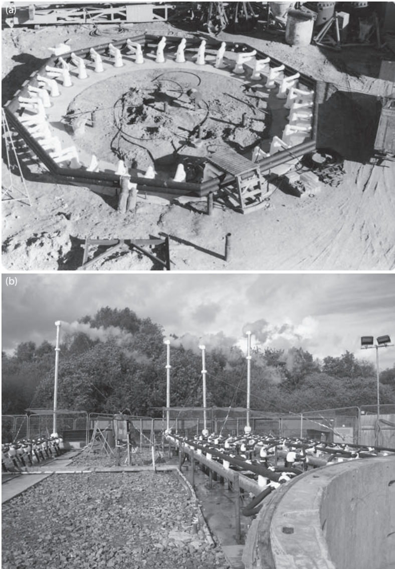
Figure 12.25 Typical layouts of artificial ground freezing systems. (a) Artificial ground freezing system (using brine as the refrigerant) prepared ready for sinking of a circular shaft. (b) Artificial ground freezing system (using LN as the refrigerant) as part of the recovery works on a tunnel project. The white plumes are water vapor caused by the low temperatures of the nitrogen gas exhausted to the atmosphere from the four towers visible in the background. (Courtesy of the British Drilling and Freezing Company Limited, Nottingham, U.K.)
