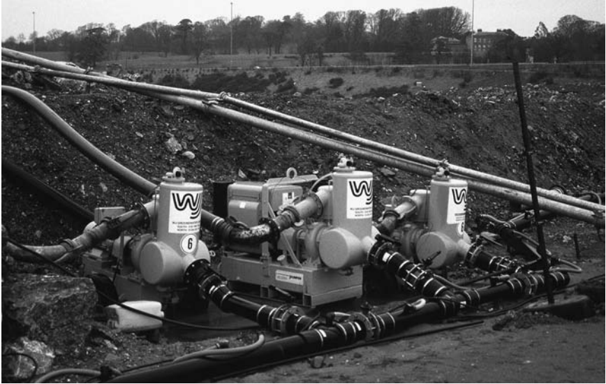
Figure 9.4 Wellpoint pumps connected to header main. The set of three wellpoint pumps is connected to the header main, with valves to isolate each pump. The center pump is a standby pump to be used if either of the other pumps is out of service. (Courtesy of WJ Groundwater Limited, Bushey, U.K.)
