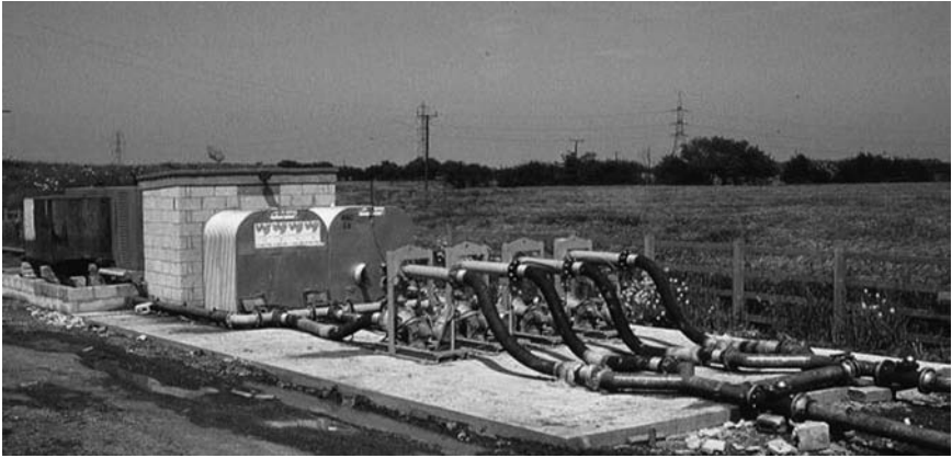
Figure 11.25 Booster pumps use to drive water from dewatering system along transfer pipeline to recharge wellfield. (Courtesy of WJ Groundwater Limited, Bushey, U.K.)
