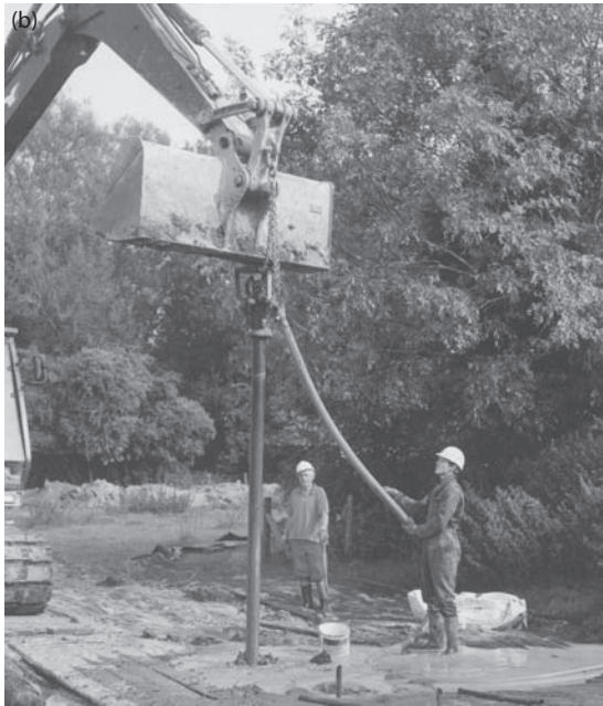
Figure 9.9 Installation of wellpoints using placing tube. (a) Steel placing tube is suspended from the excavator; (b) placing tube is jettied into the ground.
