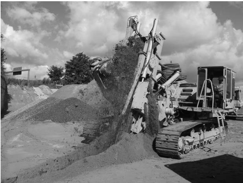
Figure 11.10 Trenching machine cutting trench and laying horizontal drains. (Courtesy of Holscher Wasserbau GmbH, Haren, Germany.)
