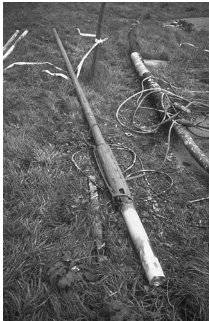
Figure 16.4 Biofouling of submersible pump due to iron-related bacteria. The submersible pump and riser pipe shown have been removed from a dewatering well after several weeks of operation. The upper part of the pump is coated with a thick red-brown biofilm slime.
