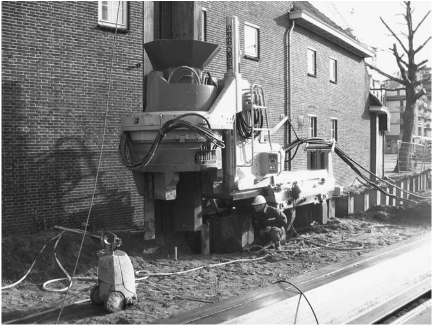
Figure 12.4 Installation of steel sheet piling by the press-in method using hydraulic jacks. The hydraulic jacking unit sits on top of the previously driven piles. The jacking unit grips onto the piles and presses new piles into the ground using the resistance of the neighboring piles. (Courtesy of Giken Europe BV, London.)
