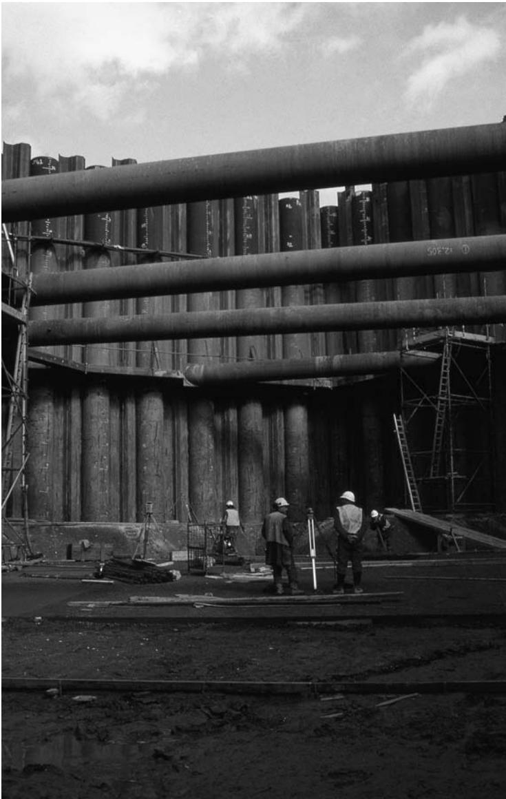
Figure 12.5 Combi-pile walls. The wall comprises primary elements (large-diameter tubular steel piles) and secondary elements (steel sheet piles) that are linked together by clutches.
