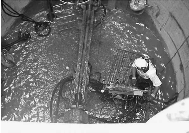
Figure 14.6 Installation of lateral wells by rotary drilling from within collector well shafts. Sump pumps are used to control the water from the drilling flush. (Courtesy of Strathclyde Partnership for Transport, Glasgow, U.K., and Keller Geotechnique, Wetherby, U.K.)
