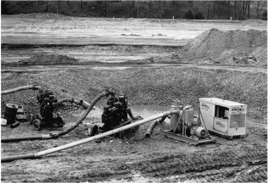
Figure 8.7 Dee Reservoir, central pumping sump. The sump pumps are composed of one electrically powered unit, supplied from a portable generator, and two diesel-powered units. (Courtesy of the Grampian Regional Council, Aberdeen, U.K.)
