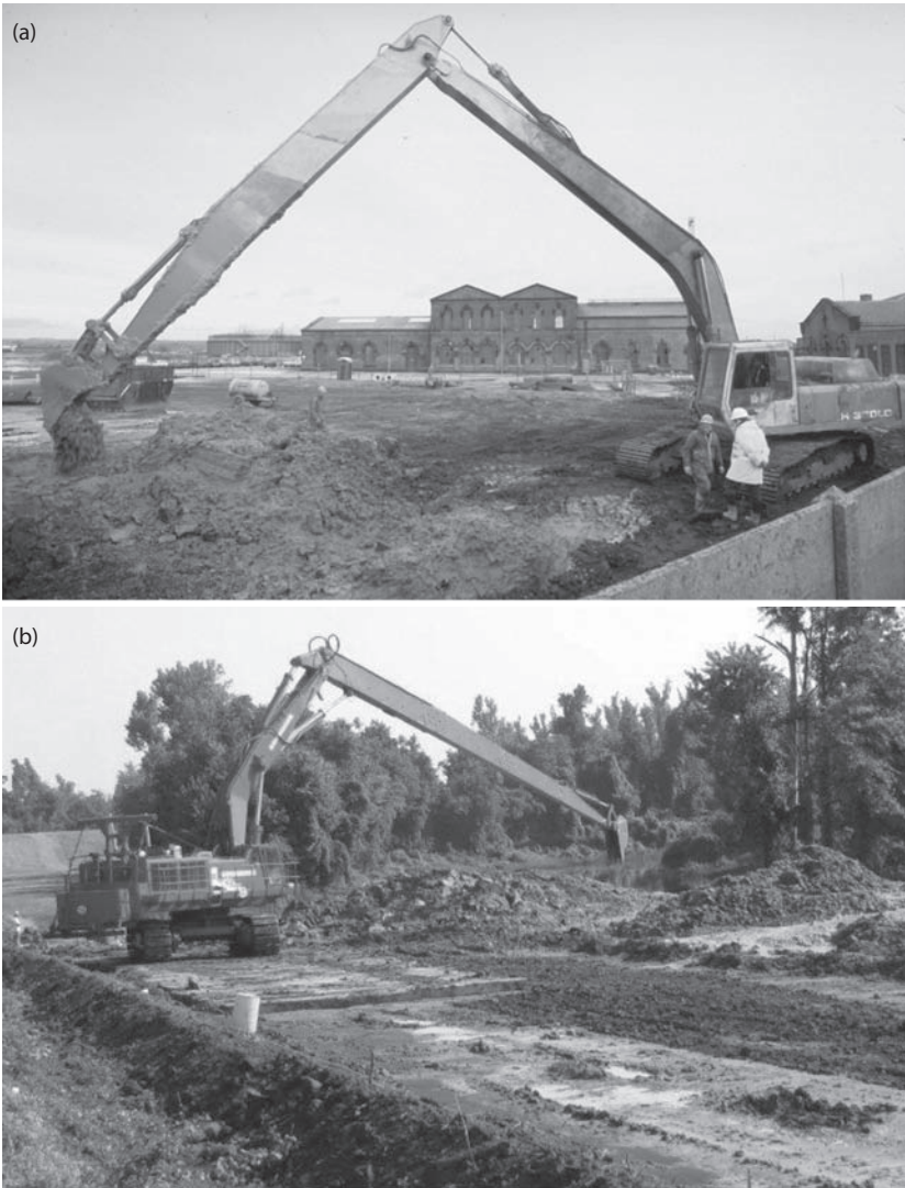
Figure 12.7 Construction slurry trench wall by backactor. (a) Excavation by conventional backactor fitted with extended boom and dipper arm. (Courtesy of Arup, London.) (b) Excavation by specialist long-reach backactor. (Courtesy of Inquip Associates, Inc., Santa Barbara, CA.)
