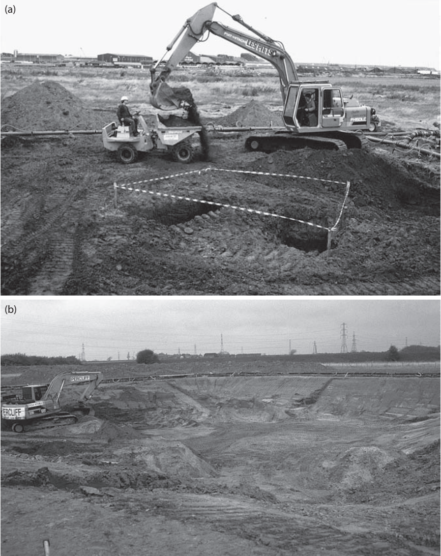
Figure 6.18 Wellpoint dewatering trials. (a) Ring of wellpoints installed around trial area. A 20 \times 20 m rectangular ring of wellpoints was installed around the trial area. Local excavations were made within the dewatered area to assess the behavior of the dewatered soil when excavated. (b) Battered excavation inside the wellpoint ring, with sides at various trial slope angles. A trial excavation was made within a 40 \times 40 m rectangular ring of wellpoints in silty sand. Trial batter slopes were formed to assess the stability of the soil after groundwater lowering. (Courtesy of WJ Groundwater Limited, Bushey, U.K.)
