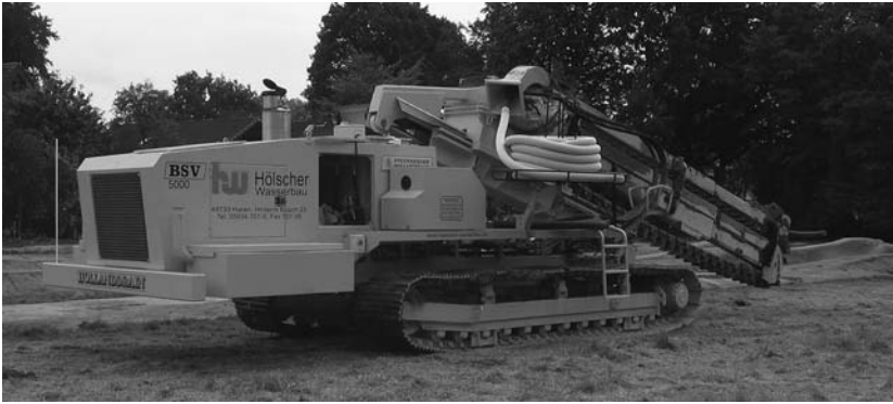
Figure 11.9 Specialist trenching machine for installation of horizontal drains. (Courtesy of Holscher Wasserbau GmbH, Haren, Germany.)
