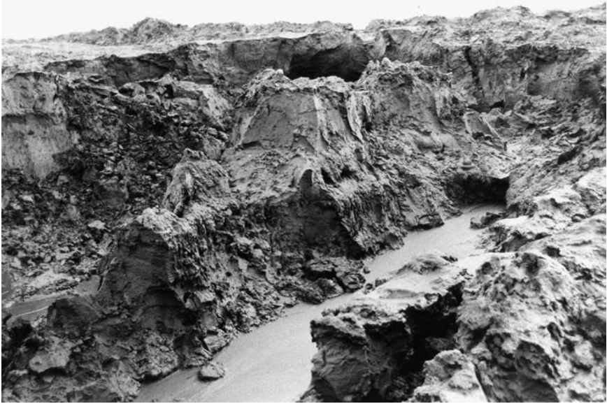
Figure 9.19 Initial excavation (showing unstable conditions) for Derwent outlet channel. (Courtesy of Northumbrian Water Limited, Durham, U.K.)
