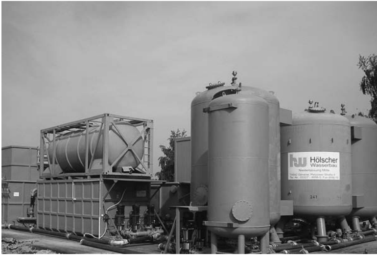
Figure 11.27 Modular groundwater treatment plant used to treat discharge from dewatering system. (Courtesy of Hölscher Wasserbau GmbH, Haren, Germany.)
