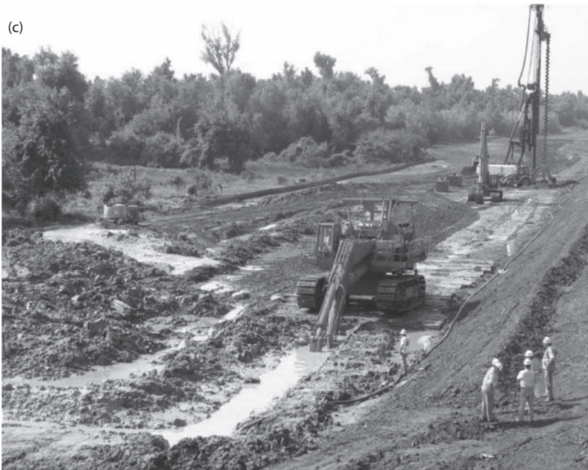
Figure 12.7 (Continued) (c) Trench kept topped up with bentonite slurry during excavation. (Courtesy of Inquip Associates, Inc., Santa Barbara, CA.)
