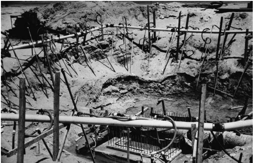
Figure 8.5 Significant ground movement caused by inappropriate sump pumping. The wellpoint risers around the perimeter of the excavation had originally been installed vertically. Loss of fines due to poorly controlled sump pumping resulted in ground movements, distorting the wellpoints from the vertical.
