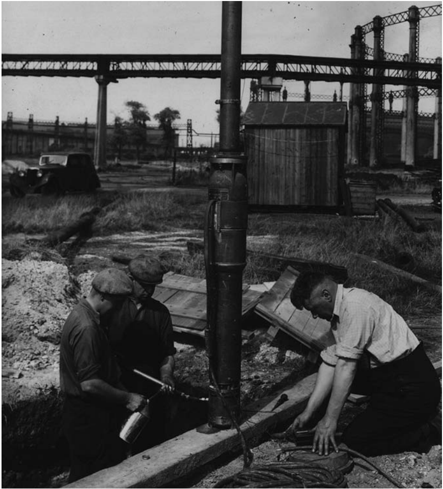
Figure 2.4 Early application of deep wells in Britain. A submersible pump is being prepared for installation into a well on-site in the 1940s.
