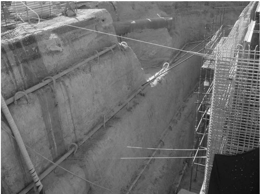
Figure 9.16 Four-stage wellpoint system. The sand being dewatered is slightly cemented, which allows the side slopes to stand very steeply in the short term. The cementing is sufficiently weak that the ground unravels in the event of water inflow but in a “dewatered” state can stand almost vertically. (Courtesy of WJ Groundwater Limited, Bushey, U.K.)
