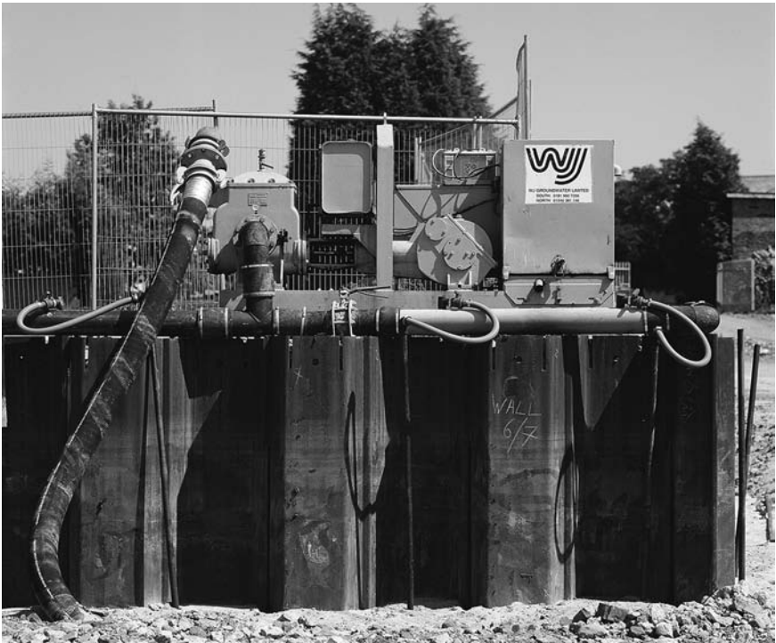
Figure 13.1 Reciprocating piston pump set used for wellpointing. (Courtesy of WJ Groundwater Limited, Bushey, U.K.)
