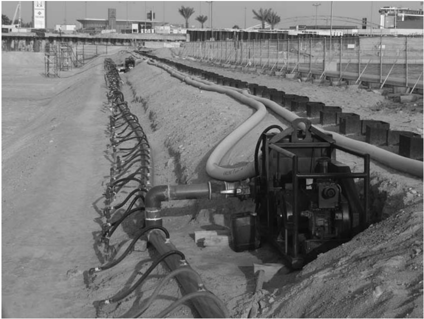
Figure 9.5 Wellpoint header main installed below the original ground level. Before dewatering, local excavations were made down to the natural groundwater level along the line of wellpoints, and the header main and pumps were installed at that level. (Courtesy of WJ Groundwater Limited, Bushey, U.K.)
