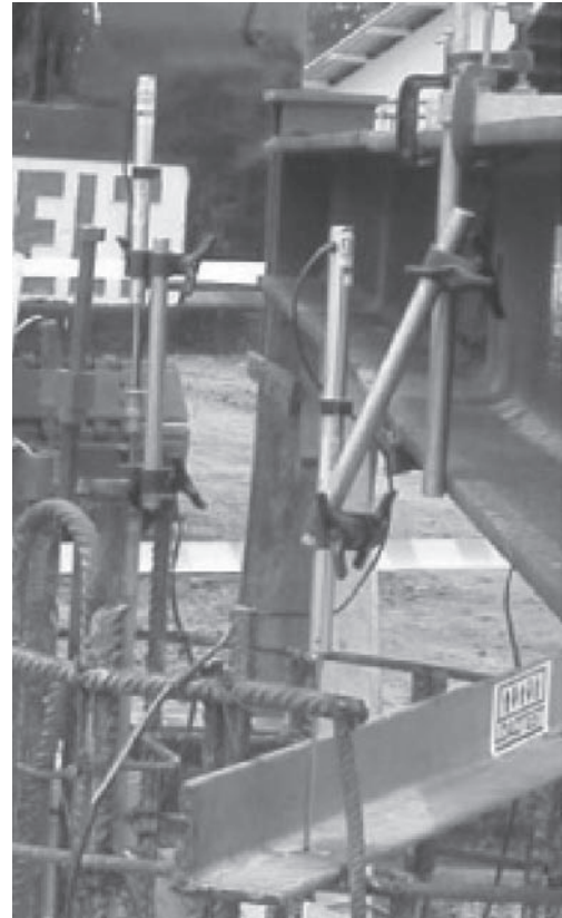
Figure 5. Two LVDTs: one monitoring the top of pile from the reference beam and the pile compression above the O-cell.
