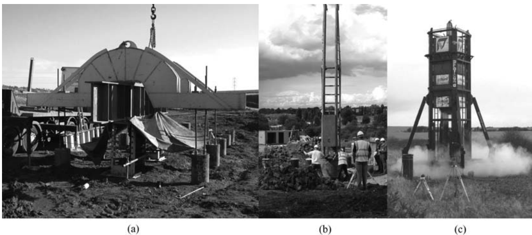
Figure 2. Photographs of the pile tests underway: a) Static test, b) Dynamic test with sliding hammer and c) Rapid test.
