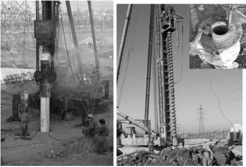
Figure 14. Driven pile. CFG-pile production. Small Pict.: hollow stem of auger ( \varnothing 10–12 cm).
