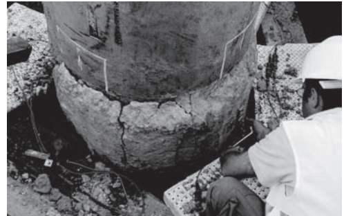
Figure 35. Damage to the pile after a high-energy impact.
