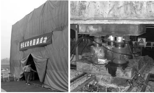
Figure 5. Tent for protecting the equipment. Top of a test pile with hydraulic jacks.
