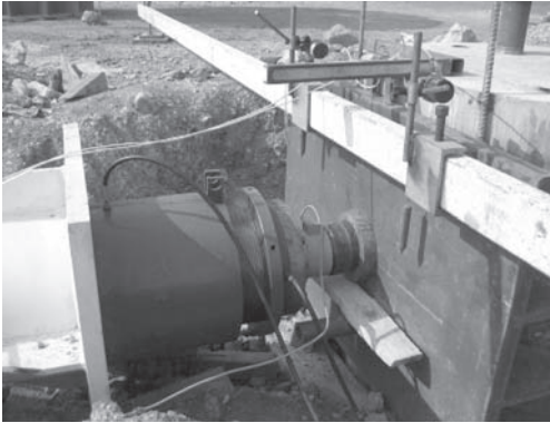
Figure 8. Detail of the hydraulic jack and reference bridge in case of horizontal load test.
