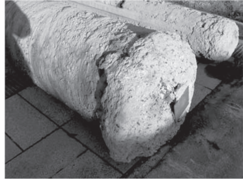
Figure 13. Excavated CFA pile (left) with casing site Loenhout—detail of the pile base.
