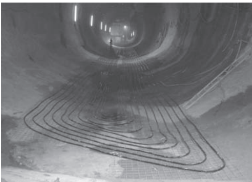
Figure 8. NATM driven station tube at “U2/2 Taborstraße” with thermal activation of tunnel invert.
