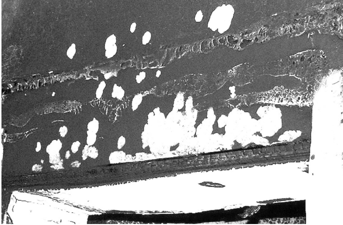
2.2 Spalling above a doorway.
