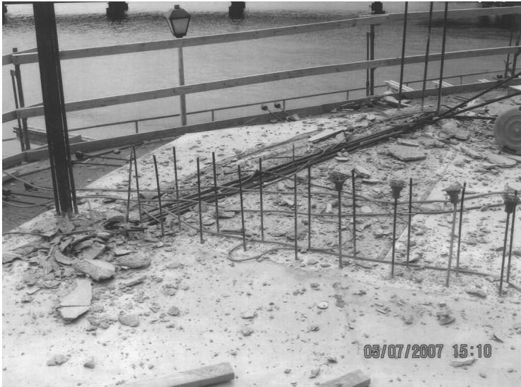
4.3 Tendons displaced during post-tensioning operations.
