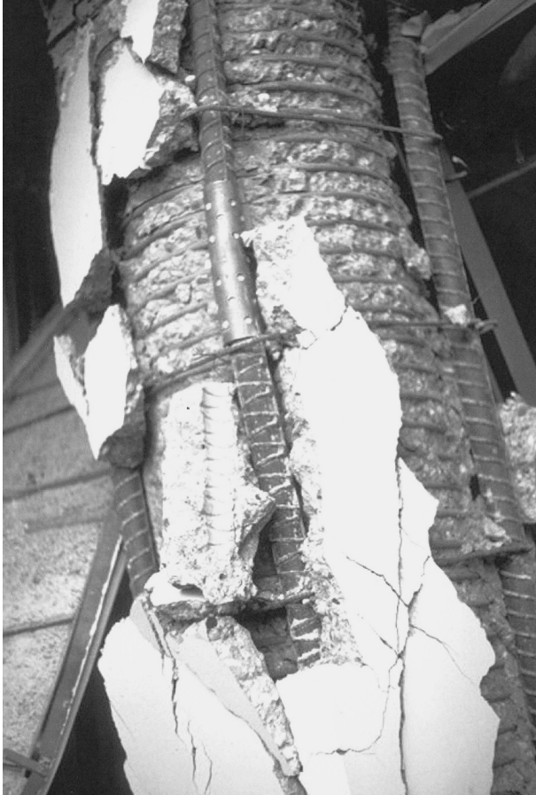
2.10 The detailed view of the column with spiral confinement steel, which helped keep the concrete core intact. 8
