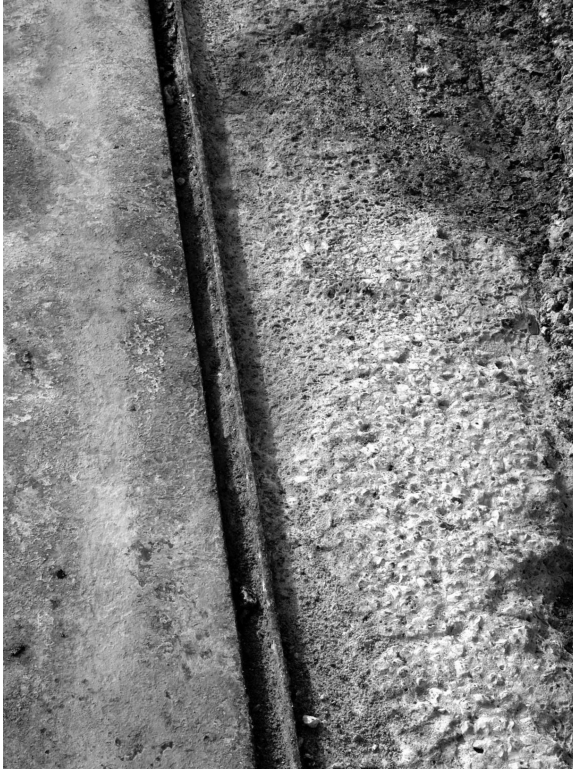
2.1 Dissolution of the concrete structure of a chemical wharf in the sea port as a result of the acidic leakage.
