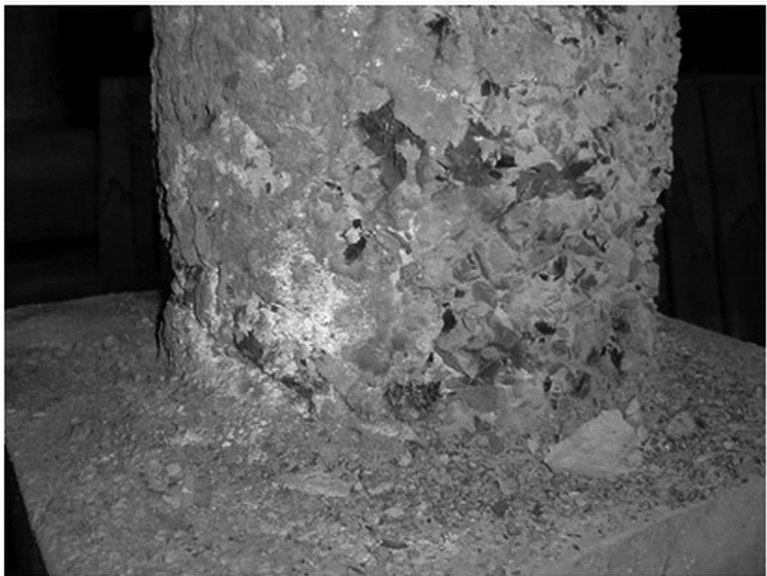
3.7 Sulfate attack at the base of a conventionally reinforced concrete column
