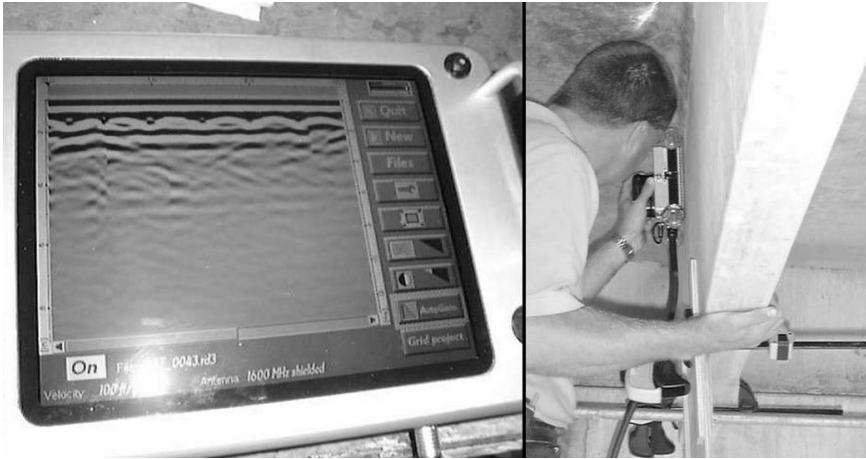
4.21 Use of GPR in identification of prestress tendons in a double-tee stem prior to coring.
