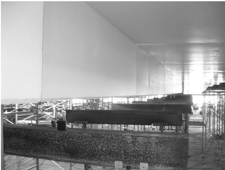
4.33 Shoring installed with gap to aid the structure in case of excessive deflections.
