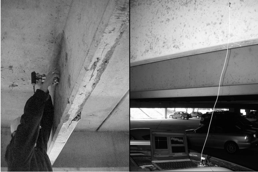
4.13 Impact-echo measurements at a fire-damaged precast double-tee using the multiple-sized impactor and transducer assembly.
