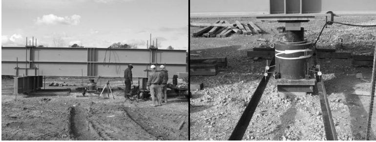
4.39 Pile load testing using a hydraulic jack and reaction frame anchored to adjacent piles.
