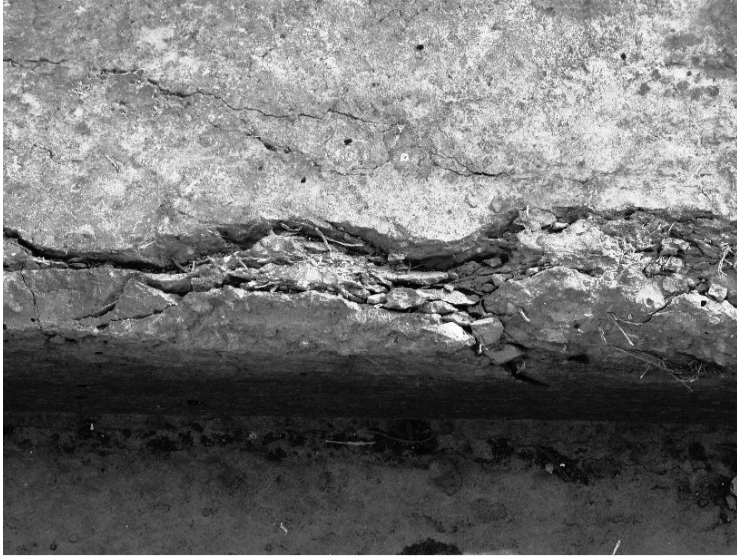
2.6 Typical impact damage of structural synthetic fiber-reinforced concrete.
