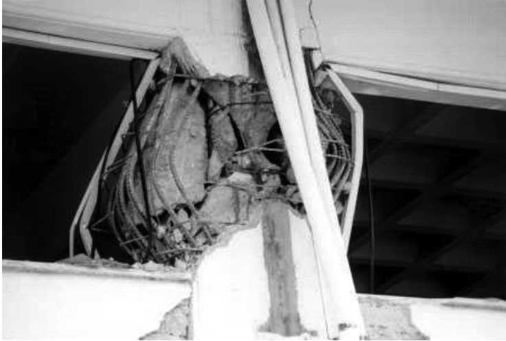
2.7 Crushing failure at bottom of column. 8
