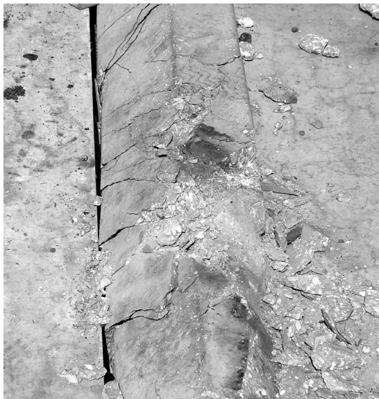
2.4 Typical impact damage of high-strength concrete containing silica fume.
