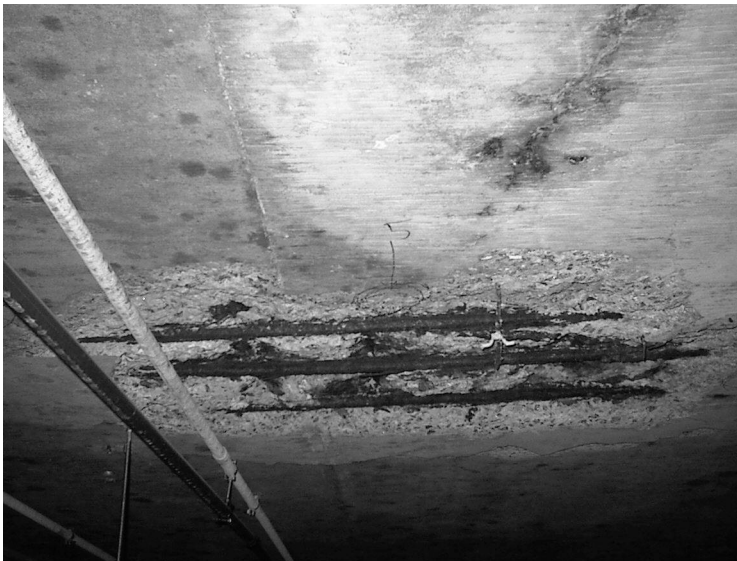
4.4 Reinforcing steel exhibiting corrosion leading to dislodged cover.
