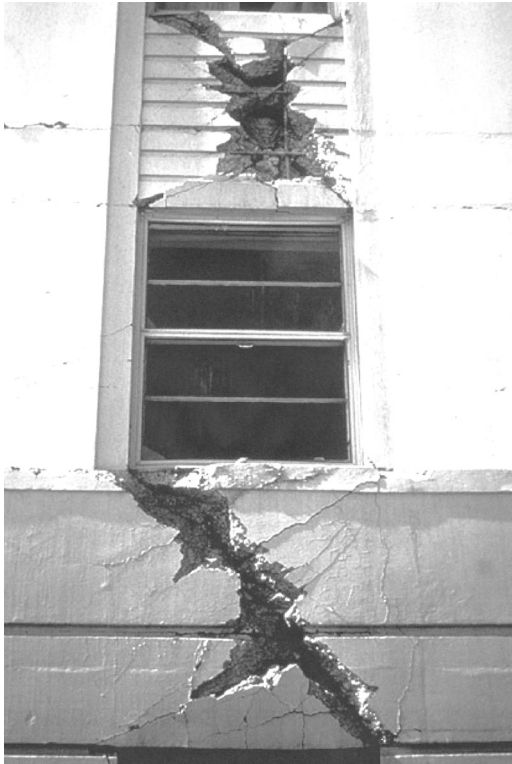
2.8 Close-up of characteristic X-shaped cracks and failure of coupling girders or short spandrel girders in the apartment building, Anchorage, Alaska. These girders were not properly designed for the shear demands.
