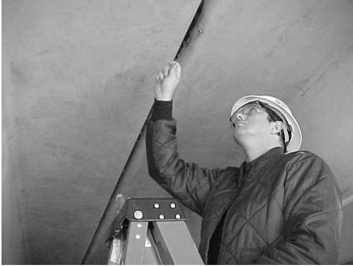
4.7 Sounding survey of precast double-tee connections for dislodged cover due to corrosion.
