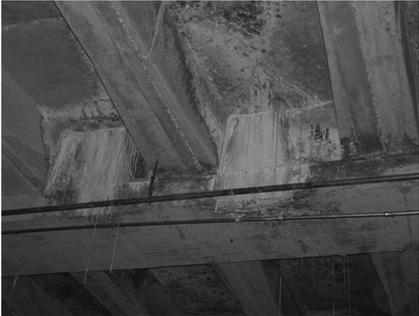
3.6 Efflorescence visible below a conventional reinforced concrete deck. (Courtesy of WJE)
