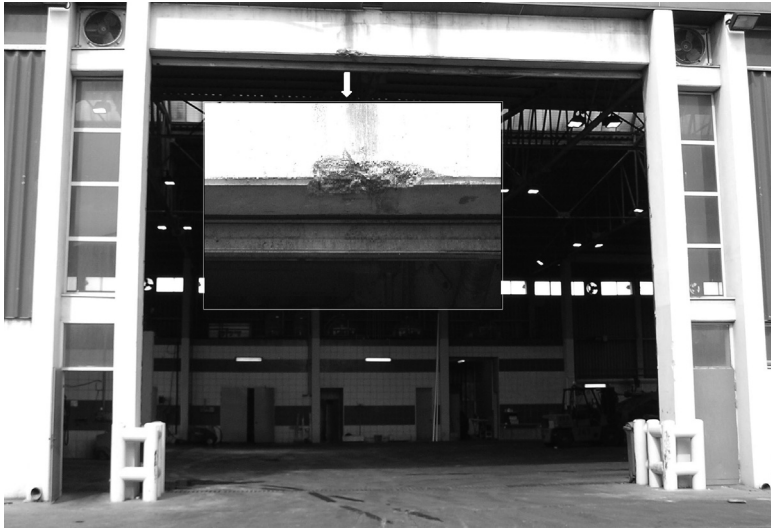
2.13 Damage of the gate frame by high vehicle.
