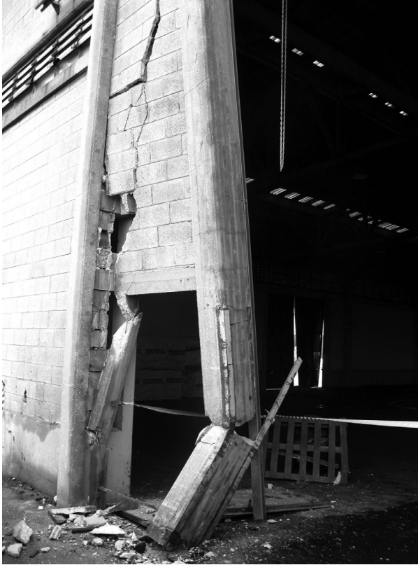
2.11 Damage to a concrete column caused by human error.
