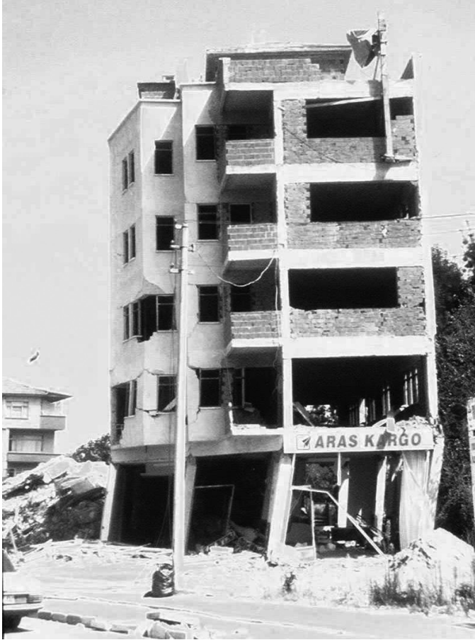
2.9 A weak-story mechanism developed at the first floor of a reinforced concrete building.
