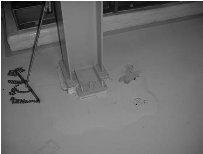
4.8 Chain drag apparatus used on a bulging industrial floor coating.
