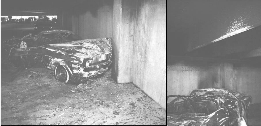
4.5 Impact and fire damage to precast concrete structure.
