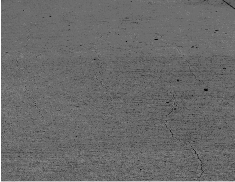
3.1 Plastic shrinkage in a bridge deck.
