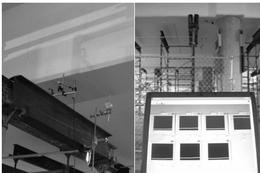
4.35 Digital LVDT allowing real-time monitoring of deflections and analog dial gauge back-up.
