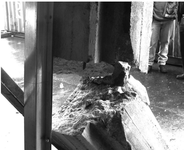
2.12 Zoom at the column cross-section demonstrating insufficient reinforcement.
