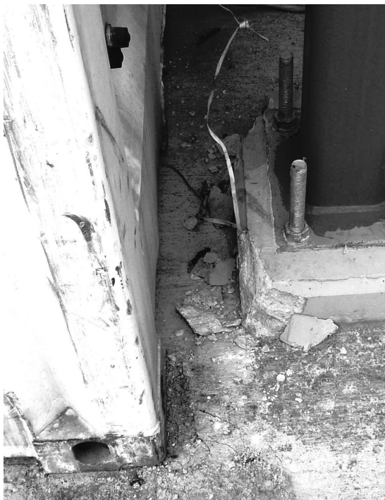
2.5 Typical impact damage of regular concrete.
