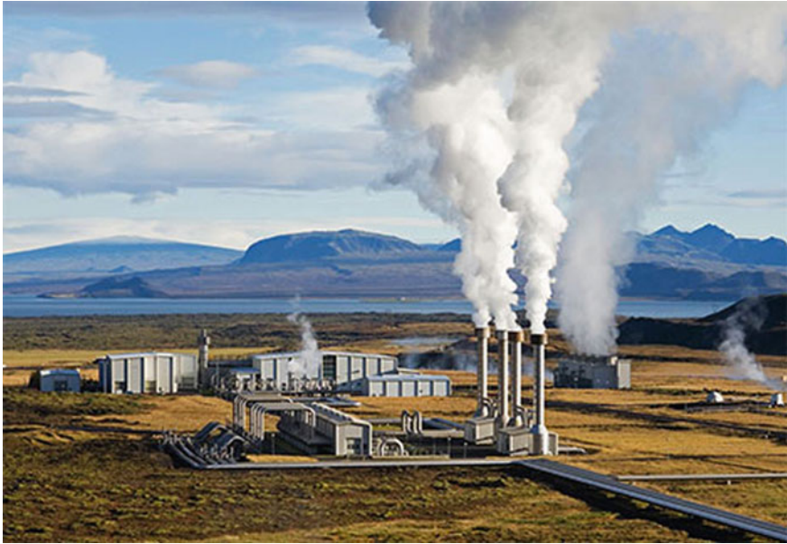
Fig. 5.24 Typical external view of the GTPP
