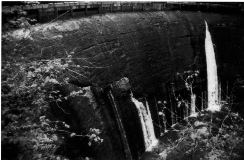
FIGURE 9.2 Water flowing from large cracks in a concrete dam face. (Courtesy of Engineered Solutions, Inc., Davis, CA.)
