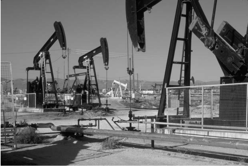
Exhibit 6.2 Oil Pump Jacks Source: Marli Bryant Miller, University of Oregon.
