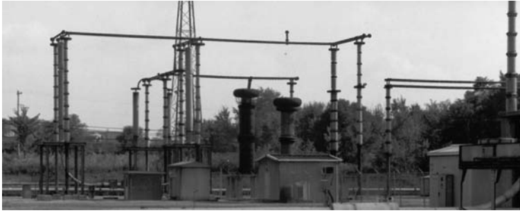
FIGURE 6.10 800-kV dc terminals of a converter station.
