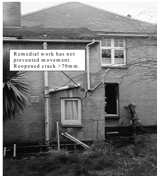
Figure 7 Subsidence induced cracking in a house in Devon, as a result of loess collapse and subsequent post-wetting consolidation (after Hunter et al. , 2001)
