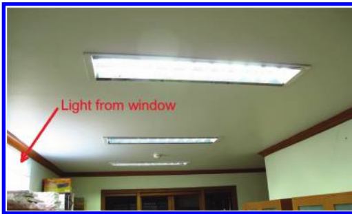
Figure 8. Example of uncontrollable window light.
