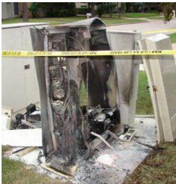
Fig. 4.3 The result of an Avestor battery fire in an AT&T system. Reproduced with permission—Copyright 2012, IEEE (Whittingham 2012)
