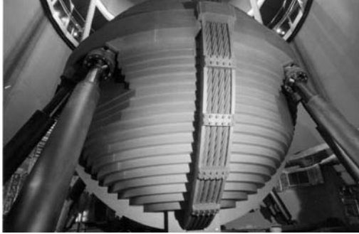
Figure 4.9: A pendulum-style tuned mass damper used in the recently completed Taipei 101, Taiwan. Photograph courtesy of Rowan Williams Davies and Irwin Inc. and Motioneering Inc.
