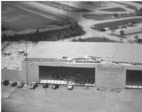
Fig. 3.5: Windward leaky hanger doors during Hurricane Andrew increased the net leading-edge roof pressures, via larger internal pressures.
