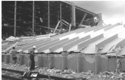
Fig. 1.5: A roof deck failure during Hurricane Andrew left the precast walls unsupported and so they failed along the internal floor slab line.
