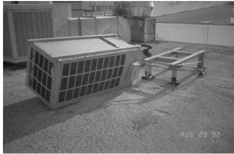
Figure 4.19: Topped rooftop HVAC equipment during Hurricane Andrew (1992).
