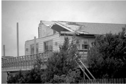
Fig. 3.8: A failed beachside deck canopy and adjacent roof segment becomes a source of many sizes of debris for downwind buildings.
