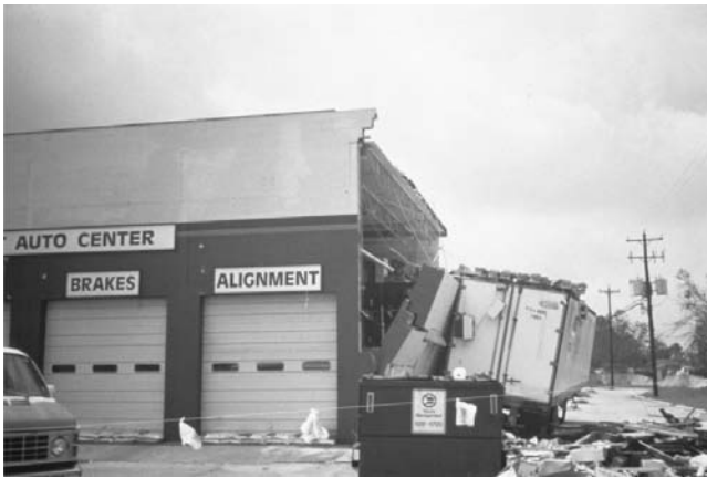
Fig. 3.4: Increased internal pressure, caused by a windward window failure (not shown to the left), overloaded the leeward unreinforced blockwork wall (Hurricane Andrew). The critical wind was from left to right.
