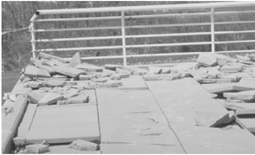
Fig. 1.4: Paver damage on a lowrise office complex during Hurricane Andrew in 1992.
