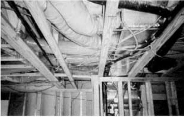
Fig 3.2 Entangled building systems. Photograph by Stephen Kendall.
