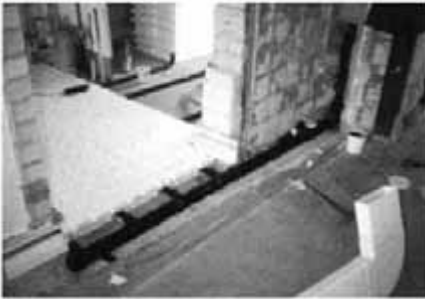
Fig. 7.2 Matrix Tile and 0-slope gray-water drain line installation. Photograph by Stephen Kendall.
