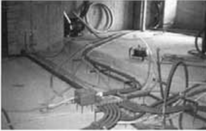
Fig. 4.61 Service lines being installed in Support trench. Photograph courtesy of Mitsuo Takada.
