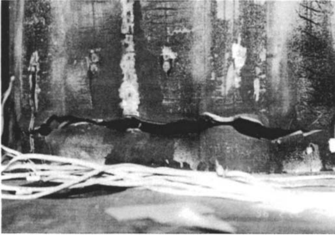
Photo 1 Local Buckling and Crack on the Base Plate Connection (Specimen Type-2 Before Retrofit)
