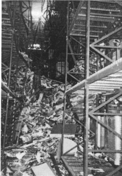
Figure 1 - Collapse of hot rolled steel shape rack
