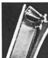
Figure 6: Typical Failure of the Stud between the Top Screw Fasteners.
