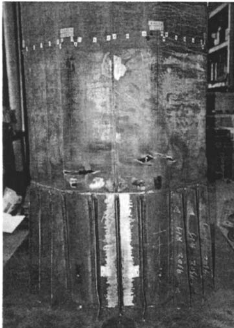
Photo 2 Local Buckling and Crack above the Retrofit Portion (Specimen Type-1 After Retrofit)
