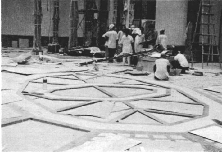
Figure 5: A view of the BCCFP floor at the Hyatt Hotel during construction
