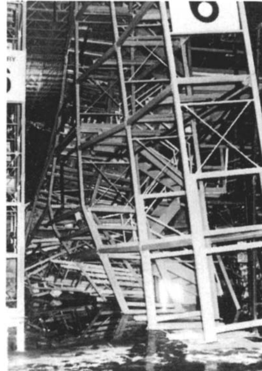
Figure 2 - Collapse of cold formed steel shape rack
