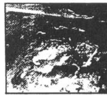
Exposed Reinforcing Steel
