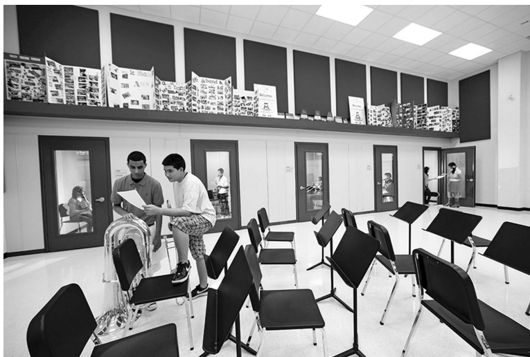
Figure 12.2 A music rehearsal environment requires both walls and doors to have good sound isolation properties. Door seals are critical. (Photo courtesy of Acentech, Studio A.)
