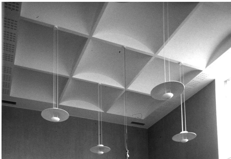
Figure 12.6 Ceiling with concave elements combined with slit sound absorbers at flat ceiling section next to walls. (Photo by Mendel Kleiner.)
