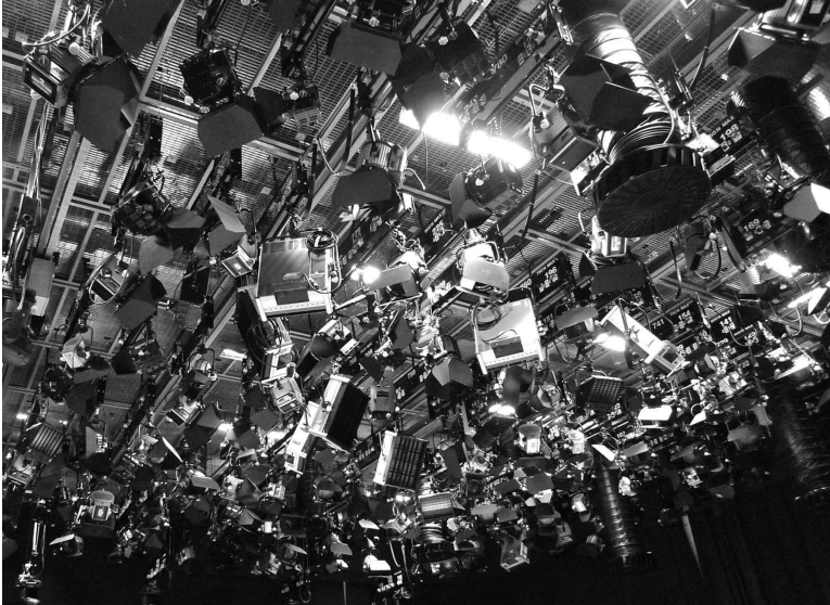
Figure 12.7 Lighting equipment functions also as volume diffusers in the ceiling of a television studio. (Photo by Mendel Kleiner.)
