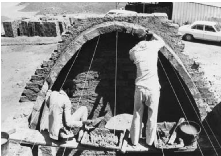
Fig. 15.8 Nubian vault: African builders from Southern Algeria, Chad and other drought-stricken areas where there are few trees are taught how to construct the Nubian vault from mud bricks, without the use of wooden formwork, reinforcement or beams (Photo: © Development Workshop)
