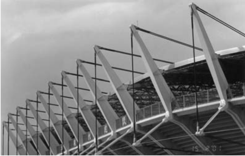
Fig. 3.1 Beams supporting the roof at the Ulsan World Cup Stadium (Photo: Kevin West)
