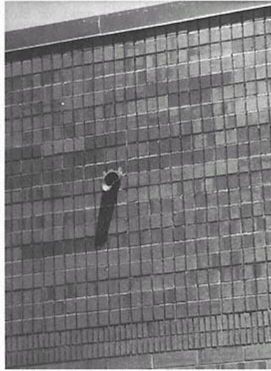
Figure 3-5 Drainage from low sloped roofs with parapet walls accomplished with a penetration through the roof wall called a parapet scupper. Photo by author.
