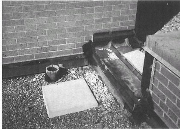
Figure 8-2 Plumbing vent. Note that flashing is carried up and over the pipe. Photograph by author.
