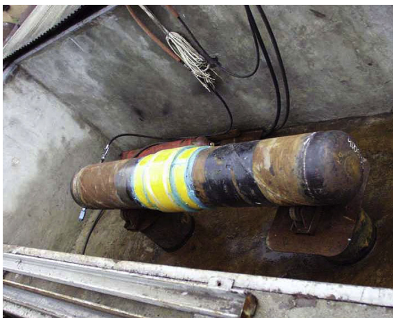
Figure 6.16 Photo of burst test section of girth weld repair.
