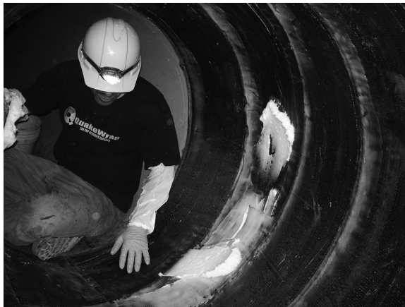
Figure 3.3 Worker installing 24-in (610-mm) wide strips of carbon fabric in a curved section of a 42-in (1065-mm) steel pipe with overlapping joints in the direction of flow.
