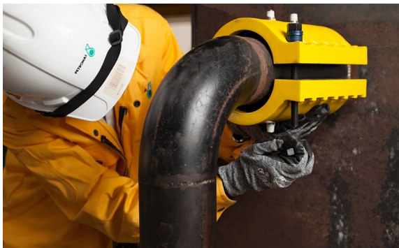
Figure 12.17 Installing a composite repair clamp onto a pipe with a through-wall defect.
