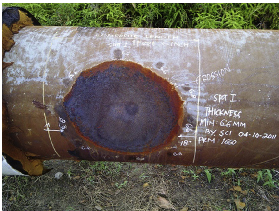
Figure 6.18 Sample of the CUI defect.
