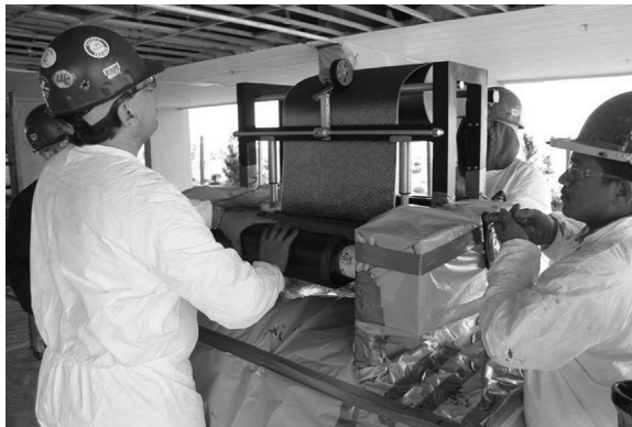
Figure 2.5 Saturation of carbon-fiber fabric of epoxy primer. Courtesy of Structural Technologies, LLC.
