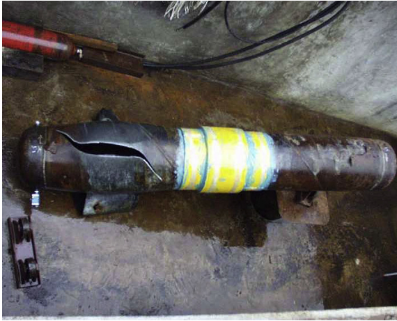
Figure 6.17 Failure of the pipe occurred outside of the repair area.
