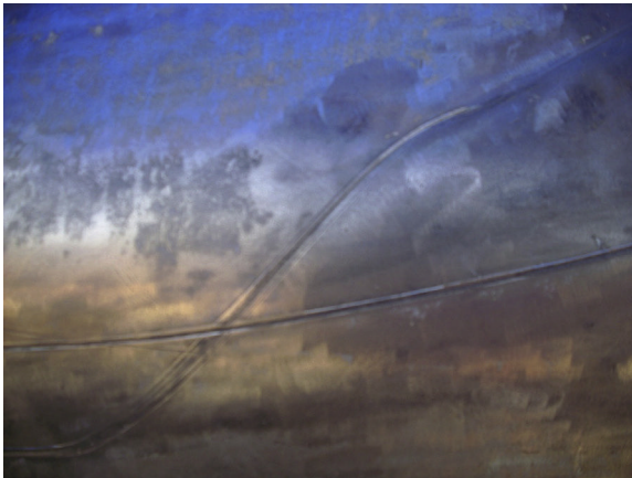
Figure 6.5 Mechanical damage defect on the 28-in. gas line.
