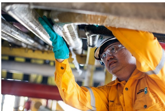
Figure 12.14 Overwrap repairs are also advantageous for repairing piping, especially where there is restricted and limited access.
