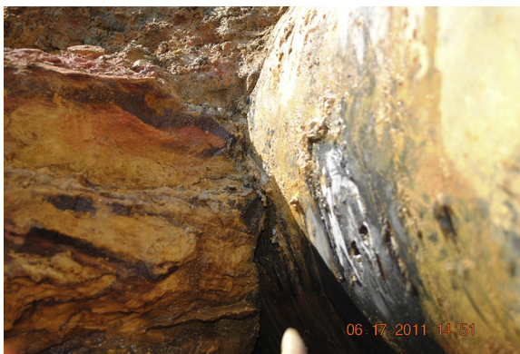
Figure 6.9 The alkaline soil erosion type defect.
