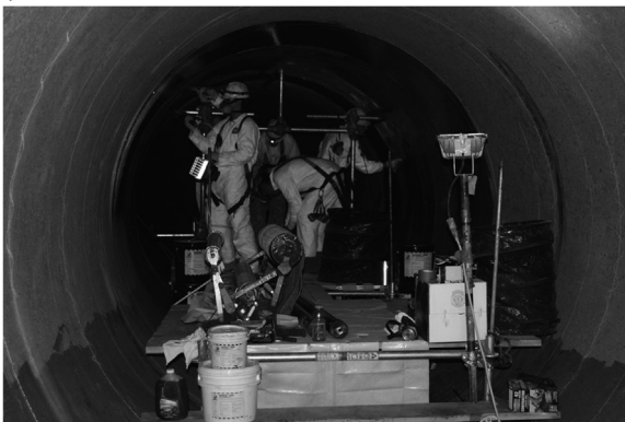
Figure 3.2 (a) Collapsible saturator machine is lowered into the pipe through a 24-in (610-mm) access port and (b) it is reassembled inside the 120-in (3-m) pipe.
