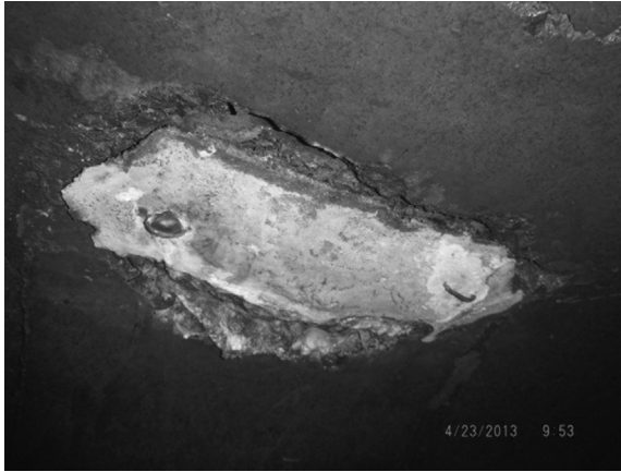
Figure 1.5 Corrosion of steel cylinder. Courtesy of Mr Michael Ambroziak of CPM.
