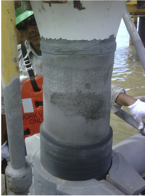
Figure 6.11 Sample of CUI defect.
