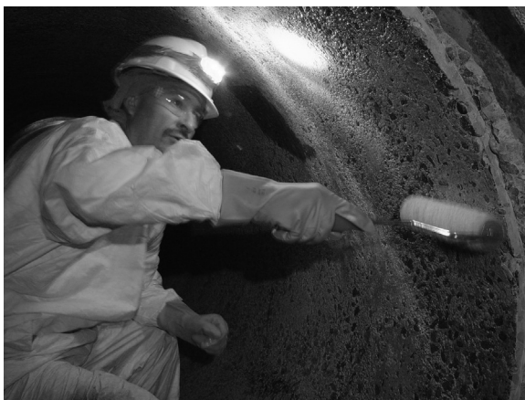
Figure 2.4 Application of epoxy primer. Courtesy of Mr Hector Posada of Tucson Water.
