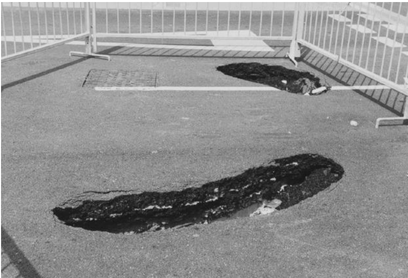
Figure 1.18 Surface subsidence following inadequate compaction of backfill around a soak-away.
