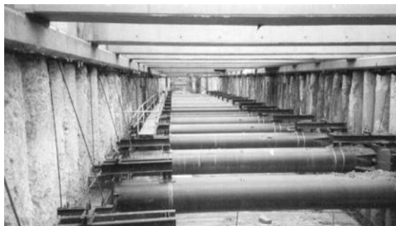
Figure 9.8 Contiguous bored pile retaining wall with permanent reinforced concrete and temporary tubular steel props during construction. (Courtesy of Professor D.J. Richards.)
