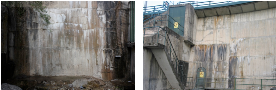
Figure 5. Downstream views of the bottom zone of the right arch (on left) and of the upper zone of the left arch (on right), in 2015
