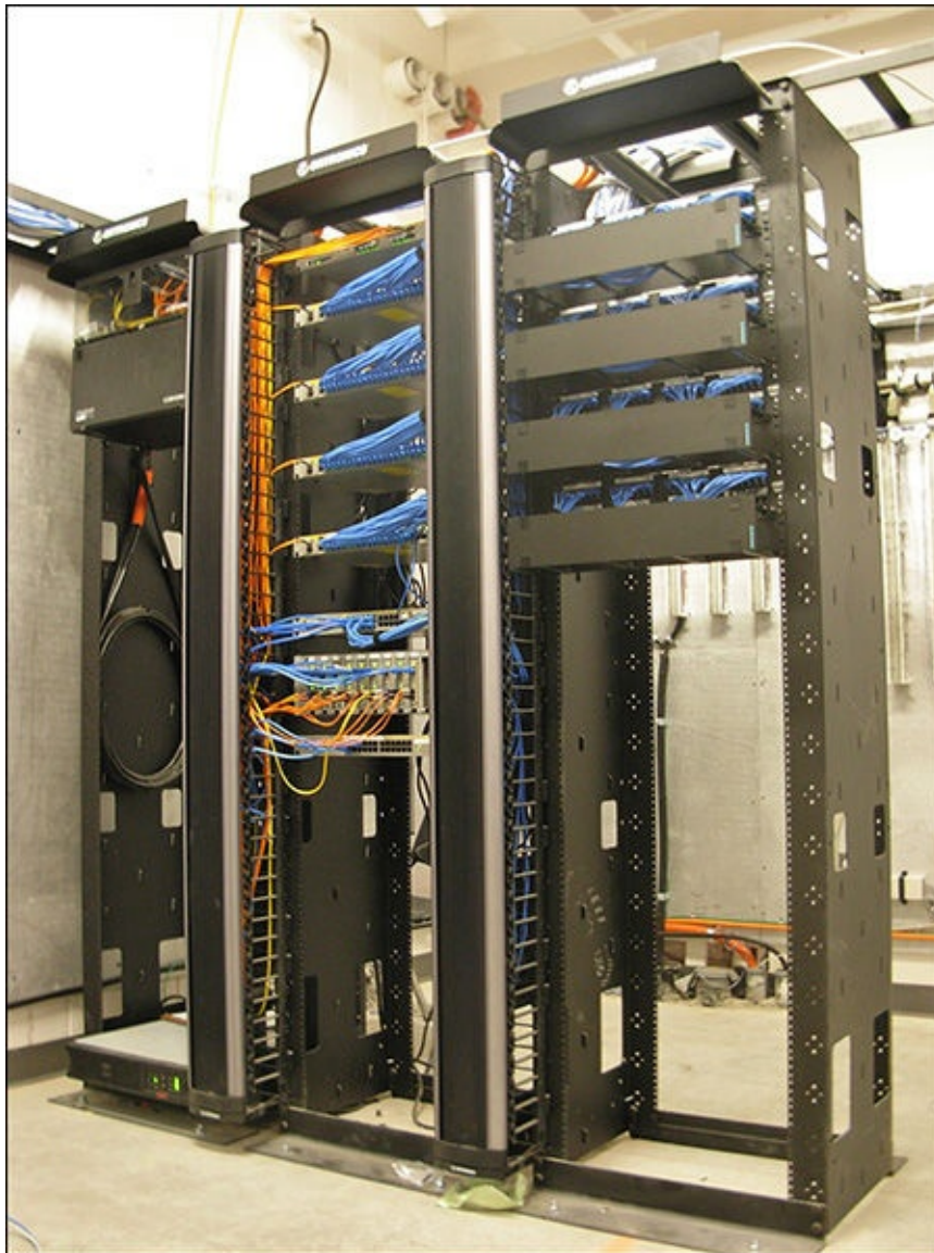
FIGURE 2-5 Inside a telecommunications closet.
