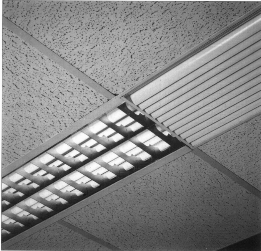
Figure 15 Example of air diffusers located in lighting units
