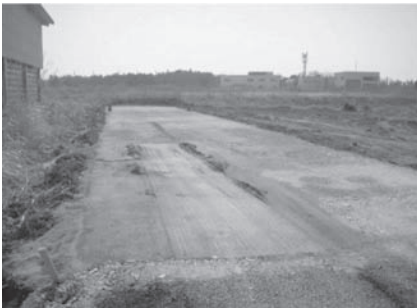
Photo 1. Test pavement condition after loading test.
