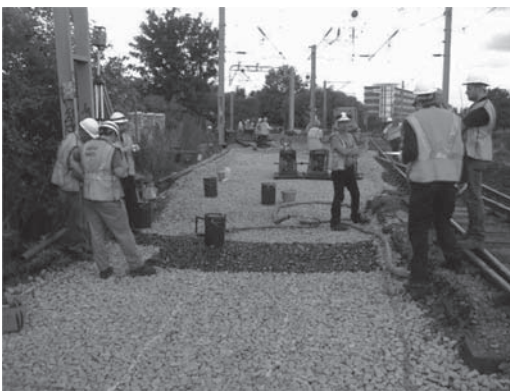
Figure 1. Application of 3D polyurethane reinforcement at a bridge transition on the Stansted to London line UK.
