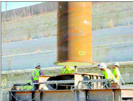
Figure 13. Bolting flanges on well casing
