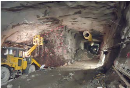
Figure 20. Drilling the top heading west side slash in station cavern after completing the center drift
