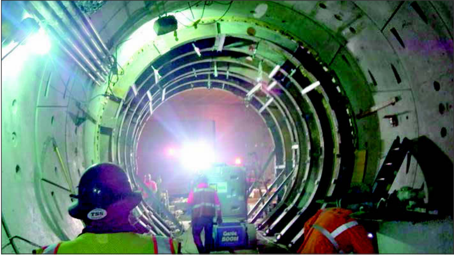
Figure 9. Formwork for final SB tie-in to the pre-existing PSST (the light at the end of the tunnel)
