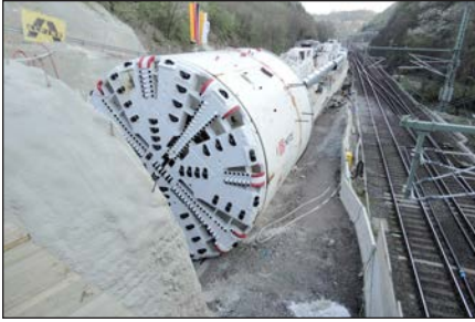
Figure 2. View of the TBM's starting position at the Ediger-Eller portal (Source: ABT, 2010)
