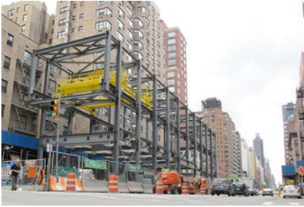
Figure 12. Construction of one of two Muck Houses erected at the site—for efficient materials handling
