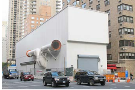
Figure 13. Operational Muck House at 72nd Street site. Ventilation and electrical systems are also enclosed.
