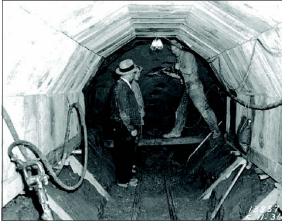
Figure 3. Pneumatic spaders used in the hard clay heading of the timber supported Henderson Street Sewer Tunnel, ca. 1936 (Seattle Municipal Archives Photograph Collection Item No. 10381)
