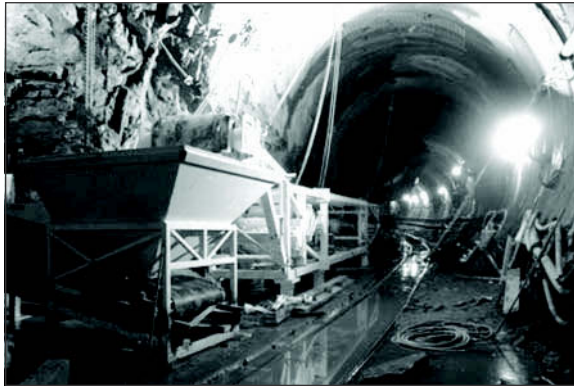
Figure 3. Take-up unit and transfer belt on crusher branch prior to 36-inch belt installation
