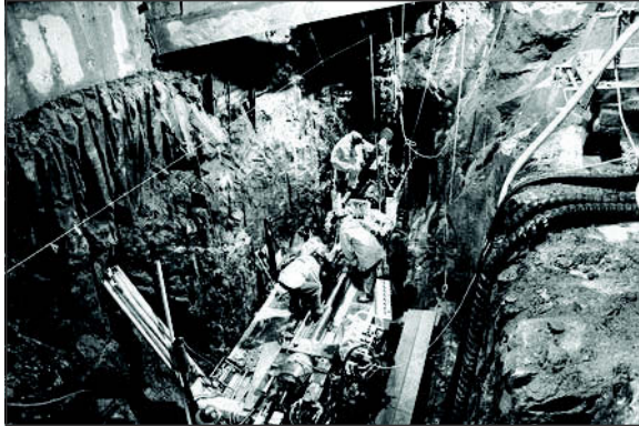
Figure 8. Drilling of the lowermost freeze holes from a deep pit excavated in rock. The lowermost pipes had to be installed full length through competent rock.
