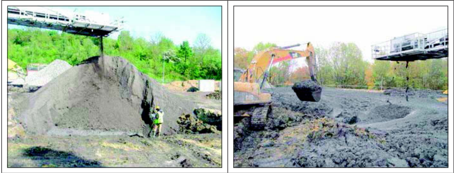
Figure 16. Turning the clayshale rock into a plastic mud by adding several cubic meters of water and foam was unavoidable but also the best solution
