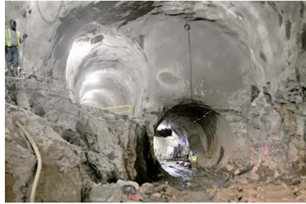
Figure 30. Completion of the G3 and G4 tunnels at the Stub Cavern—with a final separation of only 6 feet
