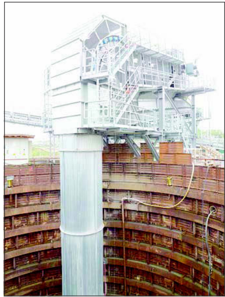
Figure 5. Vertical conveyor, head station
