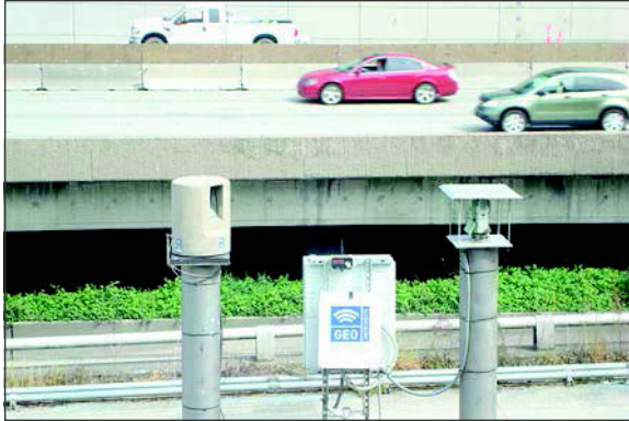
Figure 5. Typical AMTS installation
