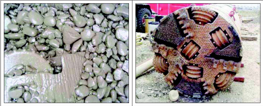
Figure 1. Woods Trunk Sewer Replacement Project. Left: Crushing chamber packed with gravel after MTBM stalled. Right: MTBM cutterhead after modifications including closure pieces to reduce COR. (Staheli 2008)
