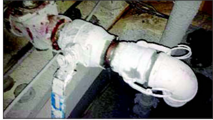
Figure 7. Air vent port used for bleeding accumulations of compressed air on U230 project
