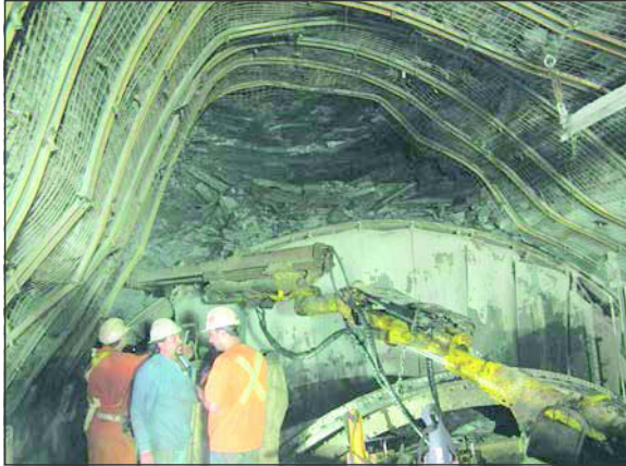
Figure 2. Overbreak issues in recent two-pass tunnel in shale
