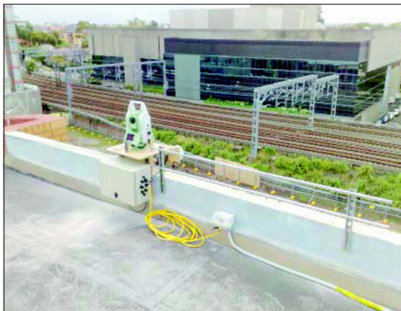
Figure 5. Typical robotic monitoring set up for track deformation
