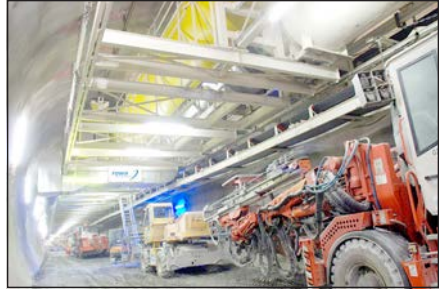
Figure 5. CBT—Increased safety due to predefined parking and working areas, rationalization of all work flows and generous illumination (Courtesy of Rowa, www.rowa-ag.ch )
