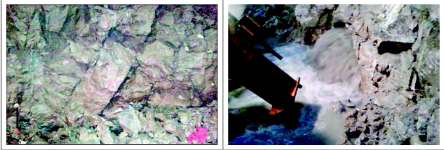
Figure 5. High angle joint in limestone with clay in-filling, and water inflow through joint
