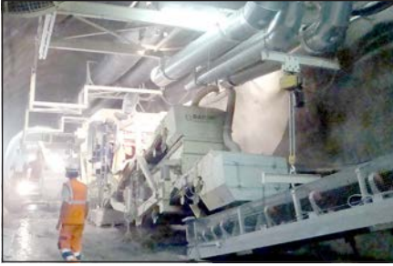
Figure 4. CBT—Telescopic ventilation platform for optimal fresh air supply to the face and efficient flushing of blasting fumes (Courtesy of Rowa, www.rowa-ag.ch )
