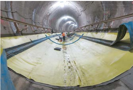
Figure 41. Invert waterproofing installation in the running tunnel. The blue material is water barrier.
