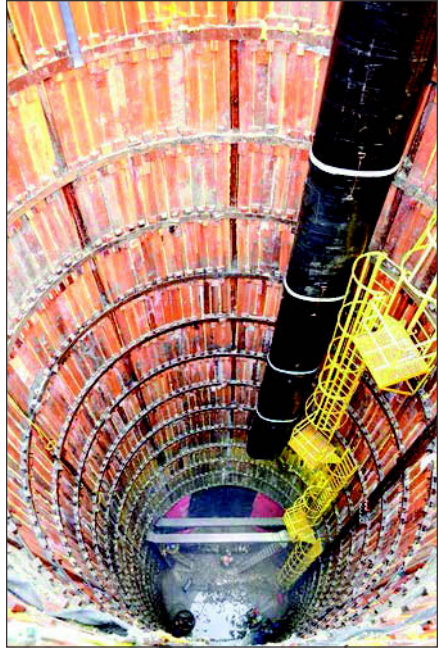
Figure 12. Bay Tunnel–Newark shaft freezing with ring beams and wooden lagging support. Photo courtesy of the SFPUC.
