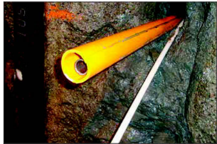
Figure 4. HIPI casing installation during U215 contract. Note temporary internal push rod and counterweight for casing grouting operation.
