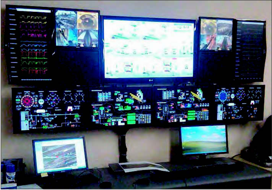
Figure 23. Main site office—system control center
