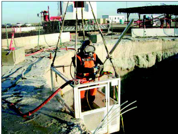
Figure 11. Bay Tunnel–Ravenswood shaft using diver to inspect and connect steel reinforcement. Photo courtesy of the Global Diving and Salvage.
