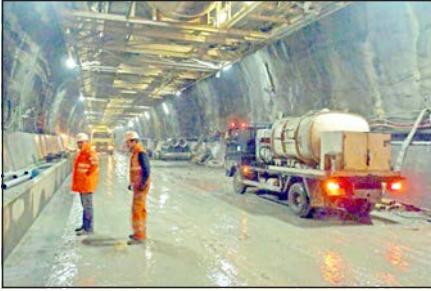
Figure 11. RPHT—Rationalization of work flows and increased safety due to a second level for working and parking below the heading platform (Courtesy of m+m, www.moergeli.com )
