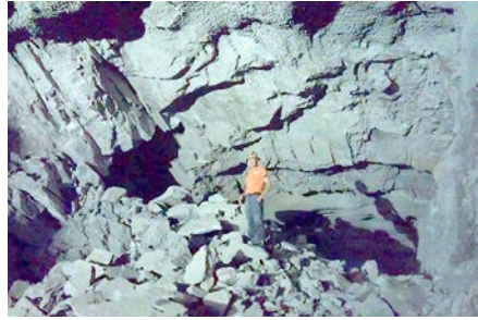
Figure 23. Holing-through the center top heading 1 before starting the east and west side slashes, 2 and 3
