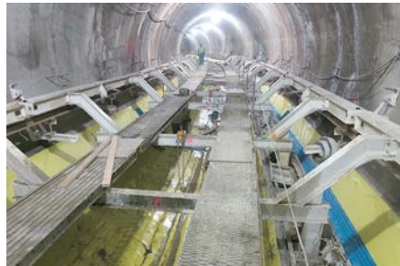
Figure 42. Tunnel invert forms in place for the pour. A follow-on arch pour will complete the tunnel lining.
