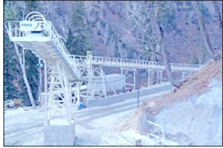
Figure 12. RPHT—Continuous conveyor and discharge tower at the muck disposal site (Courtesy of Rowa, www.rowa-ag.ch )
