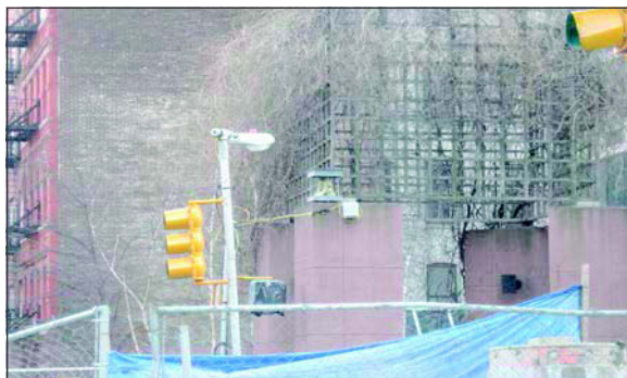
Figure 7. AMTS on Second Avenue project with power from light pole
