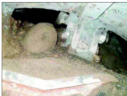
Figure 8. Boulder in cutterhead opening with ground loss void due to running ground
