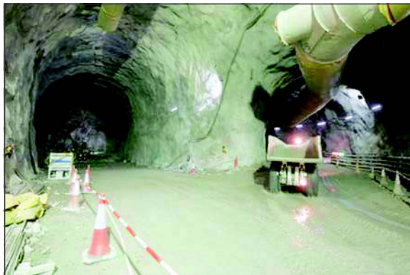
Figure 6. Intersection of south bypass (right) and Kwai Chung adit. The drill jumbo is faintly visible at left working in the junction area.
