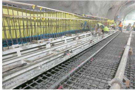
Figure 32. Placing concrete in a station invert slab after all forms, rebar and piping were in place
