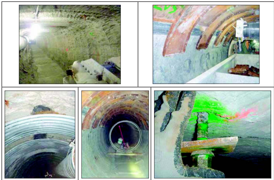
Figure 2. (Clockwise from top left) Spot bolting in Austin Chalk; semi-circular liner plates supporting bentonite zones; rock bolt failure in pyroclastic material; liner plates; steel arches supported pyroclastic materials
