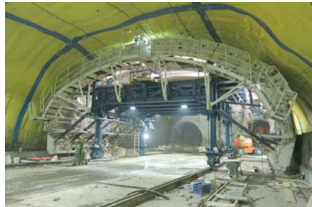
Figure 36. Cross-Over arch form in place in the North Cross-Over—ready for the first pour
