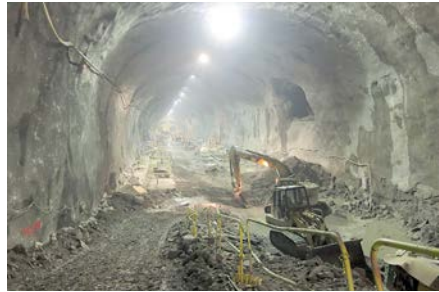
Figure 25. Final stage of station cavern excavation before the start of final lining operations
