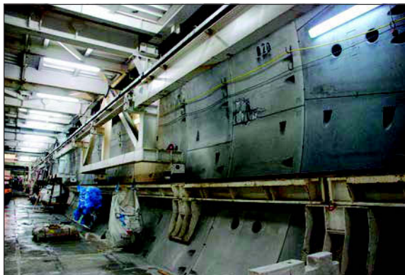
Figure 2. Support brackets and gantry above
