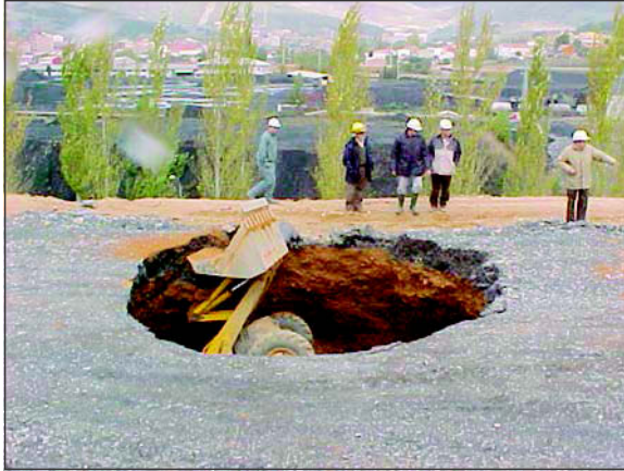
Figure 13. TBM tunnel collapse produced by over excavation
