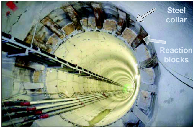
Figure 14. Bracing for EPBM start in underground station consisted of a steel collar and reaction blocks
