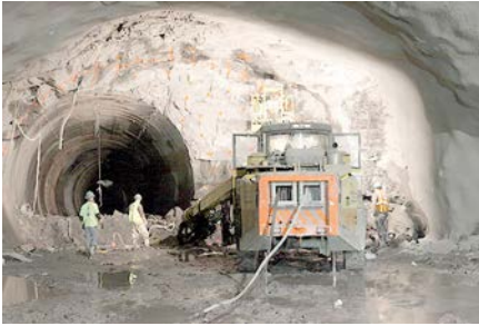
Figure 29. Drilling for rock excavation in the G4 turn-out cavern. A previous TBM tunnel is on the left.
