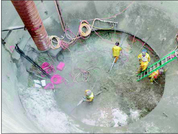
Figure 4. Drilling for rockbolts at the Calaveras Dam intake shaft. Photo courtesy of Drill Tech drilling and Shoring, Inc.
