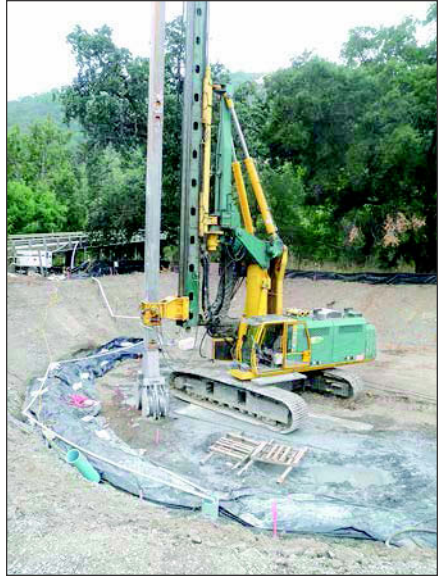
Figure 2. Cutter soil mixing construction at the launching shaft at the Sunol Valley Water Treatment Plant. Photo courtesy of Drill Tech Drilling and Shoring, Inc.
