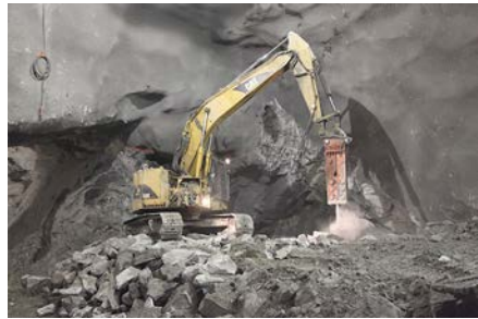
Figure 21. Final muck removal in the station cavern after completing the cross-overs and bench excavation
