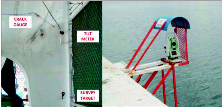
Figure 9. Instrumentation in Shed #2 (left) and automated total stations used for data collection (right)
