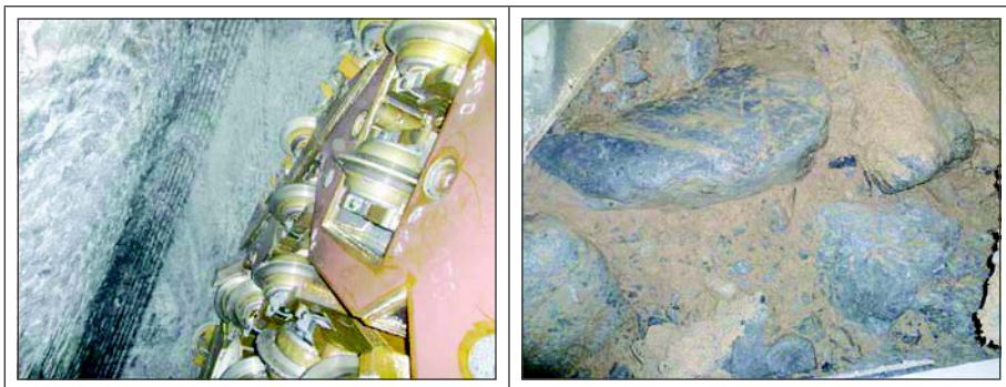
Figure 6. Competent rock mass (left); Situation in the fault zone with loose blocks embedded in a loamy matrix (right)
