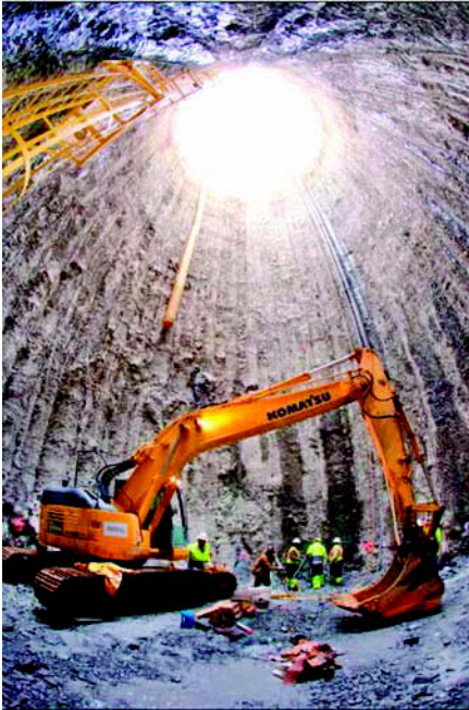
Figure 3. Secant pile shaft at the New Irvington Tunnel Project. Photo © Jacobs Associates 2003.
