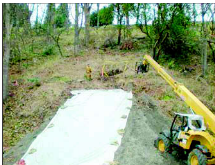
Figure 9. Sinkhole in bluff slope above tunnel
