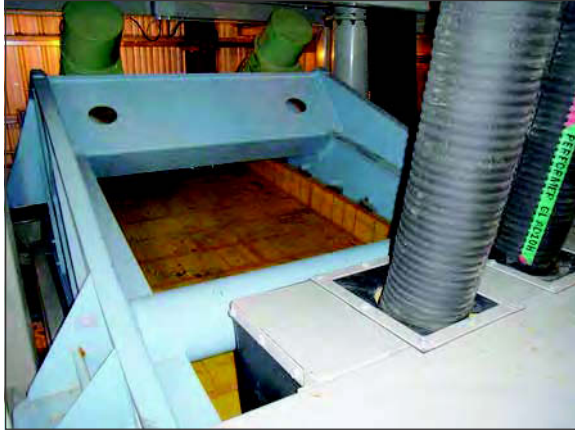
Figure 12. MS STP shaker screens
