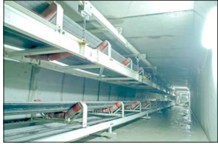
Figure 15. RPHT—Towing conveyor and continuous conveyor in the escape tunnel (Courtesy of Rowa, www.rowa-ag.ch )
