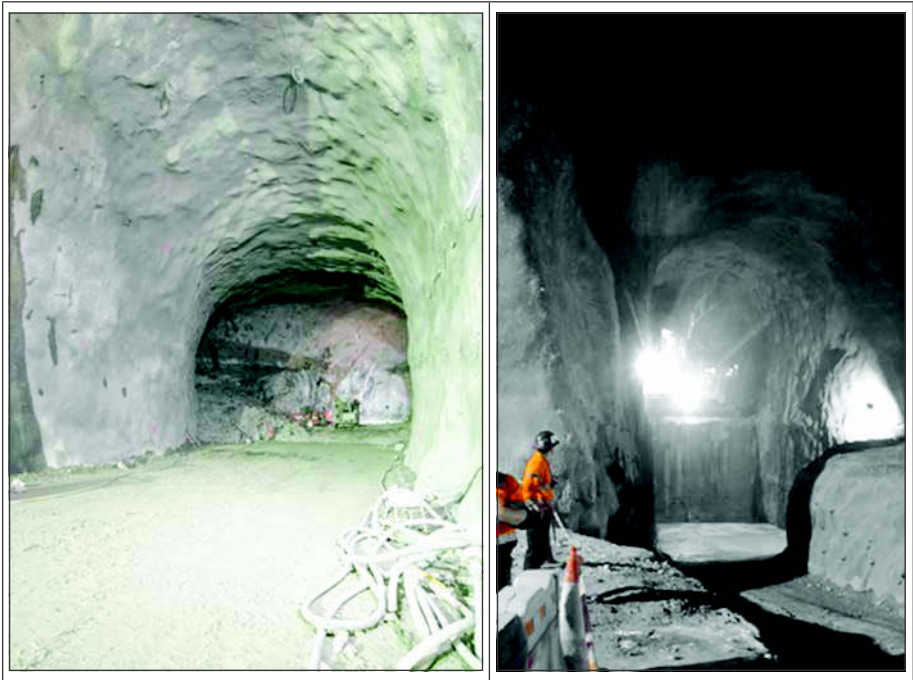
Figure 9. Completed development of junction as viewed down Kwai Chung adit (left) and the in line tunnel sump viewed from the junction (right)
