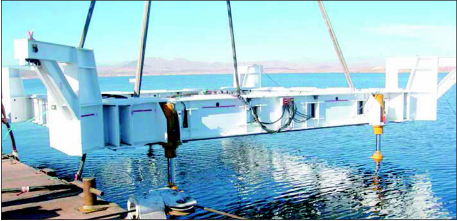
Figure 2. Guiding frame being lowered, leveling cylinders visible. Frame lowered with cylinders fully extended.
