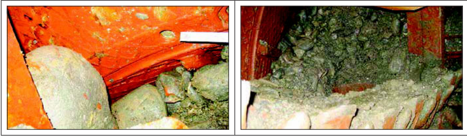
Figure 3. Alameda 4 Siphon. Left: MTBM crusher chamber with cobbles and boulders in sand and gravel matrix. Right: MTBM crusher chamber with cobbles in sand and gravel matrix. (Finney and Del Nero 2010)
