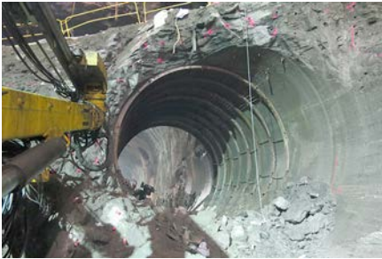
Figure 24. Final stage in the station cavern—for the removal of the rock surrounding the TBM tunnel
