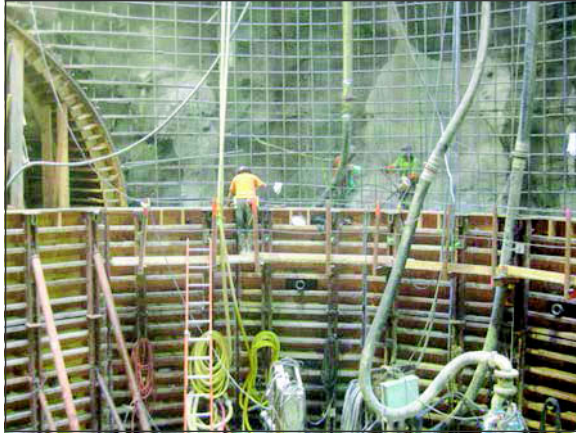
Figure 3. Concrete delivery from outside of tunnel form instead of crown pump valve
