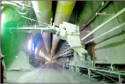
Figure 6. CBT—Cross conveyor drops the muck of the Eastern tube onto the continuous conveyor in the Western tube, (Courtesy of Rowa, www.rowa-ag.ch )
