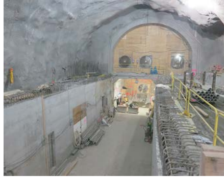
Figure 40. Stub Cavern with G4 (lower track level) completed. A soffit slab and arch pours will follow.
