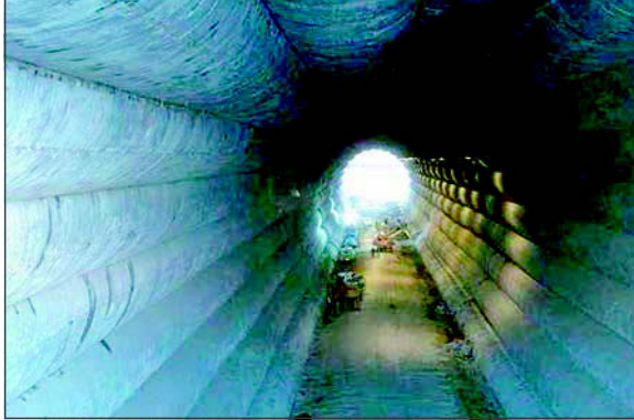
Figure 4. Mt. Baker Ridge Tunnel on Interstate 90 complete in 1986 by a unique stacked drift method to form a semi-flexible compression ring liner. The 24 cylindrical drifts are 2.5 m diameter and the excavated core is 19.8 m diameter.
