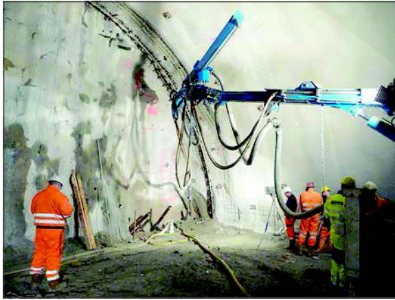
Figure 11. Filling the invert with mortar through a pipe umbrella (Source: ABT, 2010b)
