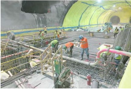
Figure 31. Constructing a station invert slab with rebar and forms. Note the waterproofing in the NXO.
