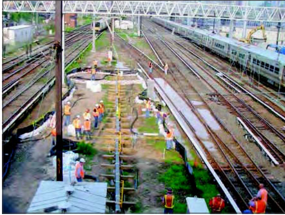
Figure 22. Slurry spill on the surface in the morning of July 23, 2012
