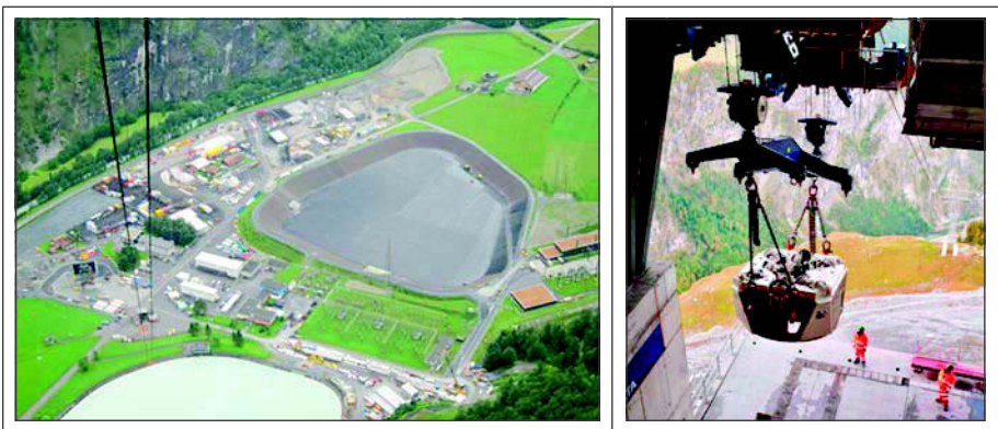
Figure 2. Access to the main work sites and transport of TBM components via cable cars
