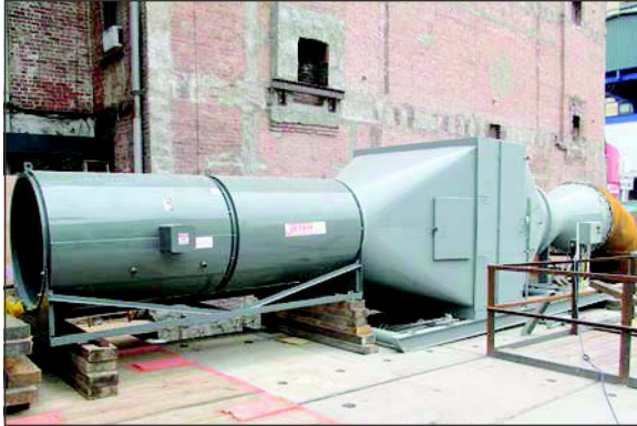
Figure 7. Photograph of wet scrubber system installed at the south shaft
