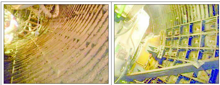
Figure 7. Additional heavy rock support measures in the Mörtalbruch zone with installation of steel cassettes as segment behind the gripper shoe
