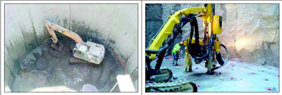
Figure 4. Excavator in Shaft 2 surrounded by diaphragm walls, and drilling for blast round
