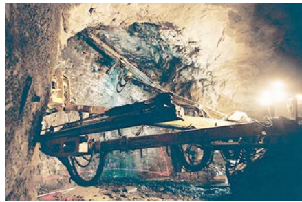
Figure 28. Drilling an adit to Ancillary 2 from the station cavern area—as the top heading proceeds
