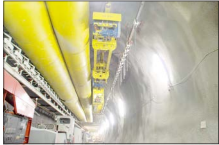
Figure 7. CBT—Monorail for direct supply to the heading area (Courtesy of Rowa, www.rowa-ag.ch )
