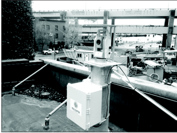
Figure 2. AMTS on building roof
