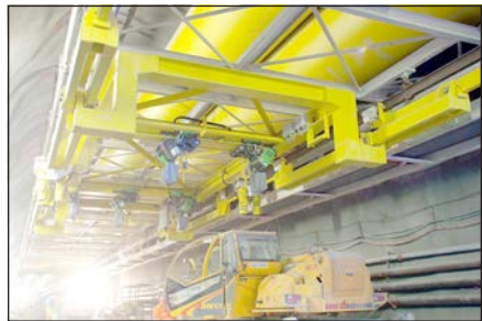
Figure 8. CBT—15-ton-capacity heavy duty crane over the invert construction area (Courtesy of Rowa, www.rowa-ag.ch )
