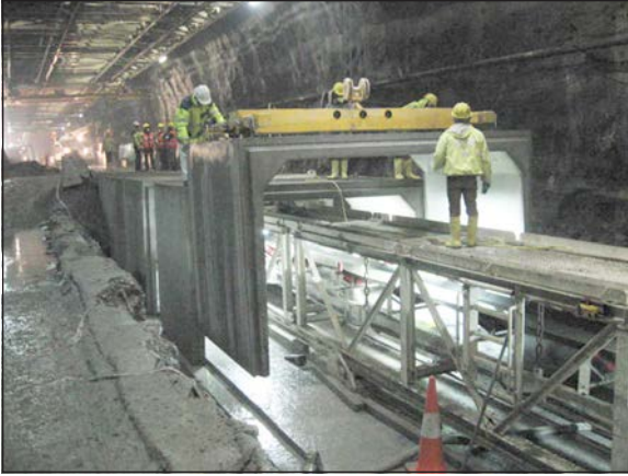
Figure 17. RPHT—Placing of the escape tunnel precast elements with a heavy duty crane (Courtesy of Rowa, www.rowa-ag.ch )
