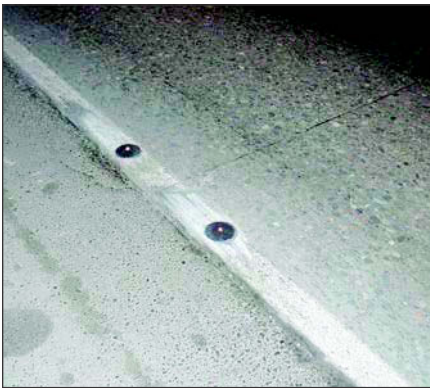
Figure 6. Road prisms at pavement panel corners
