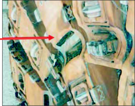
Figure 2. Detail of the damaged structure
