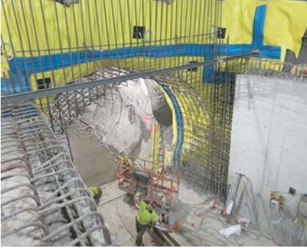
Figure 39. Stub Cavern walls at G4 tunnel. A soffit slab will follow to complete this over/under structure.
