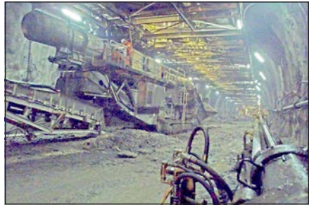
Figure 14. RPHT—Heading platform, jaw crusher and towing conveyor for bench/invert excavation (Courtesy of m+m, www.moergeli.com )
