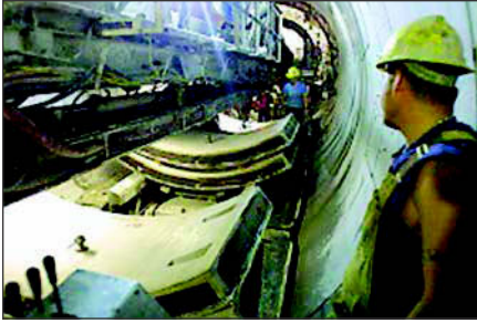
Figure 5. Gasketed segmental lining installed behind trailing gear of the EPBM in the Mercer Street Tunnel
