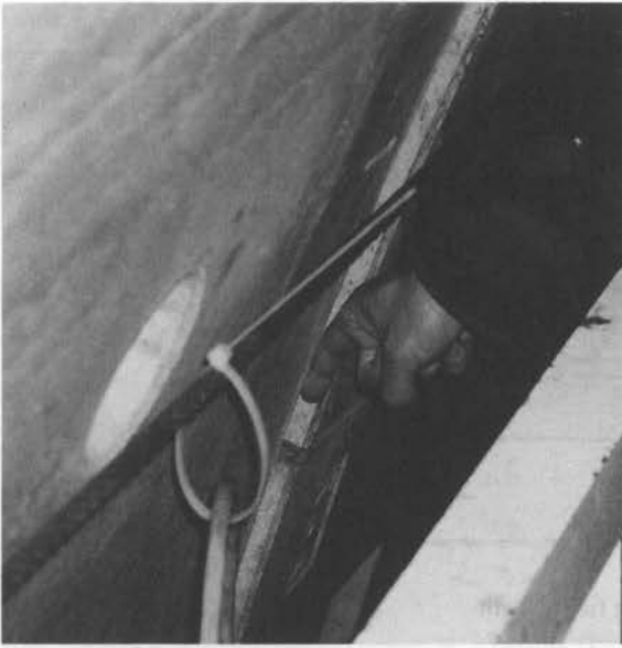
Figure 7.33 Differential displacement as observed at the Second Heineoord tunnel
