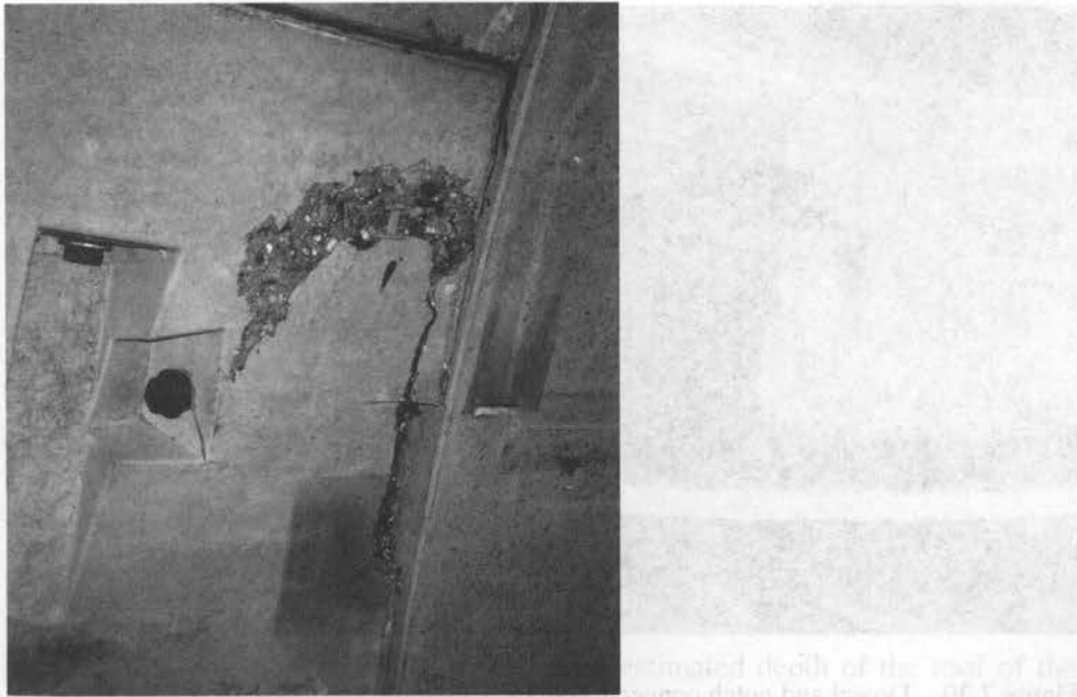
Figure 7.29 Damage to the tunnel lining; i.e. damage near the dowel and notch system
