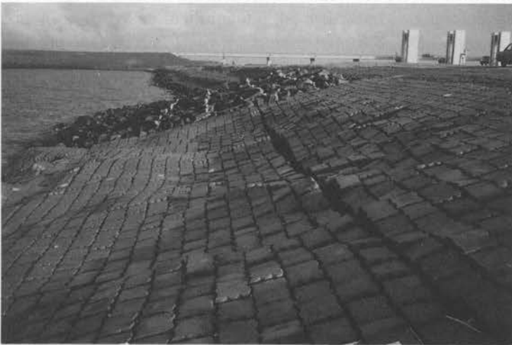
Figure 5.16 Damaged block mattresses at the test site near Lelystad at the IJsselmeer dike. Notice the fissure between the upper and the middle mattress, where the middle mattress has moved downward.
