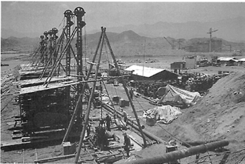
Building work in progress on the Three Gorges Dam on the Yangtze River in China
