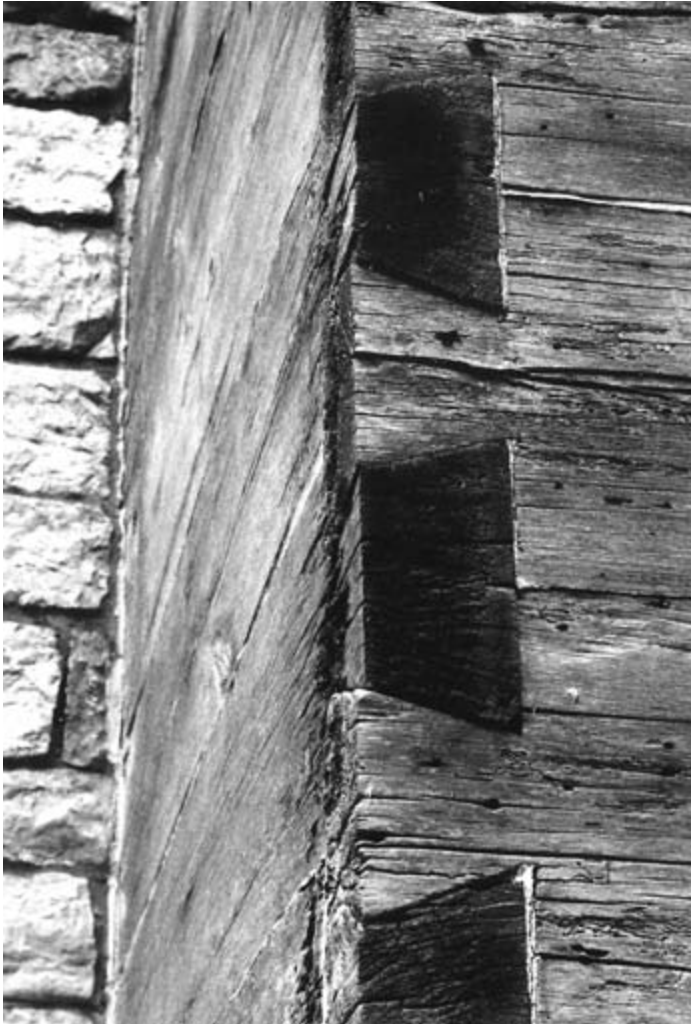
Full-dovetail notches have angled cuts on both the top and bottom while sides remain straight.
