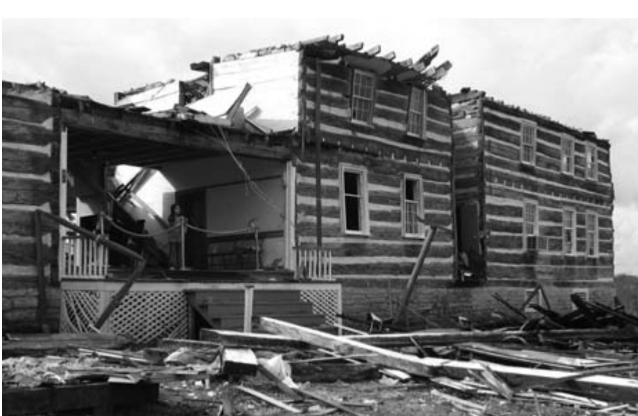
A 2008 tornado did terrible damage to Wynnewood, especially its upper floor. (Courtesy of the Tennessee Historical Commission.)
