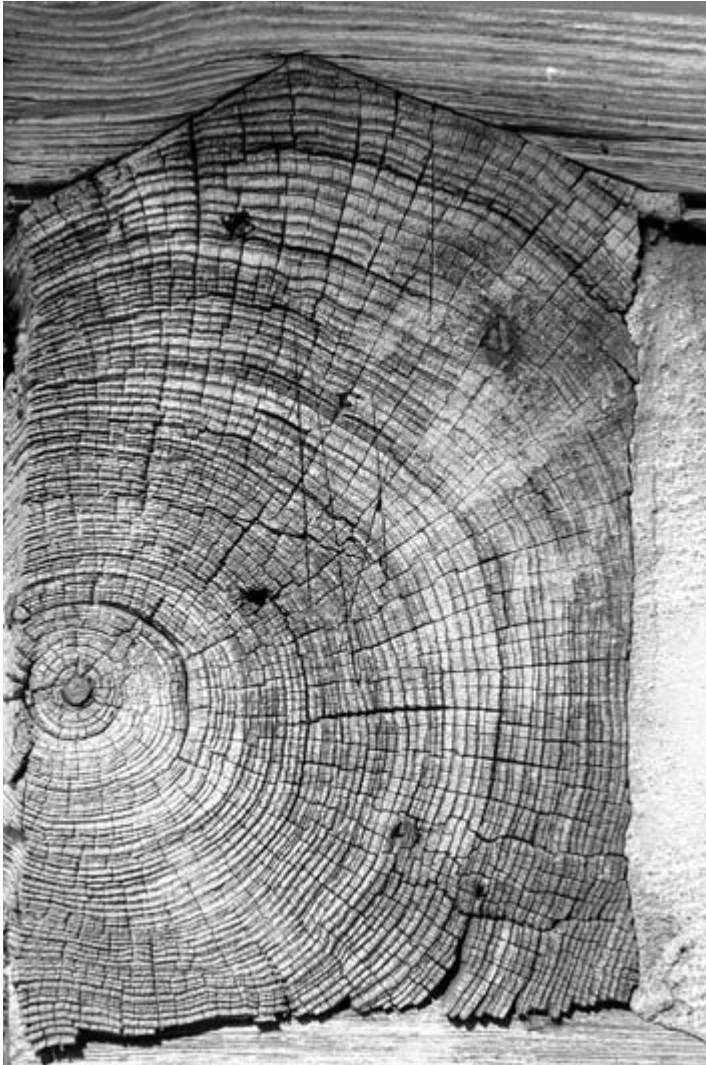
The V notch is an old notch type made on hewn squared logs.
