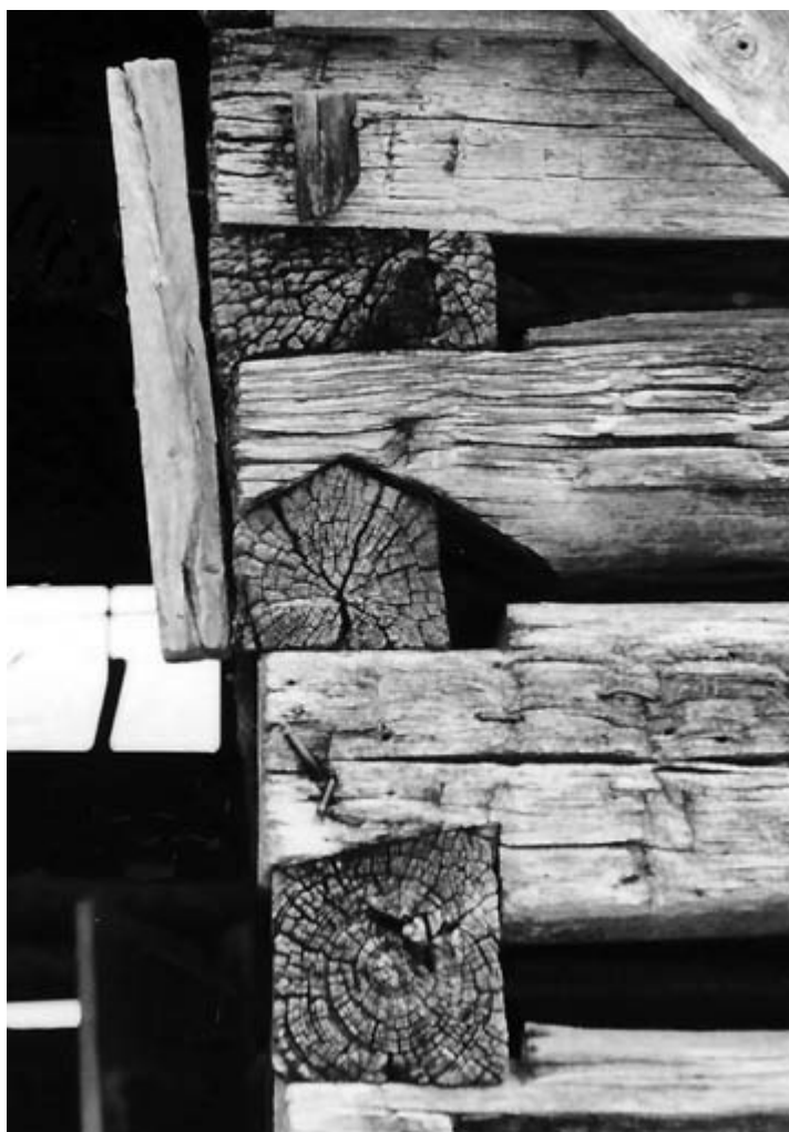
It is not unusual to find different notch types in the same building, as on this structure in Hancock County.
