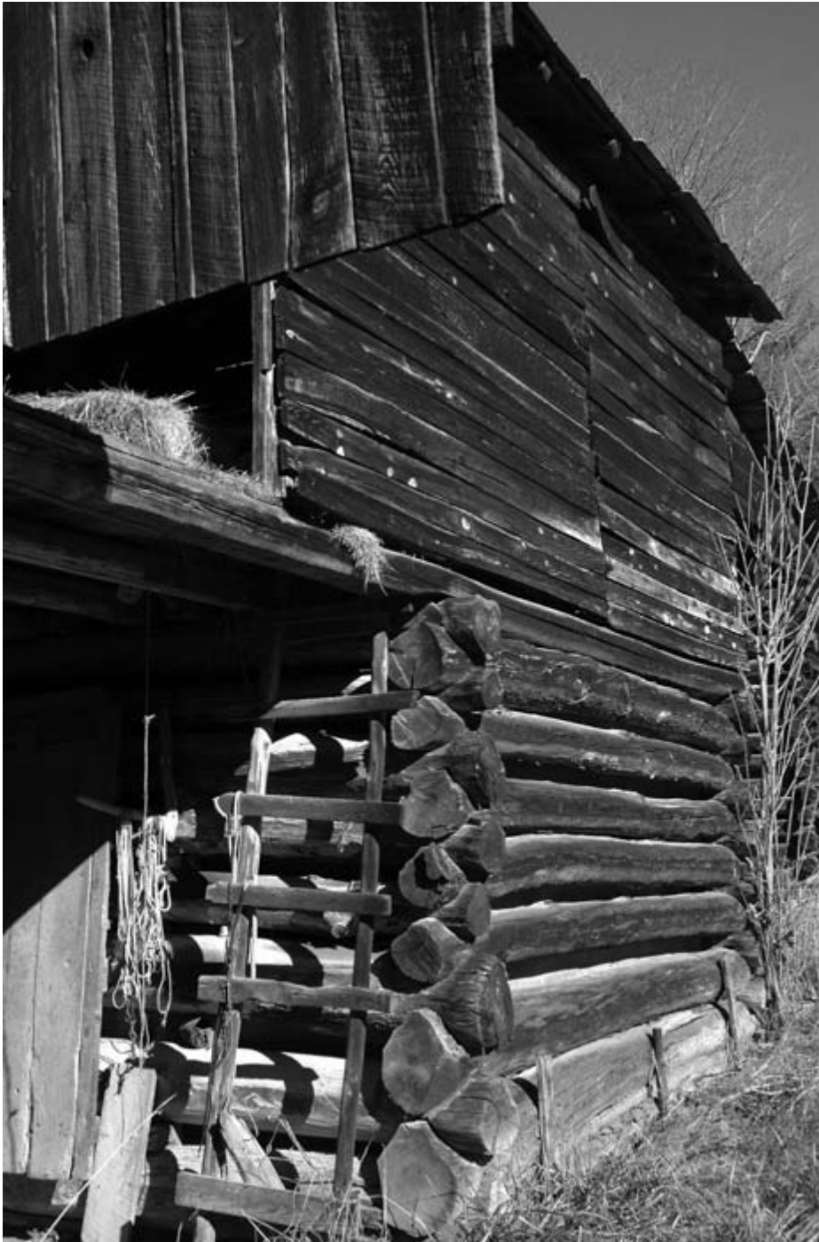
The large center crib in the Meek Williams barn was built with pine and oak logs with saddle-V notches.
