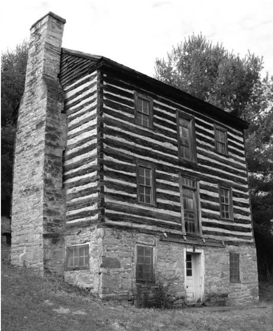
The Heinrich Ernst (c. 1784) house represents one of the oldest German-built log structures in Tennessee. Also called the Mauris-Earnest Fort house, it was built with V-notched oak logs and is located near Chuckey in Greene County.
