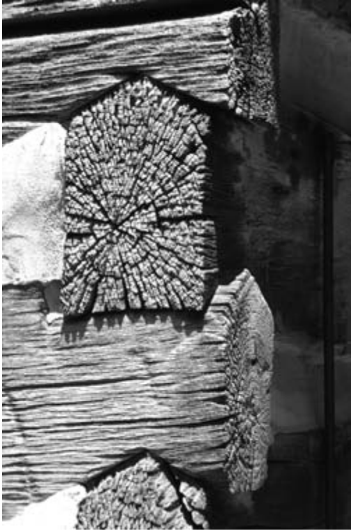
The logs at Wynnewood consist mostly of V-notched oak and black walnut logs.
