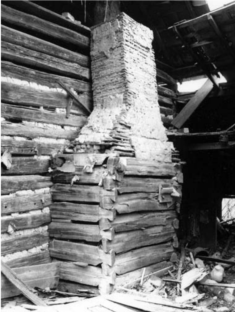
Authentic mud-and-stick chimneys, like this one in Hawkins County, are almost impossible to find because they either burned up during the early occupation of the structure or were soon replaced with limestone or brick chimneys. (Courtesy of the Tennessee Historical Commission.)
