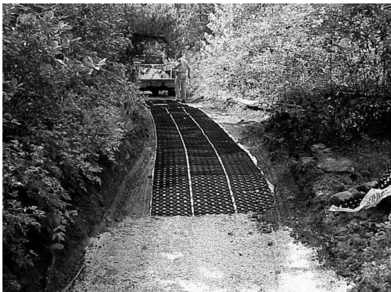
Fig. 13.5. Geosynthetics are applied on this trail in the Daniel Boone National Forest, USA, to improve trafficability for all-terrain vehicles and horses.
