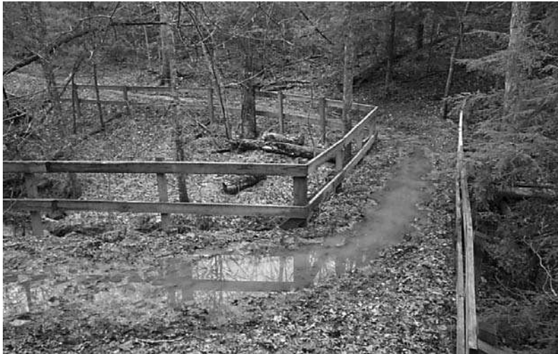
Fig. 5.15. Muddiness on a Big South Fork horse-trail bridge.
