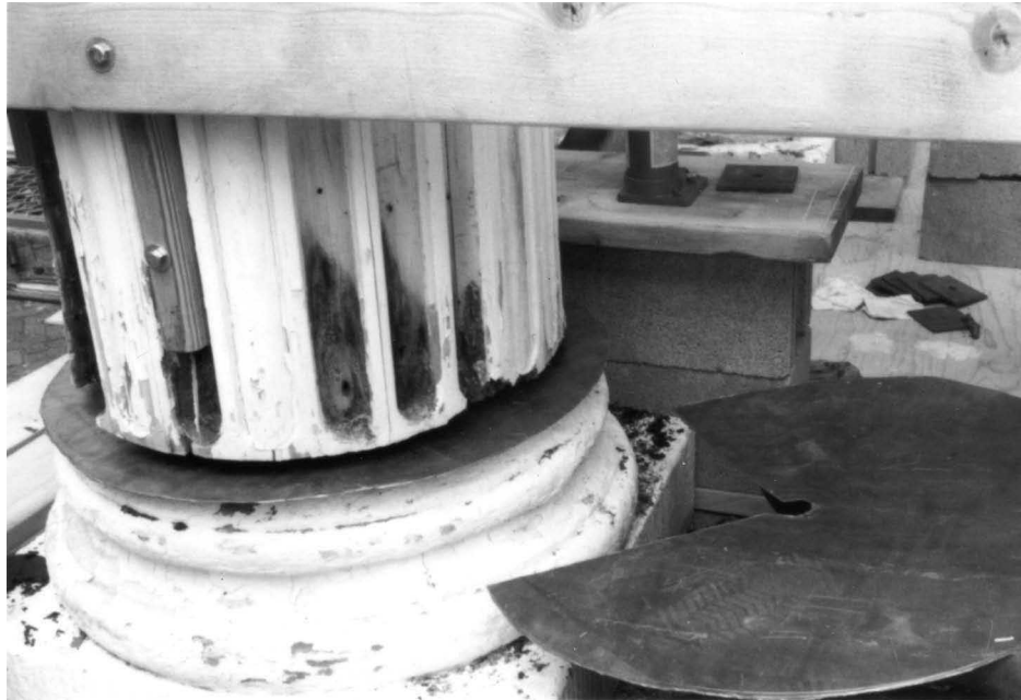
Fig. 6 —Ground moisture is often difficult to treat, particularly when it comes into contact with absorbent materials. In some cases, the insertion of a physical barrier may stop capillary action. This wooden replacement column on an entrance portico was showing decay (dark stains) after only 15 years. Moisture from the stone base was traveling up the wooden column. The insertion of a lead shield between the two materials will inhibit the rising damp and extend the life of the column. Photo: Bryan Blundell.
