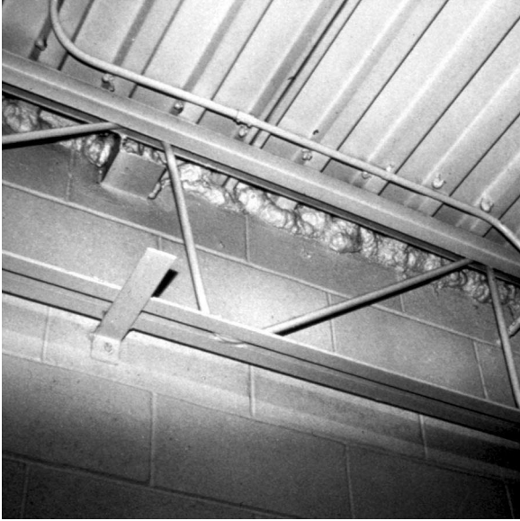
Fig. 16 —Spray foam used to seal the ends of a steel deck so it can serve as an air barrier. (Courtesy of Canam Building Envelope Specialists, Inc. and the Roof Consultants Institute.)
