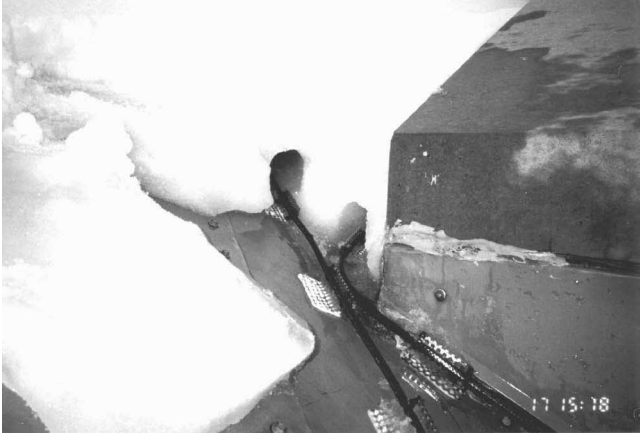
Fig. 47—Holes through an ice dam created by electrical heating cables.
