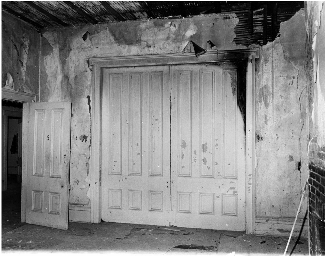
Fig. 17 —Moisture damage does not mean that all is lost. This decorative plaster ceiling in a circa 1900 Beaux Arts mansion was damaged when plumbing pipes under the roof froze and burst, but the ceiling was saved. After inspection both from below and using a fiberoptic boroscope inserted into the ceiling cavity, it was determined that most of the plaster keys holding the ceiling in place were sound and just needed to dry out. It takes about a month for every inch of damp plaster to fully dry and so the ceiling was left to dry for about a month. Next, with rubber mallet soundings, selective loose areas were reattached with epoxy adhesive injected through the plaster into the wood lath strips to create new keys. When dry, the ceiling was repainted and all the decorative elements were saved. Photo: NPS files.
