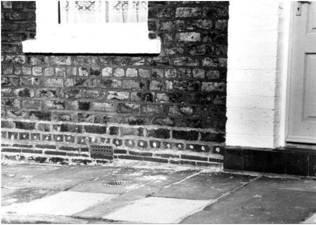
Fig. 7 —Not all methods of dealing with rising damp are successful. Chemicals injected through exterior masonry walls are popular in some countries, but should only be considered as a last resort as their long-term effectiveness is questionable and their poor appearance is visually damaging to historic buildings. Often redirecting bulk water with better guttering systems, subsurface waterproofing and footing drains, or the use of sump pumps, can effectively manage unwanted moisture. Photo: NPS files.
