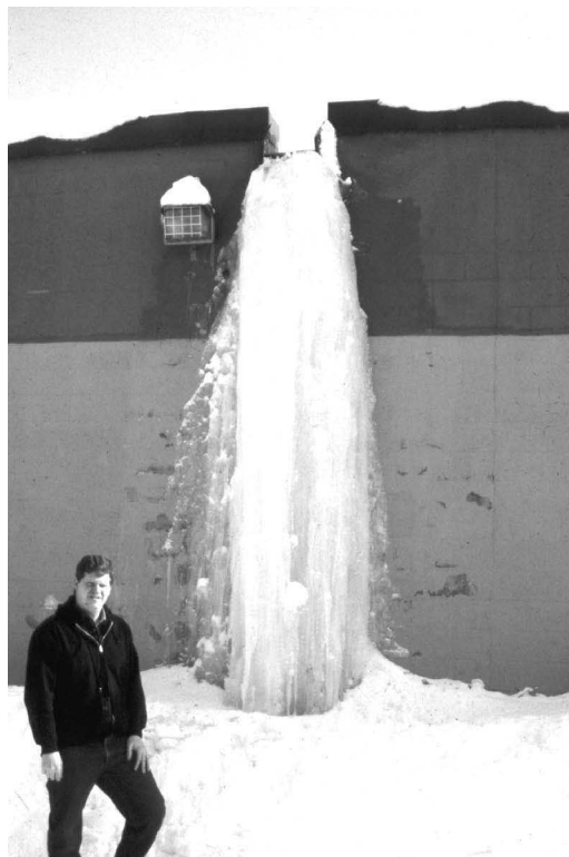
Fig. 3—Membrane roof with drainage through scuppers that have iced up.
