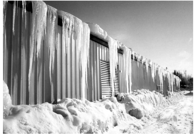
Fig. 29—Structural standing seam metal roof with severe icings along its eaves.
