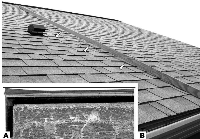
Fig. 10 —(a) Sag in the wood roof framing of a stone-wall house built in the 1850s (photo taken in 2005). Line above roof accentuates ridgeline sag. Roof framing was under-sized by modern standards. (b) Sag along the span of rafters in a house built in 1940 (photo taken in 2005). Reference stick touches the roof near peak and at eave. Arrowheads point to deflection of approximately 65 mm at mid span.
