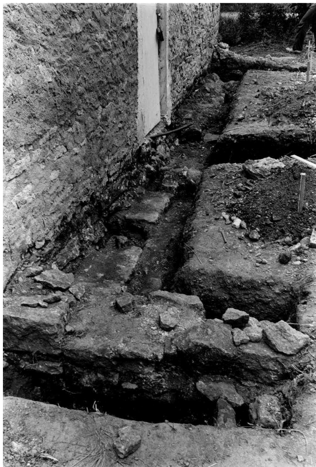
Fig. 5 —Archeological evidence may be found when regrading to alleviate poor site drainage, to install underground sewer pipes or to excavate for new footings. Care should be taken to identify and photographically record any evidence, such as lost site features, cisterns, wells, or early foundations, and to contact the State Historic Preservation Office to determine options for preserving this evidence. Photo: NPS files.
