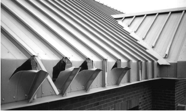
Fig. 50—The load of snow held on this metal roof by icings along its eaves peeled it apart.
