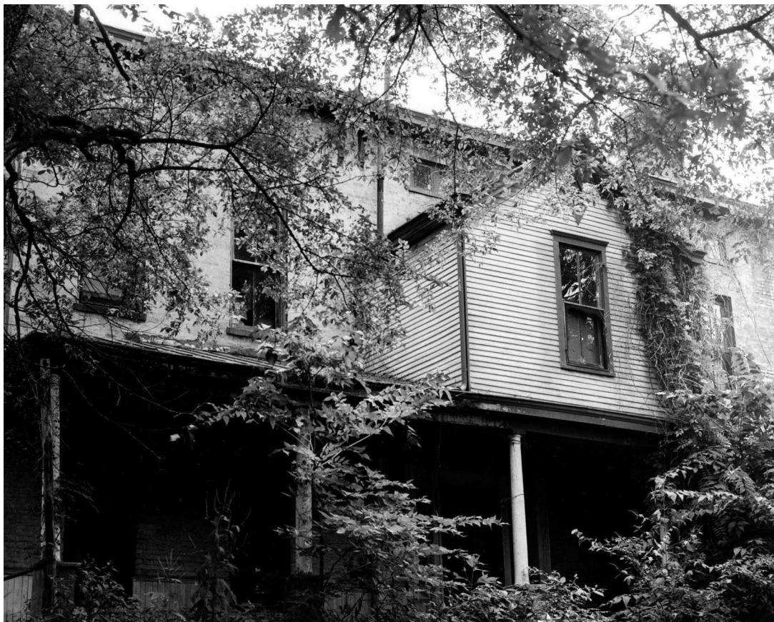
Fig. 4 —Deterioration is often most apparent on exterior surfaces exposed to contact with moisture, such as corners, foundations, or areas under and around gutters and downspouts. As part of preservation philosophy, only the damaged portions of the historic materials should be replaced in as close a match with the historic as possible. In this case, new cedar wooden shingles have been installed to replace moisture-damaged shingles and they will shortly be stained to match. It is not appropriate to replace available historic siding materials with nonmatching or synthetic siding as this would change the historic character of the property. Photo: NPS files.
