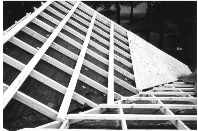
Fig. 37—Use of purlins to ventilate a valley. Without some form of cross-ventilation, valleys are not ventilated.
