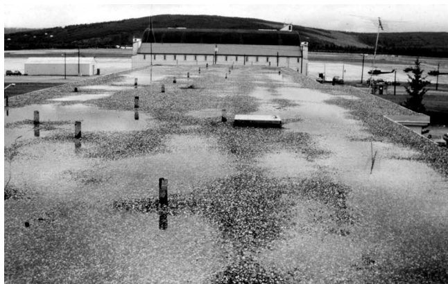
Fig. 2—Water remains on a “dead flat” membrane. Slope to drain is essential.
