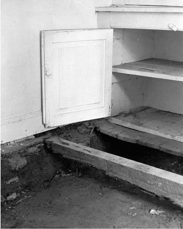
Fig. 14 —Fungal decay is a by-product of moisture damage in damp areas that can weaken structural elements. The removal of the flooring boards on this interior illustrates the loss of bearing capacity of the floor joist and that the dry rot, a type of fungus, has permeated the underside of the cupboard as well. The repair will fail unless the new joists are isolated from the damp foundation, preferably by deepening the crawl space and placing a slate or impervious element between the masonry wall and the joist. It is not advisable to install a poured concrete slab in the crawl space unless under-slab drains are installed to handle subsurface moisture as the build-up of ground moisture might cause a rising-damp condition in the wall. Photo: NPS files.
