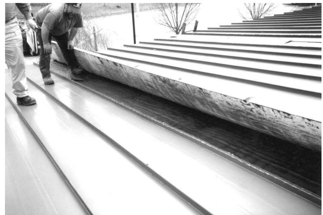
Fig. 8—Architectural metal panel lifted to show corrosion on its underside.
