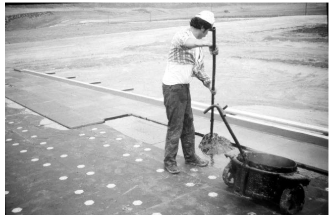
Fig. 25 —Using hot asphalt to adhere a layer of insulation to mechanically attached insulation below. (Courtesy of Dick Fricklas who advises that safety issues such as the unguarded perimeter and unprotected forearms are present.)
