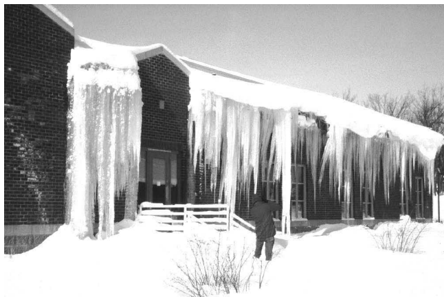
Fig. 1—Steeply sloped metal roof with severe icings along its eaves.
