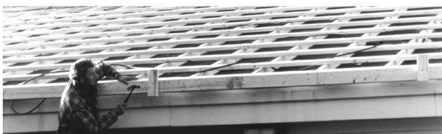
Fig. 36—Use of purlins to interconnect the ventilating airways of a framed roof.
