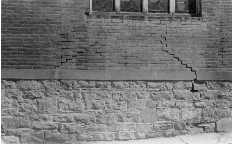
Fig. 9 —The preservation team should include a structural engineer familiar with historic construction. The settlement cracks in this masonry wall, seen as staggered along the brick and stone coursing, is indicative of a foundation failure. Instead of merely repointing the masonry, the underlying cause should be determined or settlement will likely return. Mortar analysis of the historic mortar, for both the brick and stone repointing, should be made so that each repointing mortar matches in composition, strength, color, and texture of the historic. Photo: NPS files.
