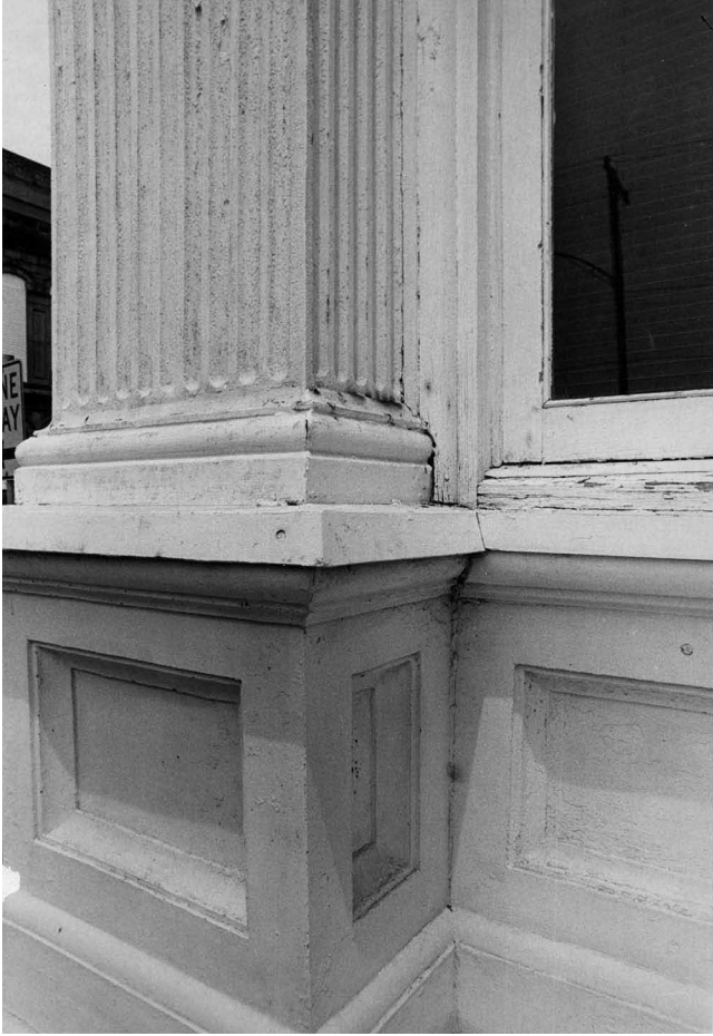
Fig. 12 —Window and door openings are vulnerable to moisture decay and must be maintained to protect aging materials. In this leaded window in a historic gymnasium, the wooden frame is rotting and must be reinforced. In this case, either a wooden patch or a synthetic compound with a binder and wood fiber can successfully fill the relatively small hole and be shaped to the correct profile. With prime and top-coats of paint, the patch should be stable for a long time. Photo: NPS files.
