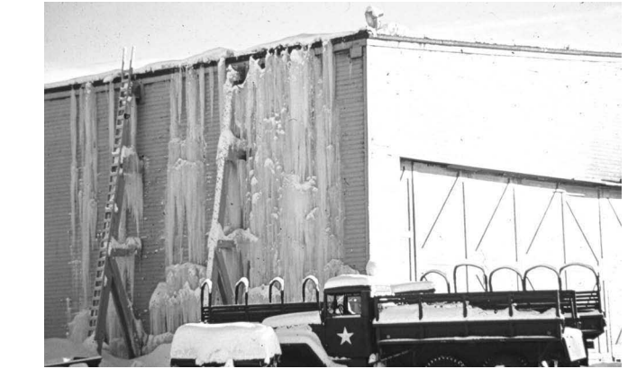
Fig. 40 —Icings can form on walls if the eaves do not overhang far enough.
