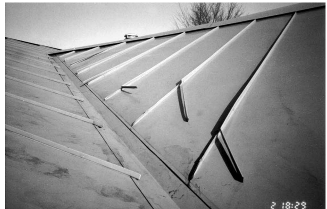
Fig. 49—Snow sliding down a valley does not move parallel to the standing seams of a metal roof but tends to bend them over and push them apart.
