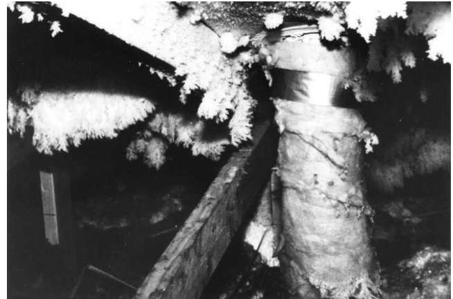
Fig. 32—Attic frost caused by leakage of indoor air by a ceiling with a vapor retarder but not an air barrier.
