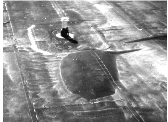
Fig. 27 —Breather vents do not prevent membrane blistering.
