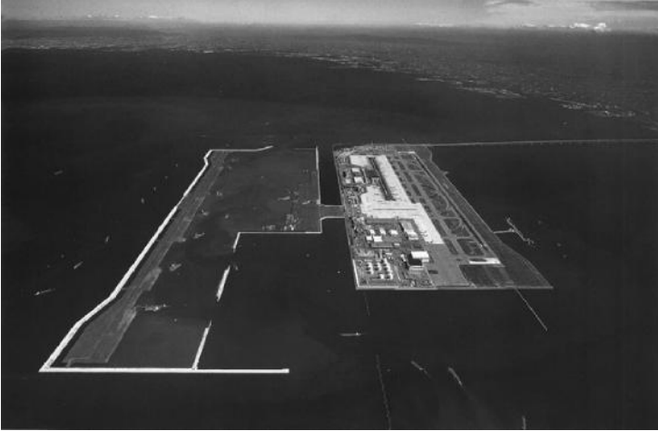
FIGURE 1.4 Kansai International Airport during Phase-II construction in 2002. (Photo courtesy by Kansai International Airport Land Development Co.)
