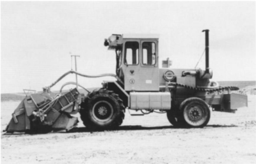
Figure 18.5 On-road stabilizing plant, Bathurst, New South Wales. This tractor is being used to cement-modify granular base to a depth of 150 mm during reconstruction of a rural highway. The shroud in front covers a rotating drum fitted with mixing picks; dry cement and water are fed in by different hoses in controlled quantities.
