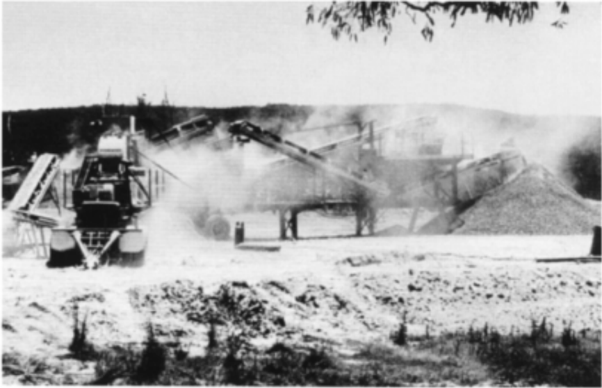
Figure 19.2 Dust nuisance at a temporary quarry site on a windy day, southeastern Queensland. Most of the dust is from open vibratory screens and conveyors rather than from the crusher. (Photo: R.A.Bathurst.)
