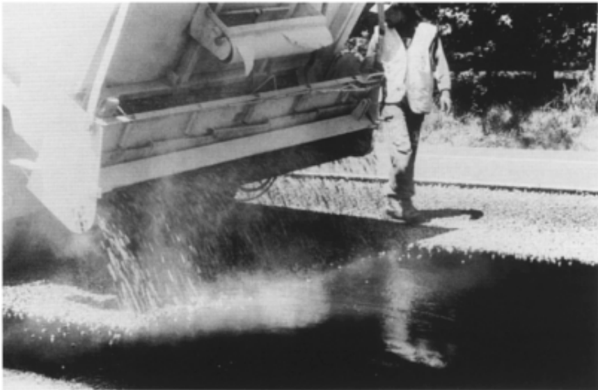
Figure 9.3 Spreading cover aggregate (chippings) on sprayed hot bitumen, Hamilton, New Zealand. The one-stone-thick layer was subsequently rolled before being re-opened to traffic.
