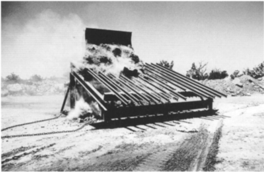
Figure 12.4 Rockfill being passed over a bar screen (‘grizzly’) to skim off oversize. The chains allow the grizzly to be towed a few metres as each pile of undersize is completed.
