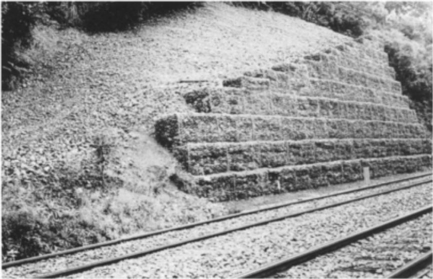
Figure 12.1 Three coarse rock materials together: railbed ballast (nominal 75 mm size), gabion stone (100 mm) and free-draining rubble (300 mm) behind the gabion retaining wall.
