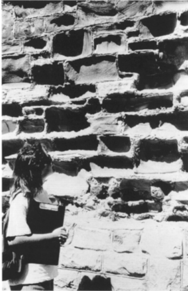
Figure 14.7 Varying degrees of sandstone decay close to the sea shore, Newcastle, New South Wales. This wall has been subject to salt crystallization and wind erosion. The upper courses are of typical Coal Measures lithic sandstone, while the lower courses are of stronger and much more resistant quartz sandstone.
