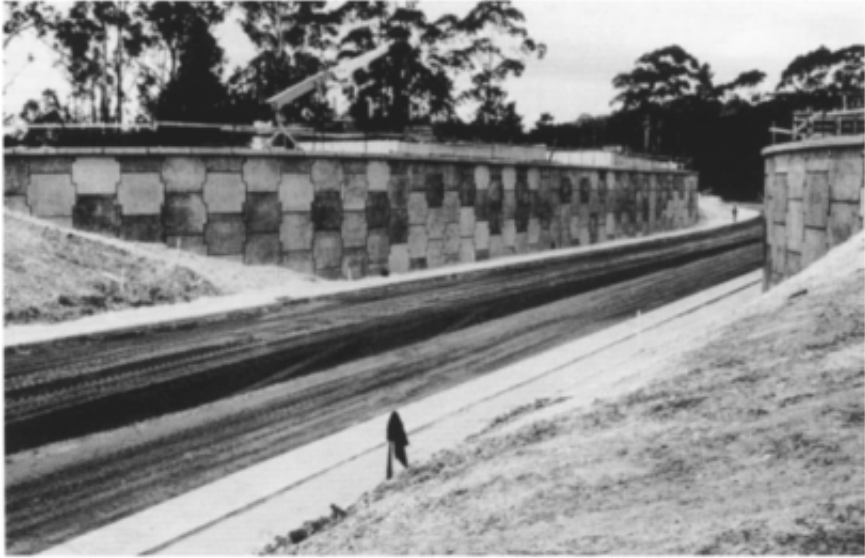
Figure 1.5 Reinforced earth bridge abutments and underpass beneath a freeway under construction at Ourimbah, New South Wales. The solidity of the abutments is deceptive: the cladding slabs are simply slotted together and held in place by steel tendons embedded in the dune sand backfill.
