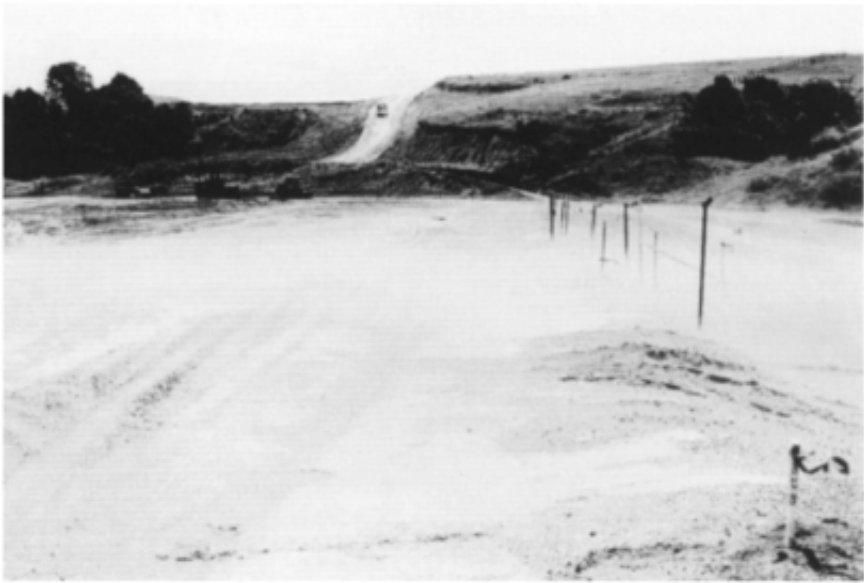
Figure 17.6 Lightweight bottom ash (FBA) fill on freeway construction site, Minmi, New South Wales. This 12 m high embankment overlies 20 m of soft estuarine mud. Note one hazard of silty fill materials—dust movement on a hot, windy day.
