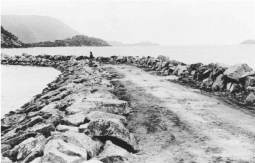
Figure 13.1 Typical rubble mound breakwater, near Cairns, Queensland. Note the attempt to lock together the primary armour blocks on the smooth leeward face. The top surface of the central core has been ‘blinded’ with crusher grit to allow vehicle movement.
