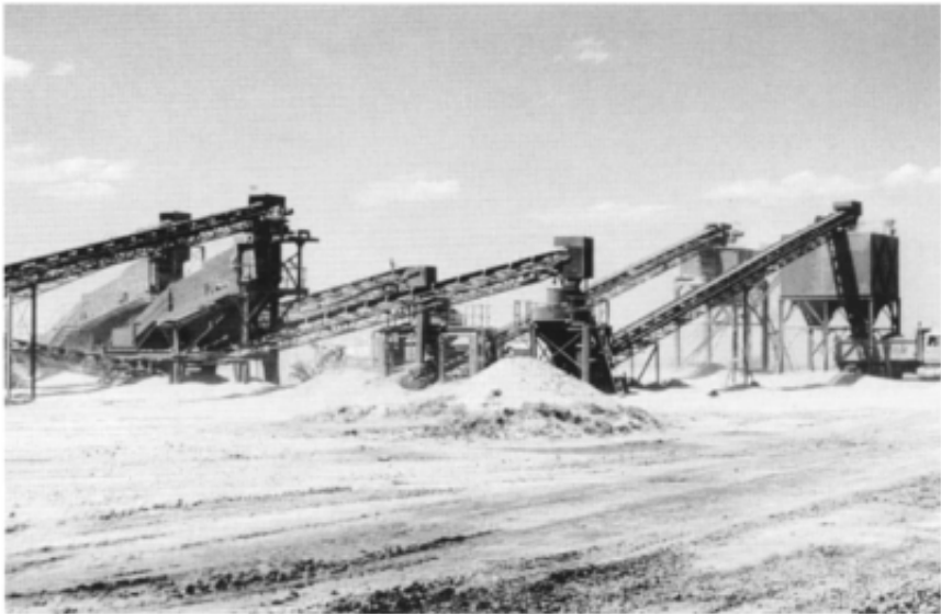
Figure 15.2 Mobile crushing and screening plant in operation north of Adelaide, South Australia. The complex arrangement of processing stages was necessary to obtain highway basecourse from sheet calcrete (‘paddock limestone’) of marginal quality, and incurred a high proportion of fines wastage. (Photo: G.Harvey.)
