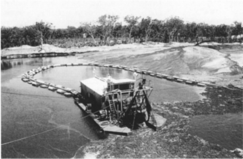
Figure 6.1 Suction-cutter barge working an offstream mineral sands deposit, Tomago, New South Wales. Note the lifting frame for manoeuvring the submerged suction pipe, the floating pipeline and the sand delta created by discharge from the treatment plant.
