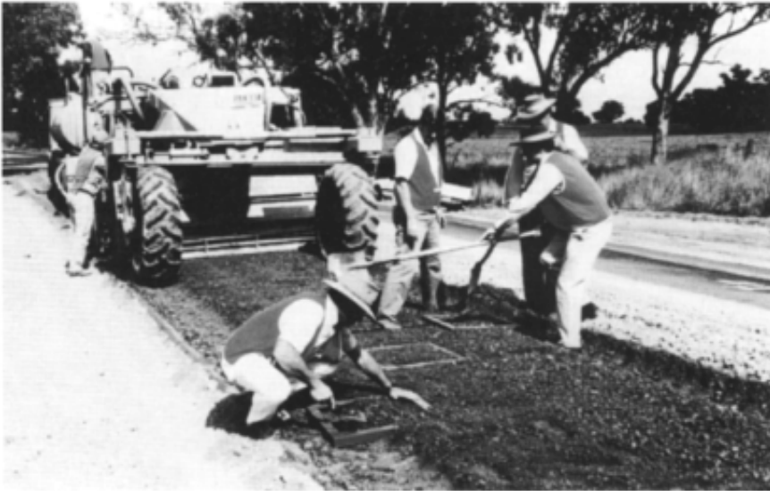
Figure 18.6 Measuring cement spreading uniformity during a deep-lift stabilization trial. The samples enclosed by the steel frames were subsequently tested for calcium content by their heat of neutralization. Note the purpose-built stabilizer at the rear, with its shrouded tine array behind the front wheels, and the adjacent highway lane still open to traffic. (Photo: I.R.Wilson.)
