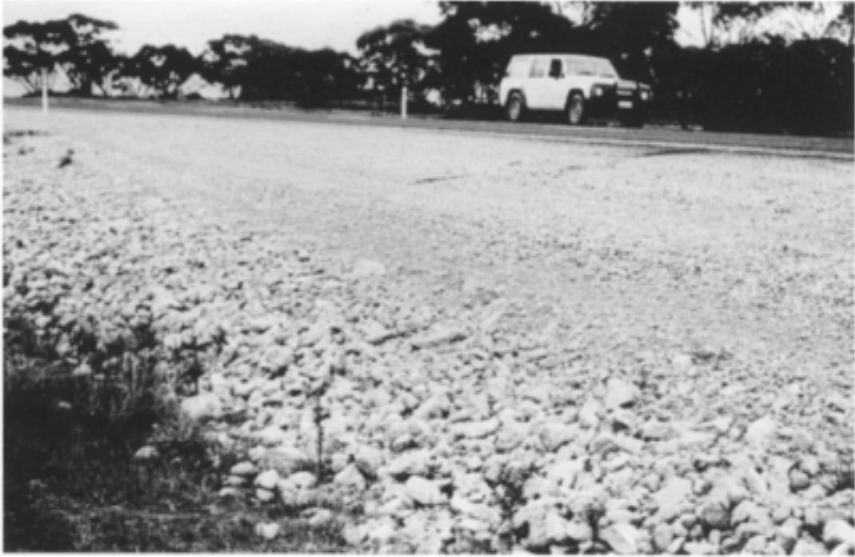
Figure 1.3 Calcrete pavement beneath a thin sprayed seal, Morgan, South Australia. This is typical of duricrust road gravels still used with minimal processing (in this case grid rolling, but elsewhere single-stage crushing) for secondary road pavements. The coarse fragments in the foreground have been moved to the edge of the road shoulder during construction, and the roadbase material beneath the seal is somewhat finer.
