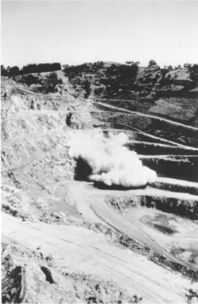
Figure 5.1 Bench blast, Riverview Quarry, Adelaide. Although this is a major quarry producing aggregates from dolomite and quartzite, a typical blast might include only 20 holes. (Photo: M.Drechsler.)
