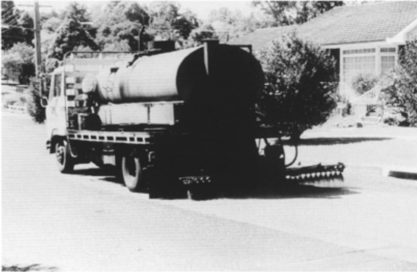
Figure 9.9 Spraying with cold bitumen emulsion to extend the life of an old chip seal by filling cracks, Turrumurra, New South Wales. In colour, the emulsion changes from light to dark brown then black in about 10 minutes, as it ‘breaks’.
