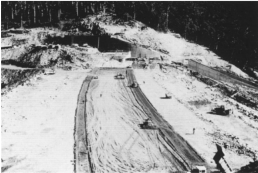
Figure 12.6 Corin Dam, near Canberra, Australia, an example of a 1960s central core rockfill dam. The darkest material is the filter zone between the core and the rockfill shell (light tones). Some of this rockfill was sulphide-bearing phyllite, which subsequently gave problems with acid leachate. (Photo: the late E.J.Best.)
