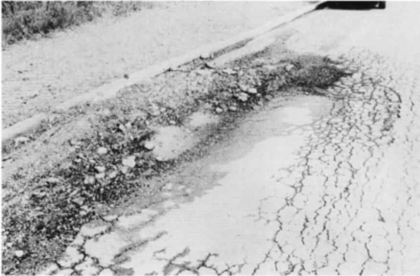
Figure 11.3 Pavement failure on a rural road near Wyong, New South Wales. The cause appears to be a combination of insufficient pavement thickness (about 120 mm of crushed sandstone) and a wet shale subgrade.
