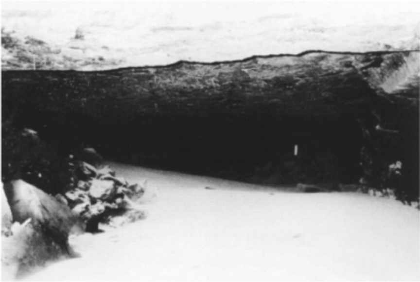
Figure 17.7 Pneumatically stowed dry fly ash in shallow abandoned colliery tunnel adjacent to a new highway cutting, Swansea, New South Wales. The void above this was subsequently filled with a wet grout containing 88% fly ash. (Photo: C.Francis.)
