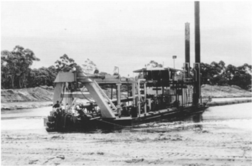
Figure 3.3 Bucketwheel dredger in littoral sands, Tomago, New South Wales. Note post-like 'spud' anchors and floating slurry pipeline at rear of barge.
