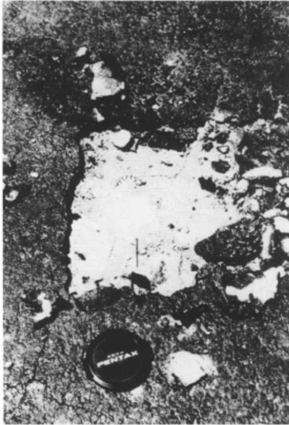
Figure 9.4 Debonded primerseal, near Broken Hill, New South Wales. The cutback bitumen has penetrated about 10mm into a calcrete gravel basecourse; seal detachment is probably due to salt in this material. (Photo: I.R.Wilson.)
