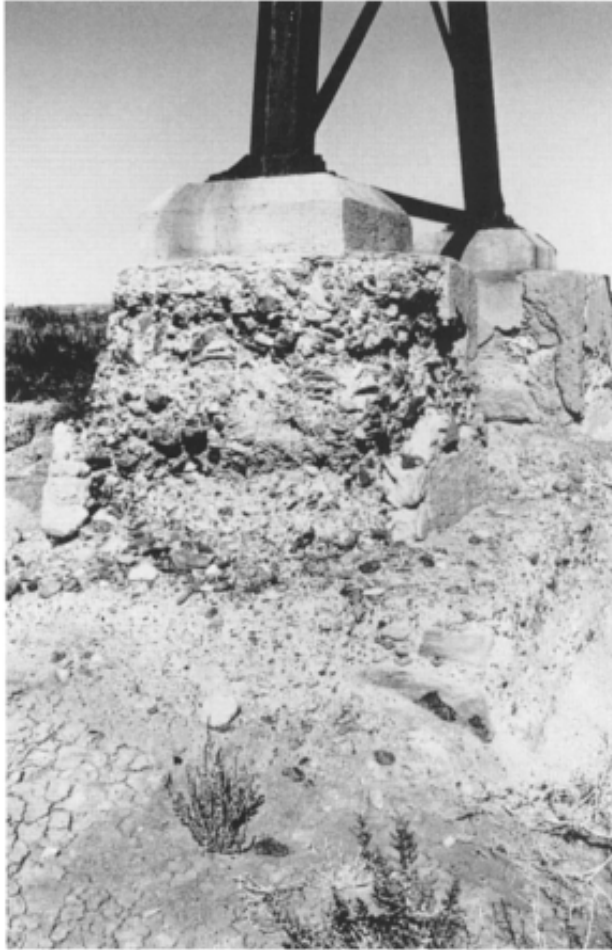
Figure 8.3 Concrete deterioration, Marree, South Australia. The primary cause of breakdown was probably dirty and gypsiferous aggregate, which was dug from the adjacent river bed in an arid area. However, silcrete pebbles predominate in the coarse aggregate and may have caused alkali-silica reaction (ASR).
