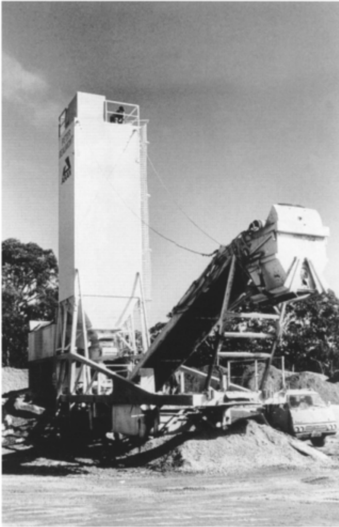
Figure 18.4 Mobile stabilizing pugmill installed at a temporary freeway quarry, Mittagong, New South Wales. The vertical bin contains cementitious stabilizer; crushed roadbase is fed into the hopper (left, behind bin), mixed by a pugmill beneath the bin and loaded into trucks by the elevating conveyor.
