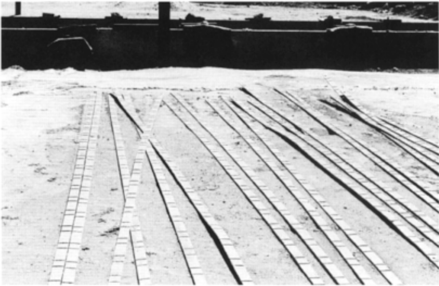
Figure 10.7 Reinforced earth tendons lying on compacted dune sand fill. Note the ribbing to increase friction between the tendons and the sand, and the cladding units at the rear.
