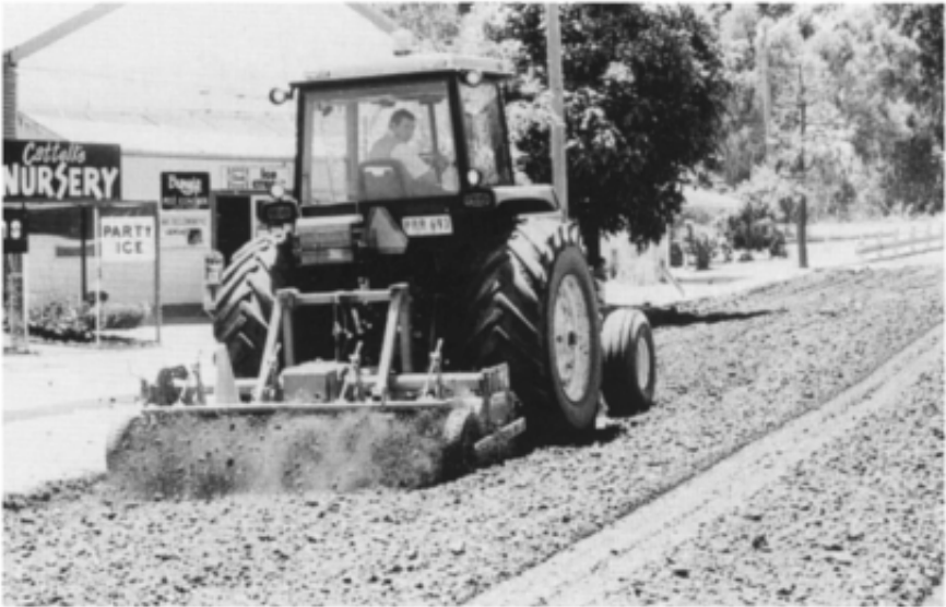
Figure 18.3 On-road granular stabilization, Darlington Point, New South Wales. An imported 30 mm crushed basalt is being blended into a well-graded but very silty alluvial sand of maximum size 5 mm from a local pit, in the proportion 1:4.
