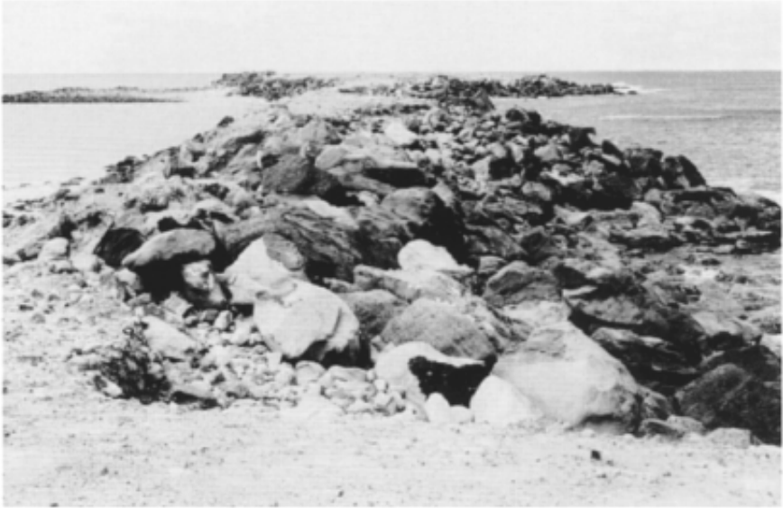
Figure 13.6 Damage to a 30-year-old disused breakwater near Newcastle, New South Wales. The rock used was randomly dumped weathered sandstone overburden from an open-cut mine (maximum block size about 5 tonnes).
