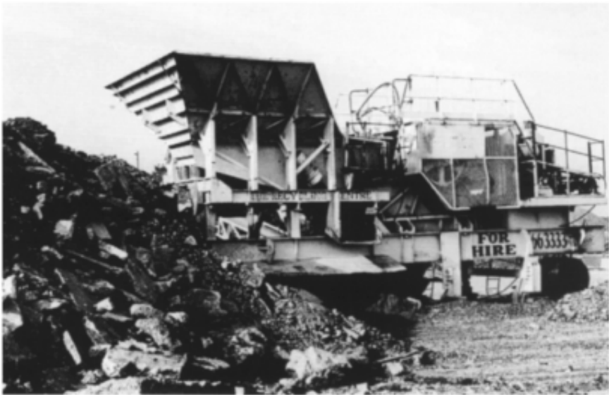
Figure 17.9 Mobile jaw crusher (note the flywheel) being used for reducing demolition rubble. The feedstock (left side) is a mixture of concrete slabs up to 0.63 m across, rock fragments and asphalt pavement chunks. A mobile impact crusher is used for secondary comminution to produce roadbase.
