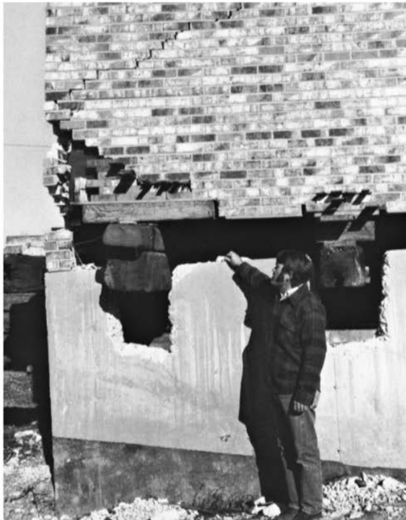
◀ FIGURE 10.19 Damage to a building by settlement. The house has been raised to its original elevation. The gap between the wall and the foundation shows the amount of settlement that has occurred. Source: Photo courtesy of USDA Soil Conservation Service.
