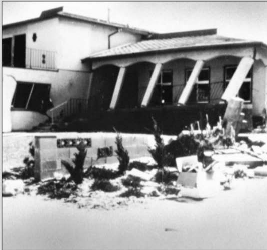
▲ FIGURE 8.80 Damage to two-story house near San Fernando. Source: Los Angeles Dept. of Building and Safety.
