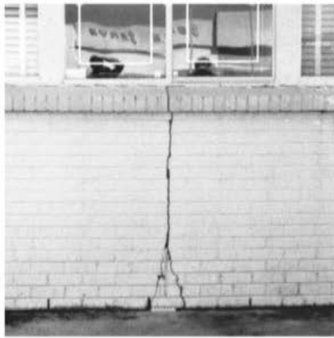
◀ FIGURE 10.31 Crack in a wall of an office building caused by swelling clays, San Antonio, Texas. The office building and adjacent shopping plaza were demolished because of structural damage by swelling soils. Source: Photo courtesy of the author.
