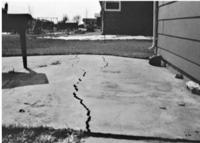
► FIGURE 16.43 Cracking of a cement slab by frost heave, Grand Forks, North Dakota. Notice the bulging of the slab in the vicinity of the crack. Source: Photo courtesy of the author.
