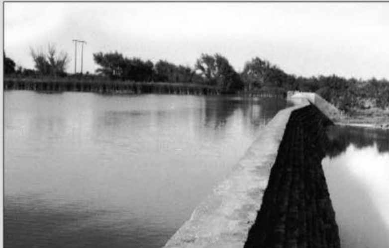
▲ FIGURE 9.35a Lake Ballinger Dam, Texas, before abandonment. Source: Photo courtesy of USDA Natural Resources Conservation Service.
