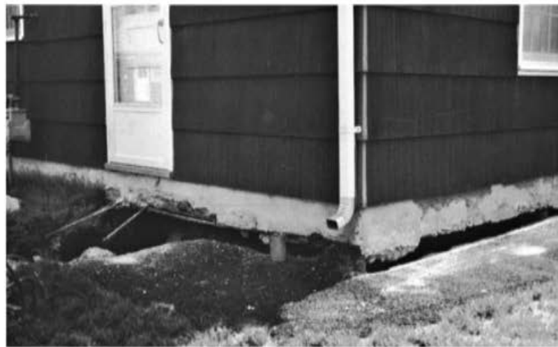
► FIGURE 10.44 Subsidence of peat and muck soils around a house built on pilings. The land surface around the house has subsided about 0.6 m in 2 years. The porch and steps have fallen off. Source: Photo courtesy of USDA Soil Conservation Service.
