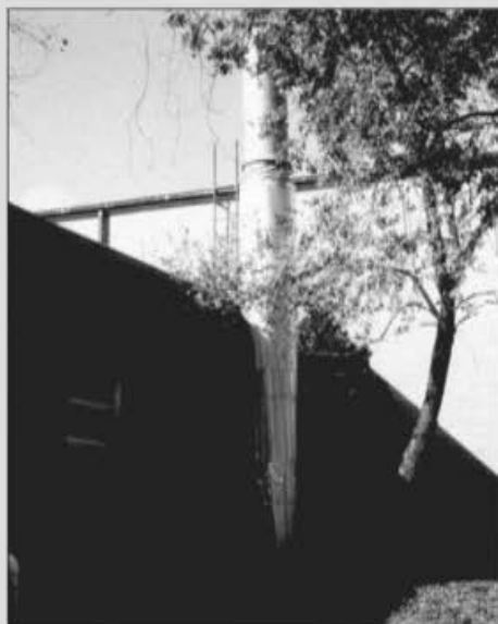
◀ FIGURE 12.38 Photo of hazardous fume ventilation pipe at elementary school in Bowling Green, Kentucky. Source: Photo courtesy of the author.
