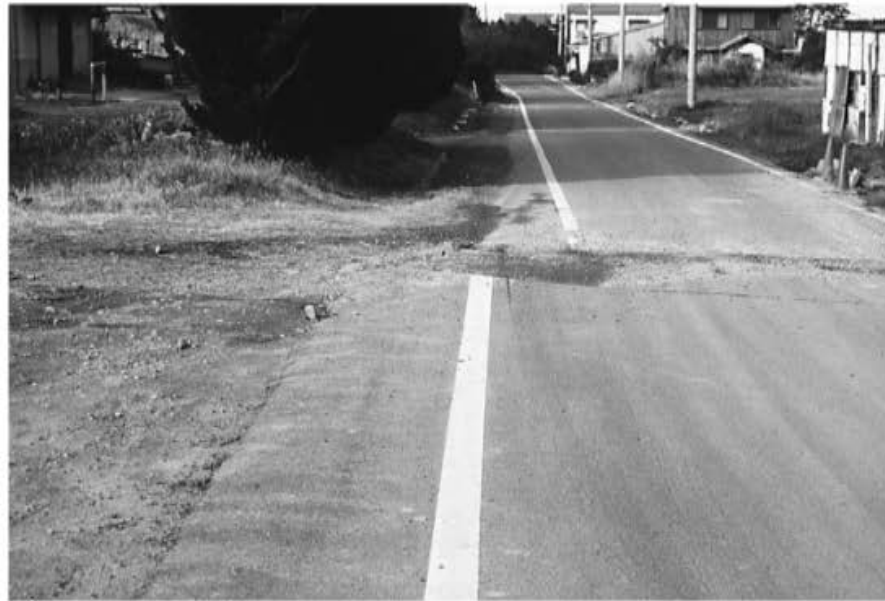
▲ FIGURE 8.25 Right-lateral displacement of 1.45 m can be measured by the offset of a paint strip along a road near Kobe, Japan. The rupture occurred during the 1995 Hanshin-Awaji (Kobe) earthquake. Source: Carol Prentice; photo courtesy of U.S. Geological Survey.
