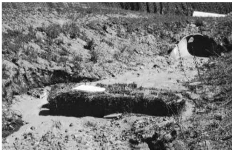
▲ FIGURE 9.32 Failure of a straw-bale filter designed to trap sediment in an unvegetated ditch along a newly constructed highway. Flow in the ditch overtopped the straw-bale dam and eroded a new channel adjacent to the straw bales. Source: Photo courtesy of the author.
