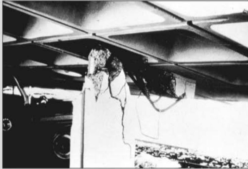
◀ FIGURE 8.79 Damaged column of re- inforced-concrete ambu- lance port at Olive View Hospital. Source: National Oceanic and Atmospheric Administration.
