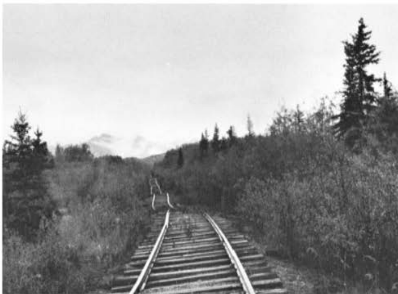
◀ FIGURE 16.49 Disruption of railroad resulting from permafrost thaw after removal of vegetation, near Valdez, Alaska. Source: O. J. Ferrans, Jr.; photo courtesy of U.S. Geological Survey.
