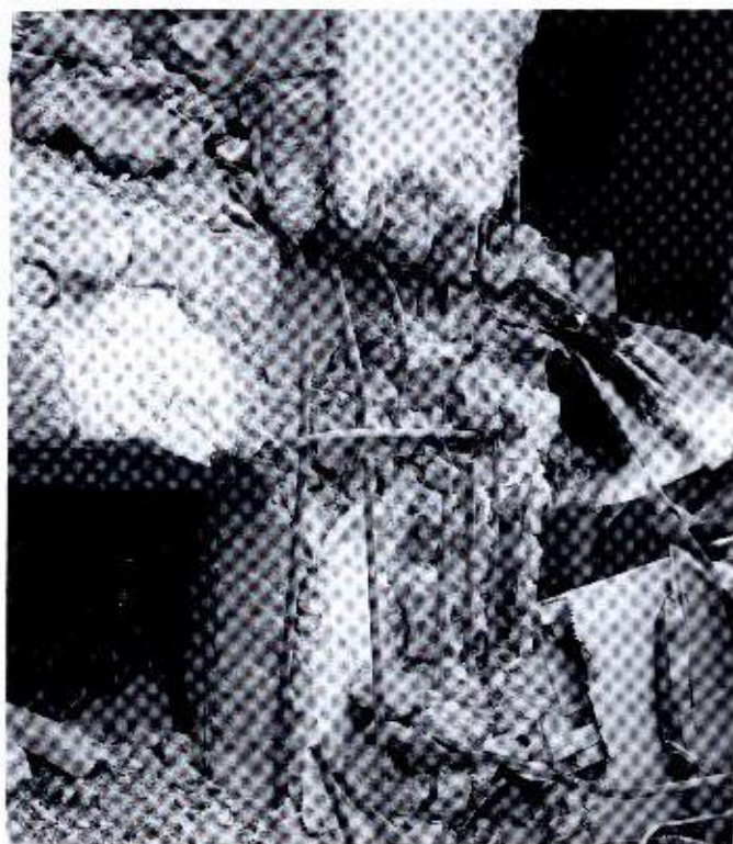
Plate 14. Failure due to insufficient ties, poor concrete quality and detailing of joints
