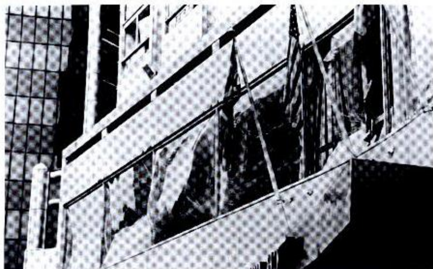
Plate 6. Europa Hotel, Belfast: laminated glazing panels are retained in robust frames despite large deflections. Photograph courtesy of Kirk McClure Morton
