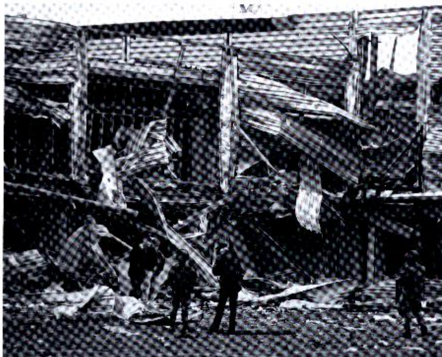
Plate 17. Severe damage to both the structure's steel frame and its lightweight metal cladding; Boucher Street, Belfast
