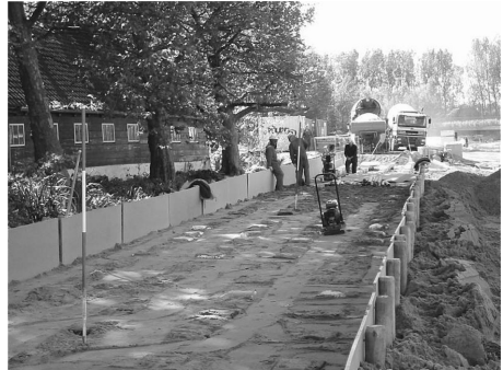
(f) Upon completion of the cap installation, sand is leveled between the caps to the top of cap level before placement of geogrid.
