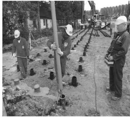
(d) The HDPE corrugated pipe is filled with grade 30 mortar and allowed 7 days for curing.
