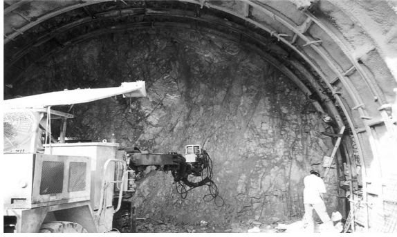
Figure 14.13. Heavy steel sets support for highly fractured/sheared granite, Sungai Selangor Dam diversion tunnel.
