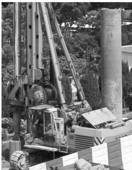
Figure 6.7. Photograph showing the steel casing in the background. In the foreground is the drill rig fitted with a cleaning bucket.
