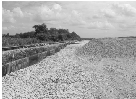
(h) Gravel bed is laid between two layers of geogrid before proceeding with layering suitable earth fill to form the final embankment profile.
