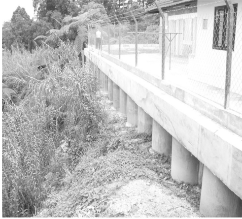
Figure 7.2. A completed caisson retaining wall complete with fencing installed at the top of the capping beam (photo courtesy of Kumpulan Ikram Sdn. Bhd.).
