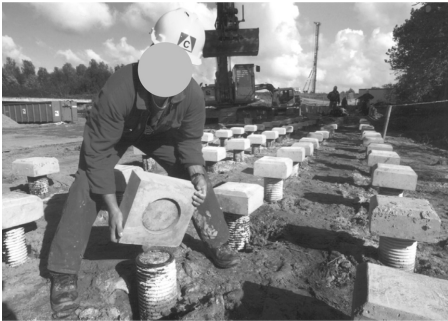
(e) The cured pile is capped with precast 300 \times 300 \times 150 mm thick grade 30 concrete cap.
