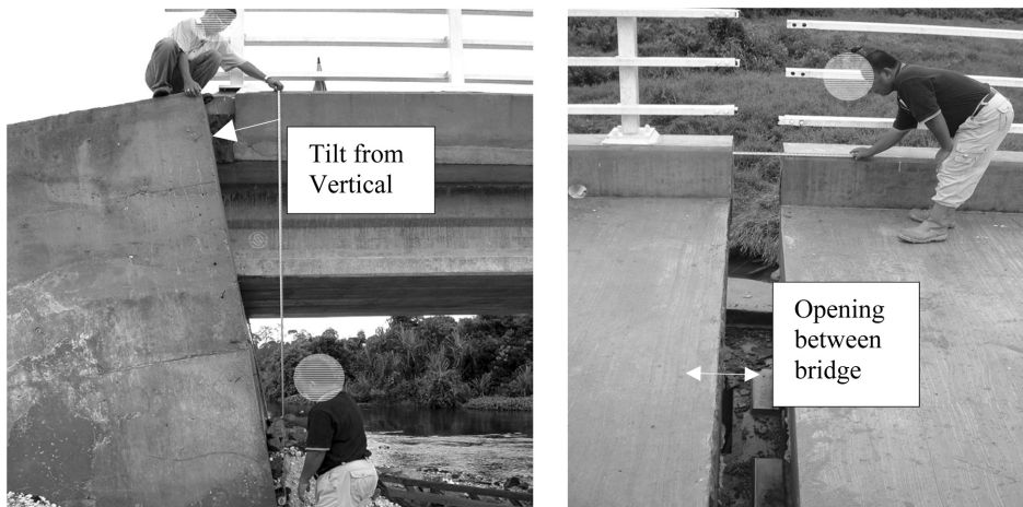
Figure 12.19. Tilted abutment and observed gap between bridge decks.
