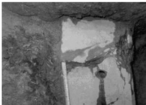
Figure 12.10. Pile C showing crushing of pile near pile cap.
