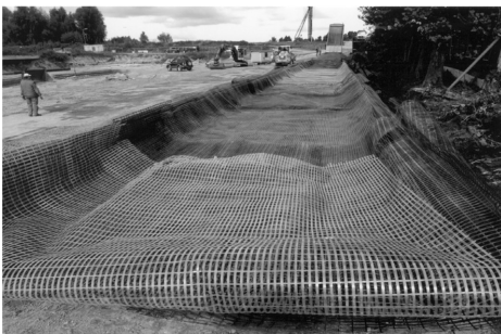
(g) Geogrid layer is placed over the sand bedding acting as the mediator to spread the embankment pressure/load onto the piles.
