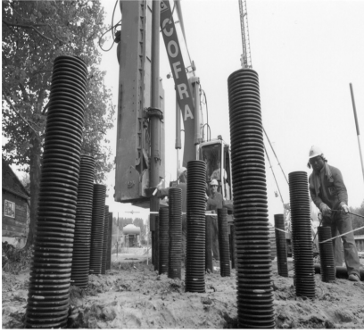
(c) Upon installation to the required pile spacing, the depth of pile is measured and reinforcement is lowered into the casing to the soffit of the pile.
