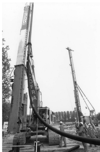
(b) The fabricated Corrugated HDPE casing is slid into the modified stitcher machine to push the pipe with the aid of a mandrel into the ground, up to two times the pile computed working load. The steel mandrel is then retracted leaving behind the corrugated pipe.
