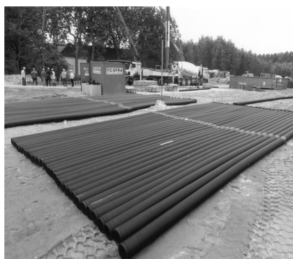
(a) Corrugated HDPE pipe is capped with 230 × 230 mm steel plate at bearing end and pushed into the soft ground with the aid of a 220 mm radius mandrel.
