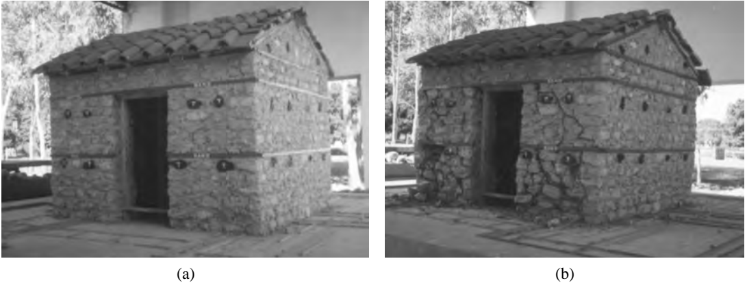
FIGURE 31.6 (a) Model 3 under shock test (b) Cracking below sill level at E-24.
