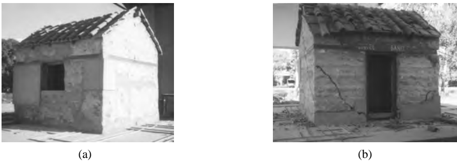
FIGURE 32.35 Behaviour of retrofitted model R1 (a) Model under shock test (b) Cracks pattern of Model R1.
