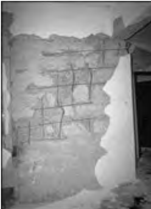
Diagonal tension-compression failure
