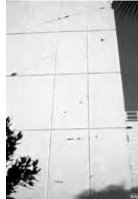
Flexure shear cracks
