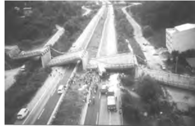
FIGURE 11.7 Failure of bridge spans due to inadequate seating length (after [2]).
