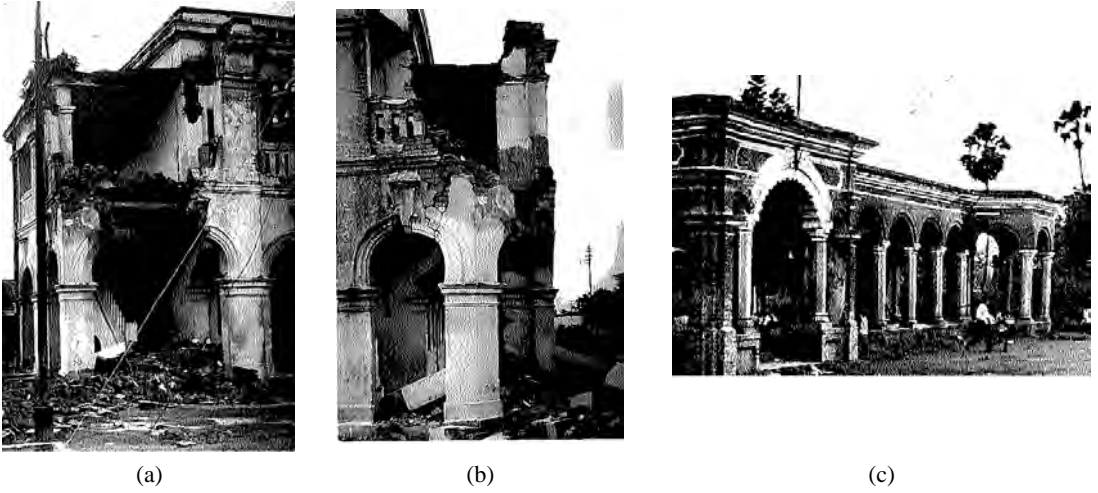
FIGURE 24.18 Typical features of damages (a) and (b) Out-of-plane failure of wall and arches (c) Failure of columns and roof.
