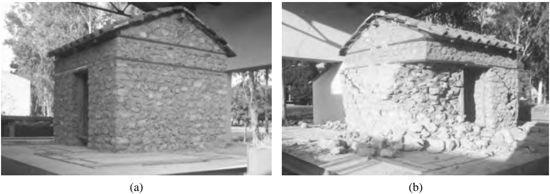
FIGURE 31.5 (a) Model 2 under shock test (b) Partial collapse below lintel band at shock E-23.
