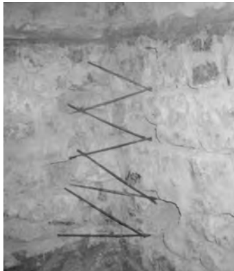
FIGURE 32.31 Stitching of damaged corner.
