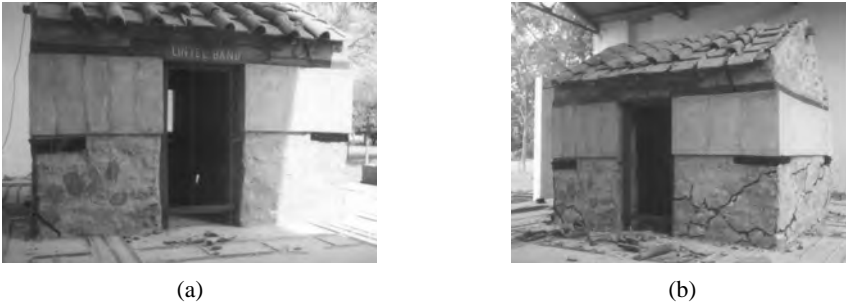
FIGURE 32.36 Behaviour of retrofitted model R2 (a) Model under shock test (b) Cracks pattern of model under shock W-21.
