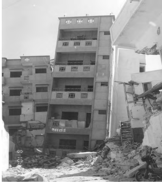
FIGURE 13.9 Anand building, Bhuj, damage resulting from pounding.
