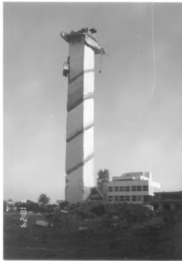
FIGURE 13.18 Undamaged lift core of a reinforced concrete building.
