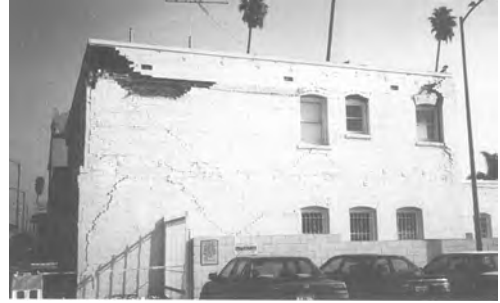
FIGURE 32.11 Weak mortar led to extensive shear cracking in the building (EERI, 1996).
