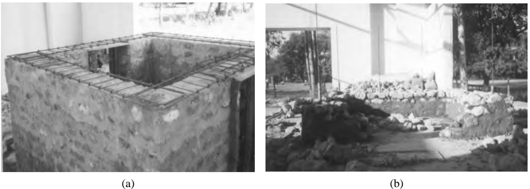
FIGURE 31.2 (a) Detail of horizontal band (main reinforcement: 2@12\phi mm, transverse reinforcement: 6\phi @ 150 mm) (b) Details of vertical and jamb steel (vertical reinforcement of diameter 12\phi mm, casing pipe of diameter 50 mm).
