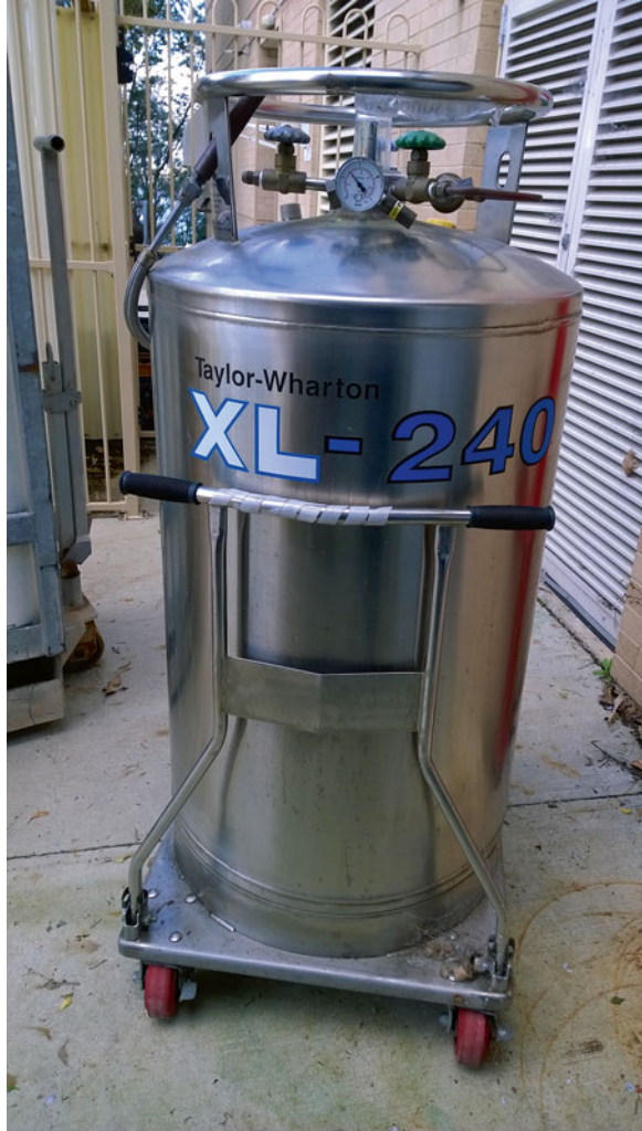
Fig. 8.2 Pressurised bulk liquid nitrogen tank
