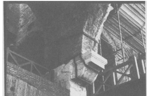
Figure 106. Detail of the support of the vault impost and of the previous reinforcement
