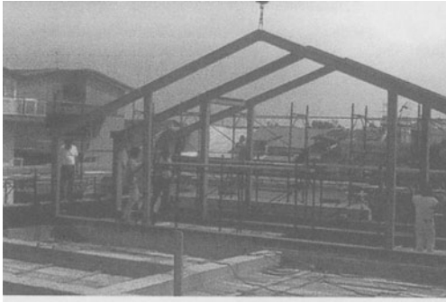
Figure 61. The new light structure for the roofing of a building in Succivo (Caserta, Italy)
