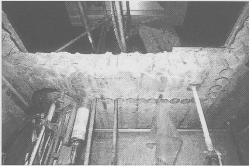
Photo 7. Drilling of an opening in a concrete floor, with a diamond core (Courtesy Zschokke)
