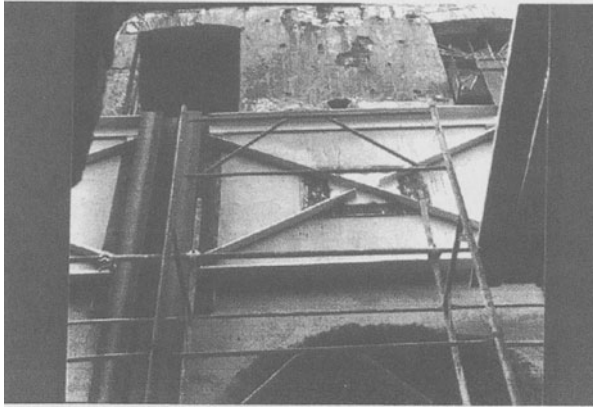
Figure 66. Steel braces on the masonry wall of the Montemarano church (Avellino, Italy)
