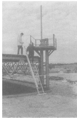
Figure 20. The lifting system of the hall roof after the placement of the first roof section to its new position.
