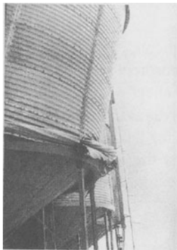
Figure 16. Failed silo with corrugated sheet.
