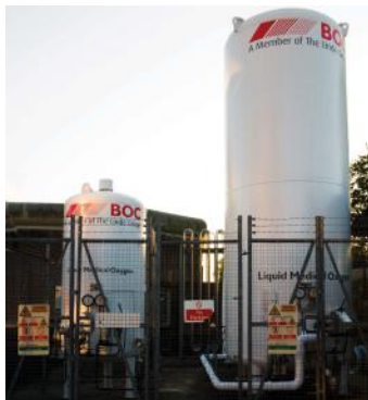
Fig. 1.1.1: The main and backup vacuum insulated evaporators outside a hospital.
