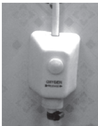
Fig. 1.1: Wall mounted outlet of the central oxygen pipeline
