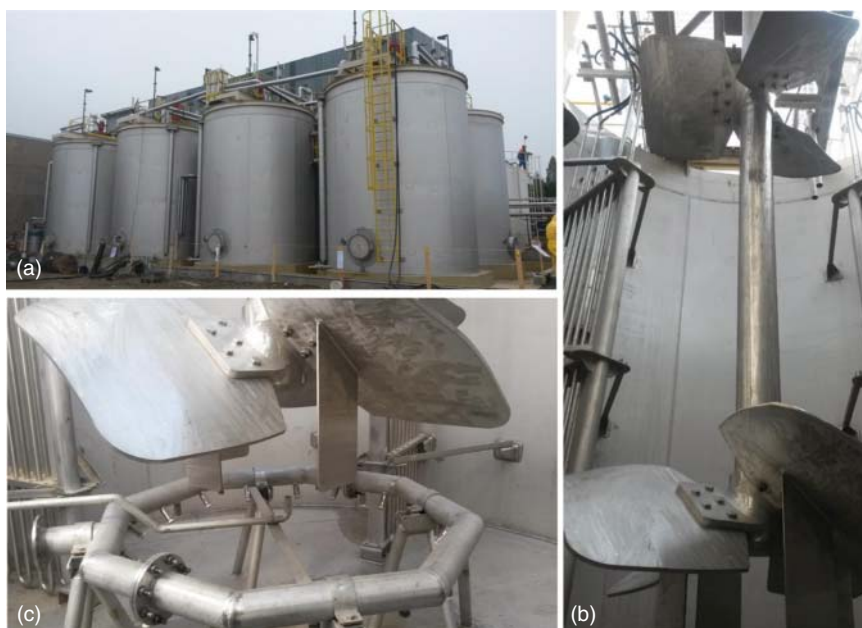
Figure 13.7 Mondo Minerals bioleach plant in Vuonos, Finland. (a) Concentrate is fed into four primary tanks operating in parallel. The secondary oxidation stage comprises another four tanks in series, which provide sufficient residence time for the target level of biologically catalyzed sulfide oxidation and sufficient reactor units to minimize short circuiting of the slurry; detail views on the stirred-tank impeller, cooling baffles (b) and the aeration ring (c). With permission from Neale et al. (2016).
