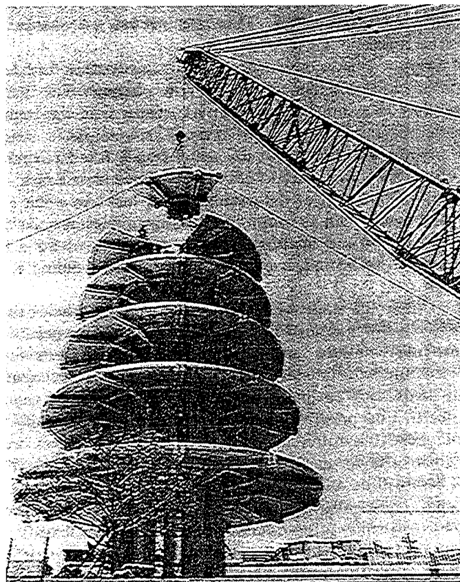
Fig. 1-29. Precast Pagoda Japanese Center, San Francisco, California, wound with circular posttensioning (T. Y. Lin International, Consulting Engineers).
