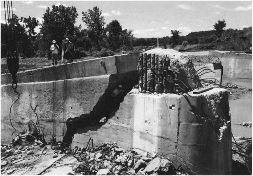
Figure 8-10. Schoharie Creek Bridge failed plinth. Courtesy Howard F. Greenspan.
