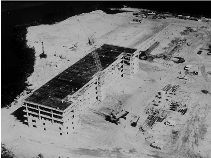
Figure 5-7. Harbour Cay Condominium before the collapse.
