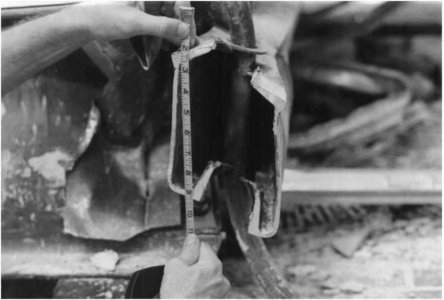
Figure 2-5. Failed fourth-floor beam. Courtesy Lee Lowery, Texas A&M University.
