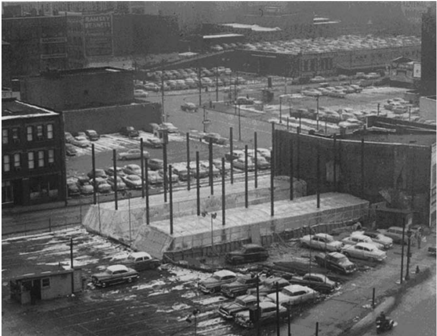
Figure 4-16. Cleveland parking garage under construction. Courtesy Cleveland Press Collection, Cleveland State University Library.
