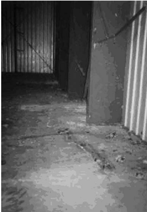
Figure 4-3. Damage to concrete foundation.
