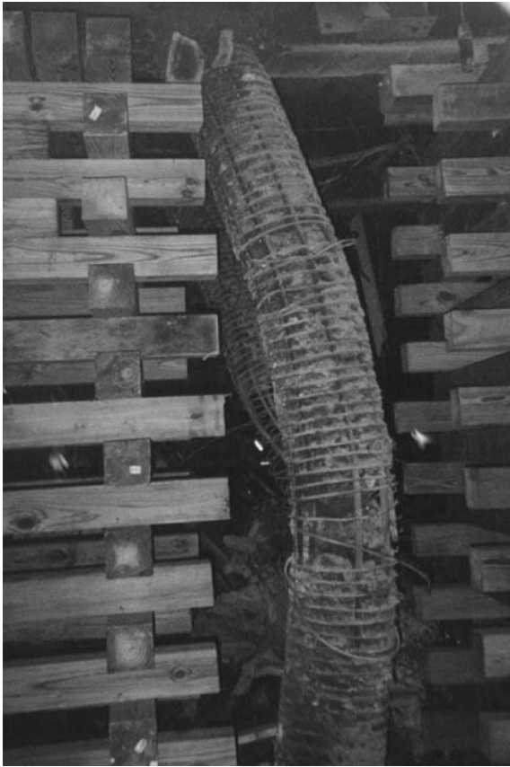
Figure 5-14. Damage to a spiral column.
