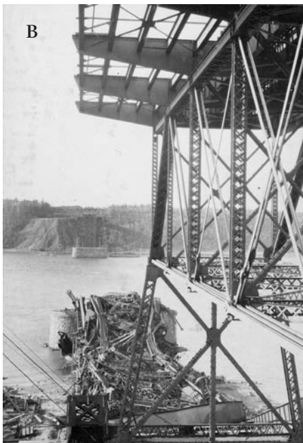
Figure 3-2a, b. The collapsed Quebec Bridge. Courtesy Archives Canada.
