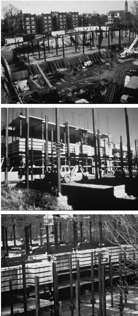
Figure 4-9. L'Ambiance Plaza Lift Slab Construction. Courtesy National Institute of Standards and Technology.
