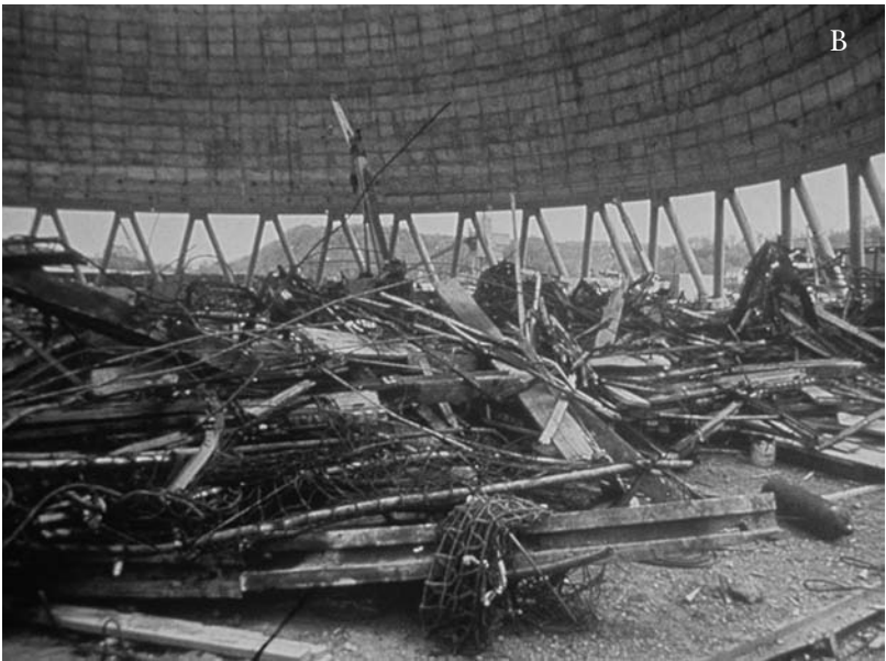
Figure 9-9a, b. Willow Island Cooling Tower collapse. Courtesy National Bureau of Standards/National Institute of Standards and Technology.
