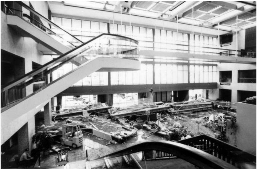
Figure 2-3. Scene of the Kansas City Hyatt Regency collapse. Photo provided by Wiss, Janney, Elstner Associates, Inc. (WJE).
