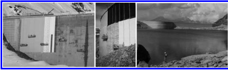
Figures 1, 2 and 3. At left Silvretta dam: from right to left control of surface, installation of vertical profiles, of support geogrid, of anti-puncture geotextile, of PVC geocomposite, and sheltered scaffolding at left abutment. At middle and right Illsee dam: exposed PVC geocomposite installed on an anti-puncture geotextile (white material) on rock masonry, and on a geonet (black material) on concrete.
