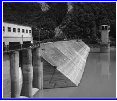
Photo 1. Concrete facing after the earthquake.
