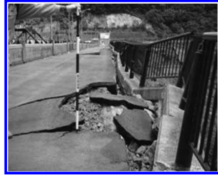
Photo 2. Deformation at the dam crest.
