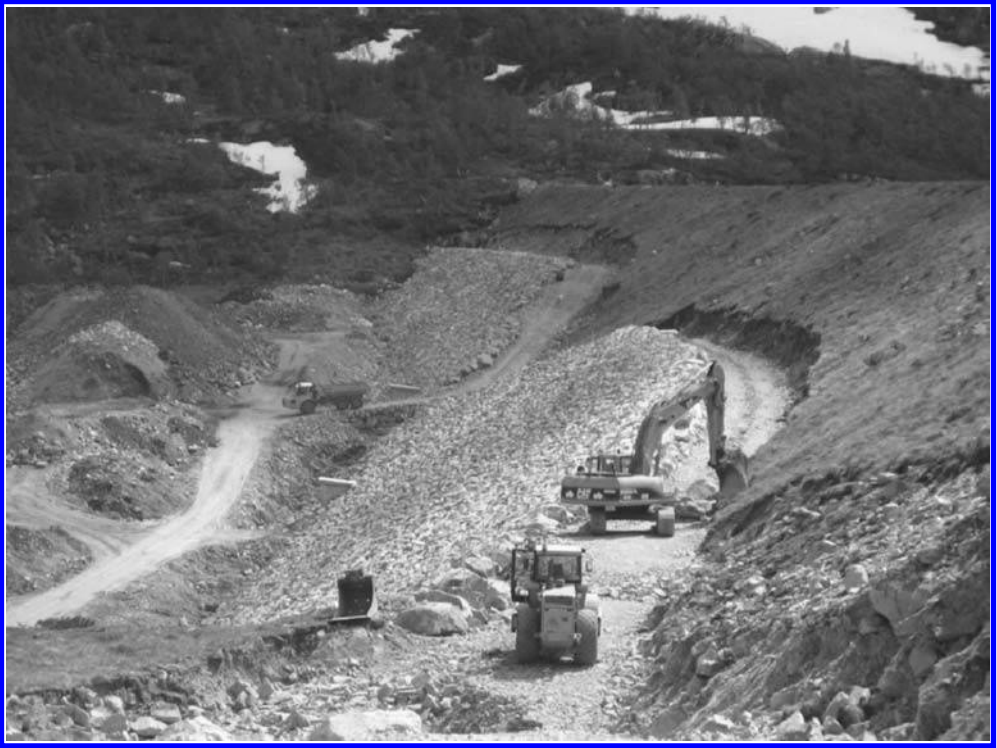
Figure 2. Excavation of vegetation and soil masses and establishing new rip rap structure. (Photo: Pedersen).
