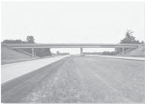
These bridge girders are statically indeterminate since they are continuous over their piers.
